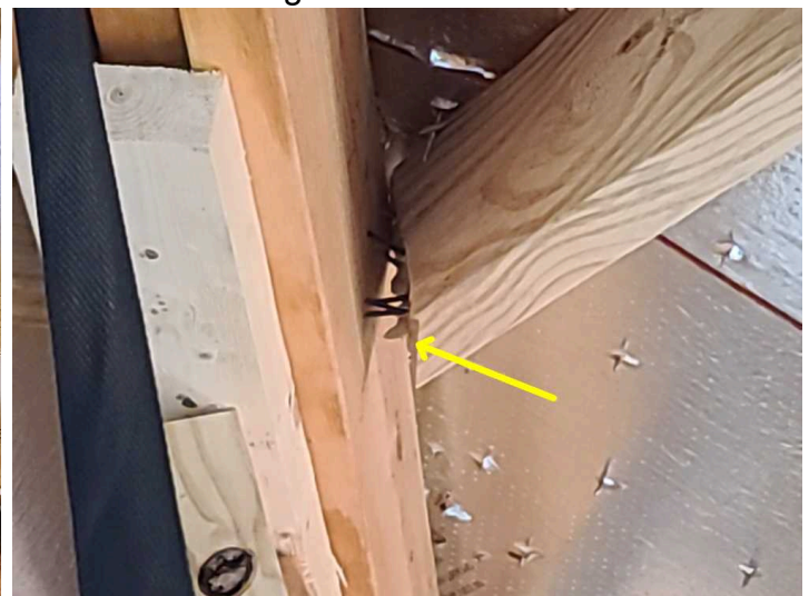
Ends of rafters were observed to be not cut flush with corresponding components; Area that needs repair is above attic access.
