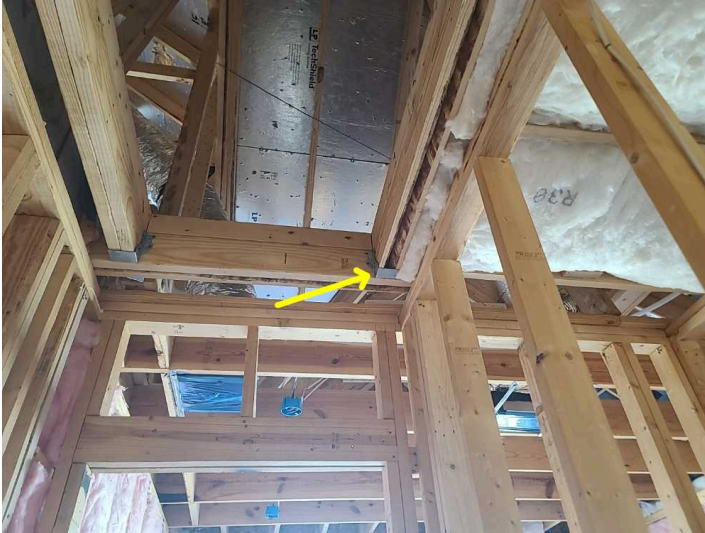
Joist hanger missing nails/ fasteners at the attic access.
