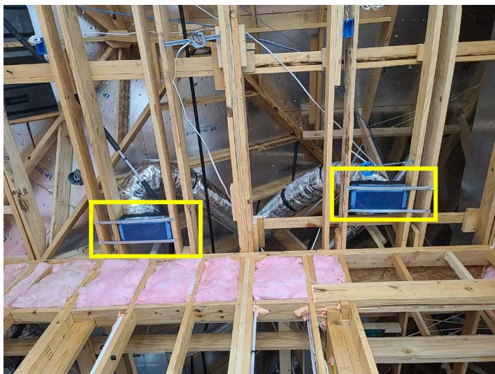
HVAC supply register boxes are not square with each other due to framing changes. Recommend reinstalling before sheetrock; bonus/ flex room ceiling.
