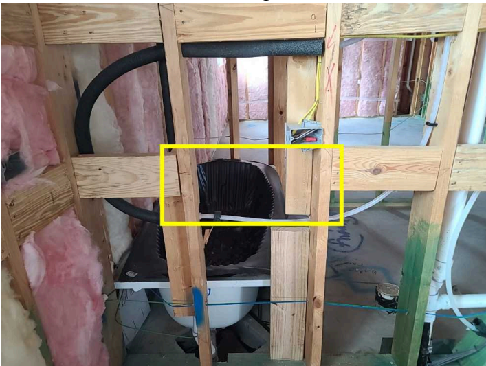
Kitchen cabinet blocking is missing along West wall
