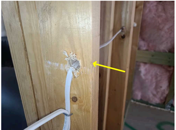
Nail plates missing at office near tub
