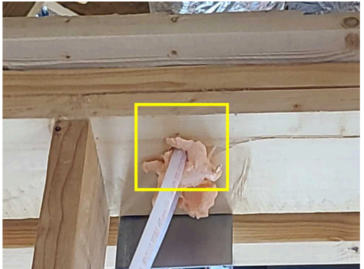
Nail plates missing at refrigerator nook
