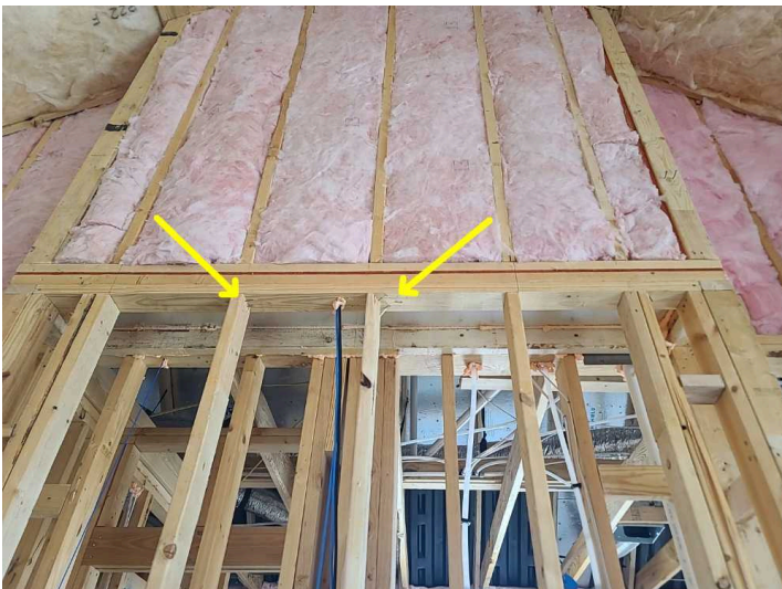
Framing/ stud above fireplace is damaged and are not completely nailed in place properly.
