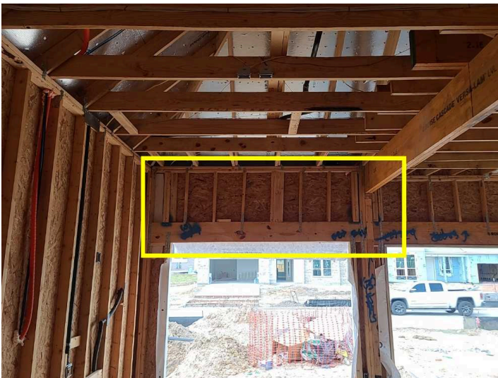
Framing above single bay garage header is not square/ leaning to the right.
