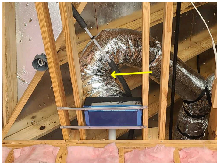
Flex duct excess material in bends; bonus/ flex room.
