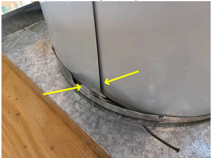
Damage observed to the body of the water heater. Possibility of hidden damage to the unit.
