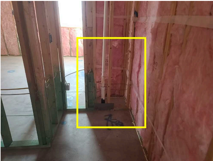
Sink water supply lines and sink drain at laundry room were not present at time of inspection. Should be addressed before sheetrock.
