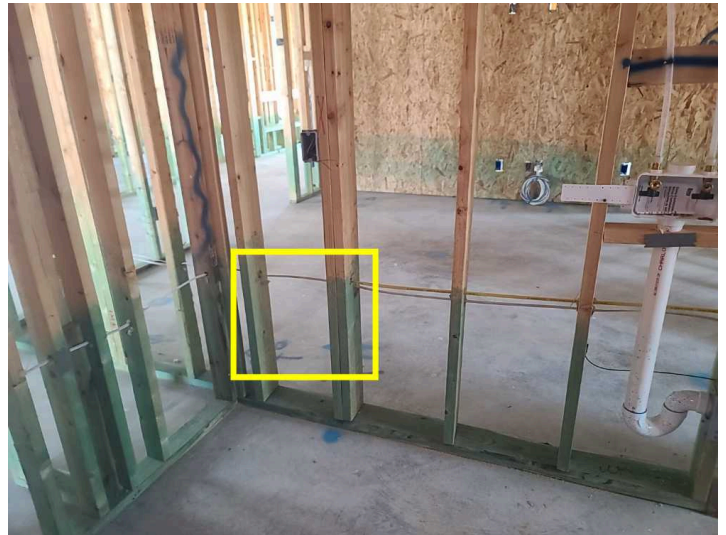
Refrigerator water supply line at laundry room was not present at time of inspection. Should be addressed before sheetrock
