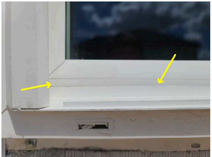
Lower window frames/ sills are not square/ not level. Flanges need adjustment; South bedroom
