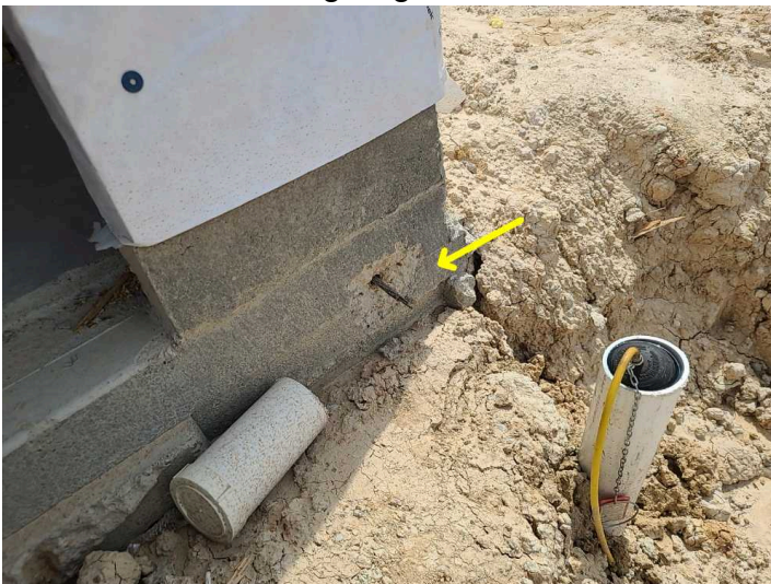
Post tension cable live ends are exposed/ not cut back at all four corners
