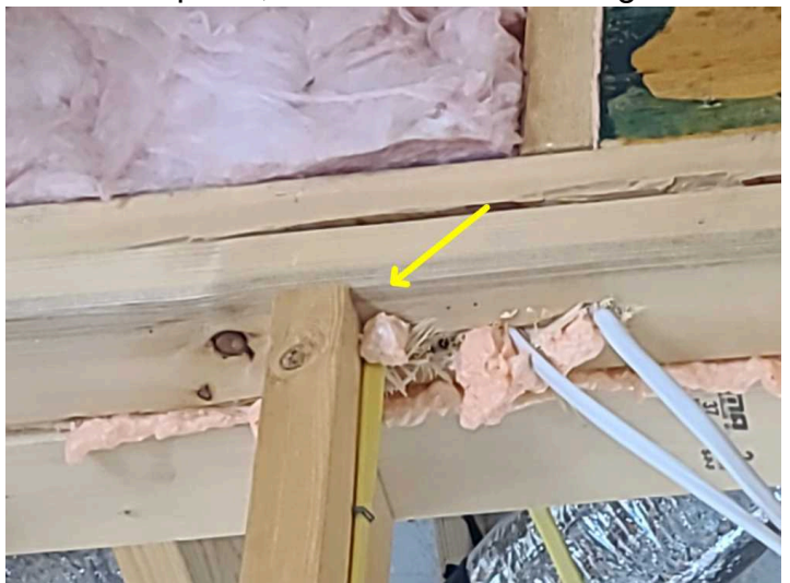
Nail plates missing near kitchen
