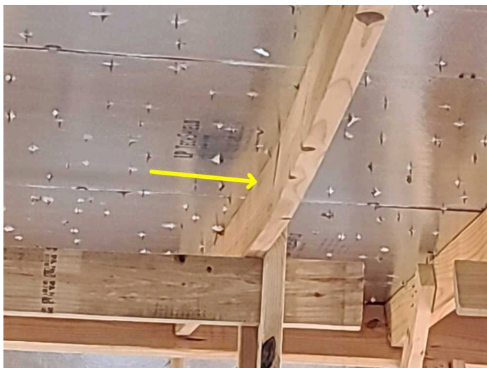
Rafters warped North side of attic above entry hall. Roof decking is not rated for the distance between rafters
