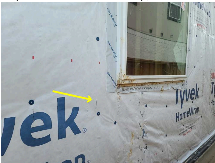
Repair holes/tears in house wrap; North exterior.
