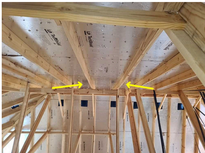
Rafters warped North side of attic above entry hall.
