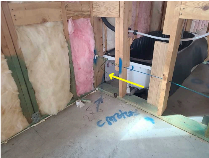
Vertical insulation missing at exterior wall behind/ below South guest tub.
