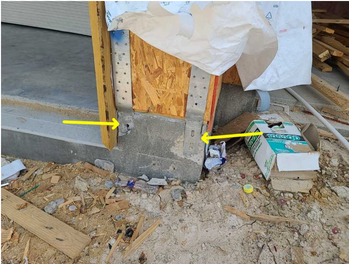
Framing straps appear to have been placed to close to edge, causing concrete to spall; between garages.
