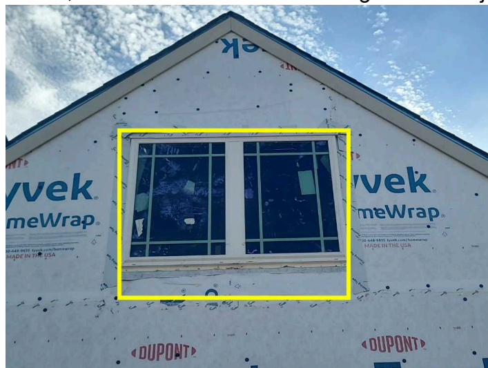
Garage attic windows lost their seals
