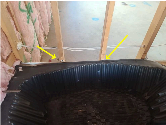
Fiberglass tub securing clips are not properly seated at tub lip; Northwest guest bedroom.
