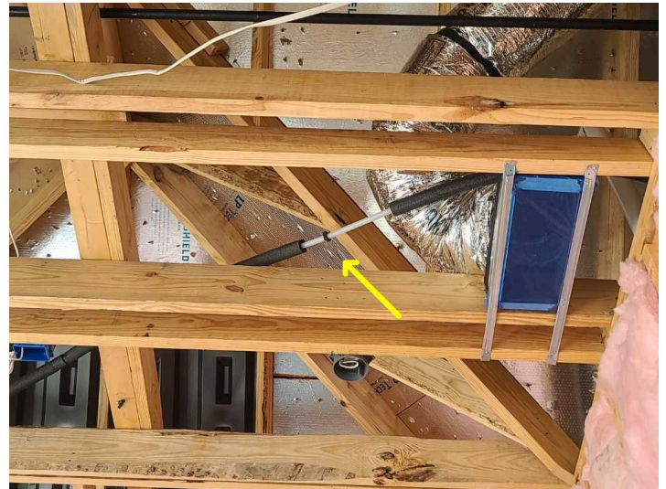
Water supply line not properly secured at; bonus room ceiling
