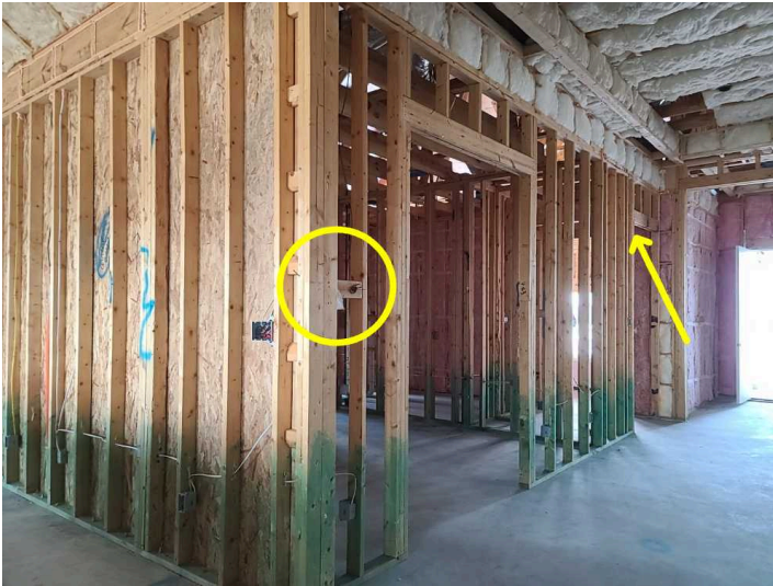
Thermostats are typically/ supposed to be located near the return air chase.
