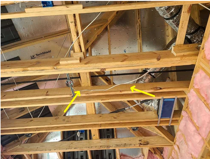
Electrical wiring is not properly secured in place; bonus/ flex room ceiling
