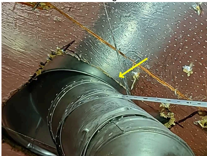
The furnace exhaust vent pipe is in contact with or does not have required minimum 1" clearance from combustible material
