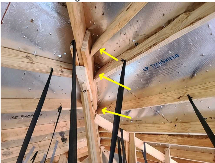
Ends of rafters were observed to be not cut flush with corresponding components; Area that needs repair is above attic access.
