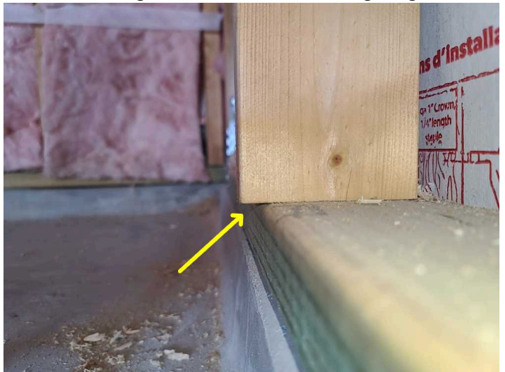
Garage wall stud is not flush with sole plate. May cause a bow in sheetrock.
