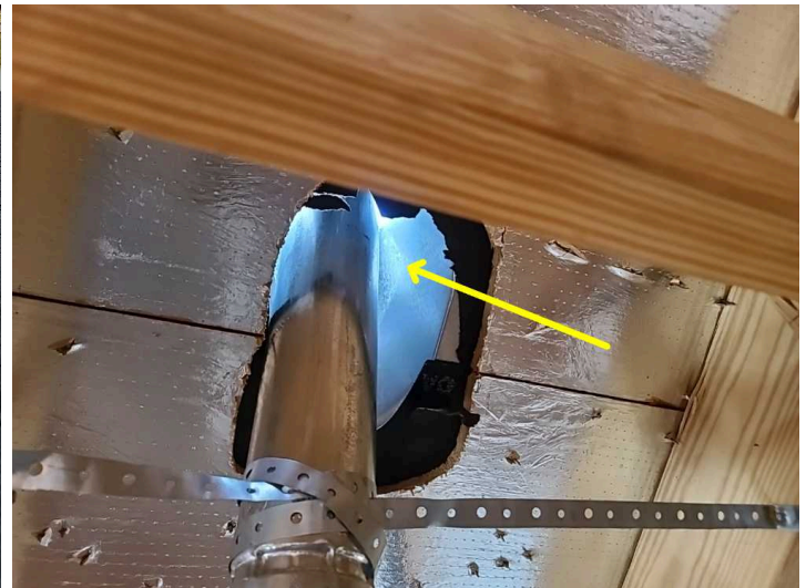
Storm collar not properly positioned on water heater vent pipe, daylight observed in attic.
