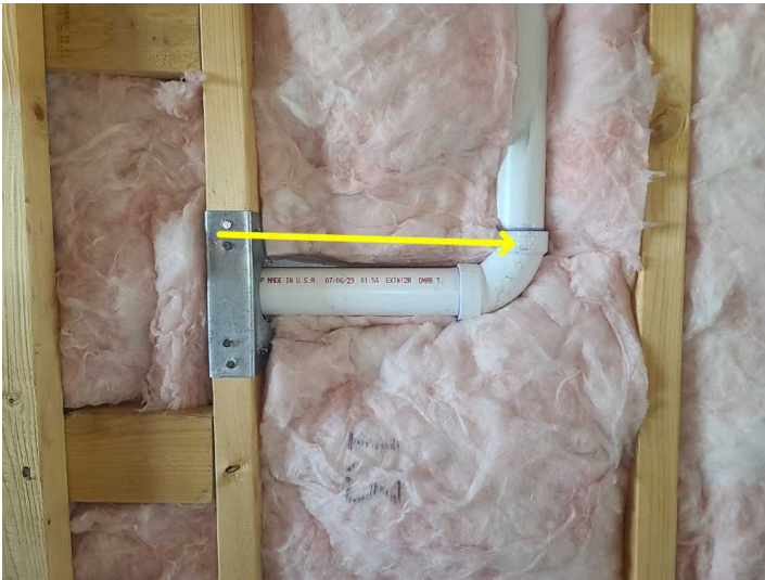
Improper slope of the drain waste vent line observed. The line does not tilt downhill for drainage of condensate; office exterior wall
