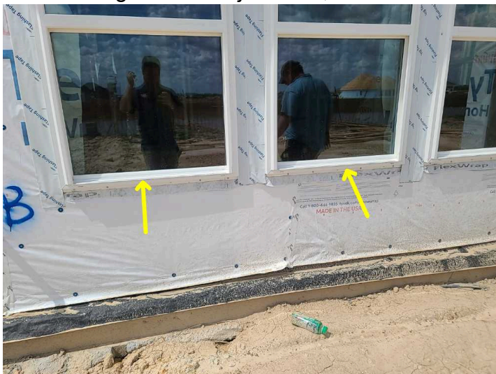
Lower window frames/ sills are not square/ not level. Flanges need adjustment; bonus/ flex room
