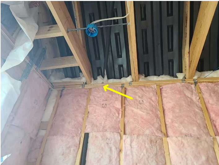
Nail plates missing at Northwest corner bedroom
