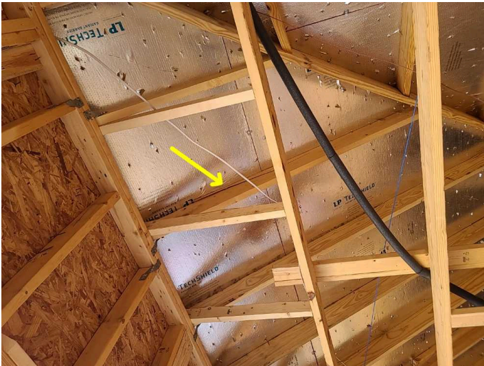
Damaged / cracked / split rafter observed above; guest bedroom.
