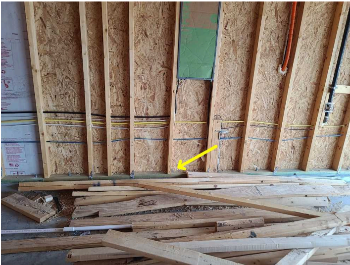
Wall framing not properly attached to foundation, missing a washer, and a nut; garage
