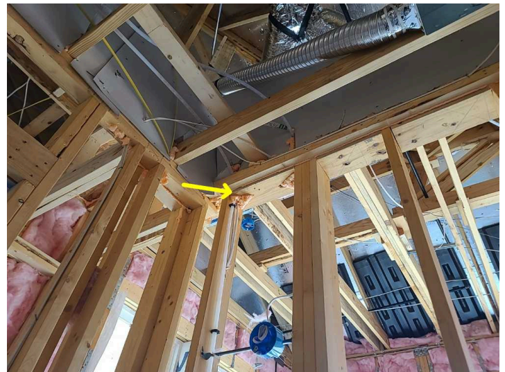
Nail plates missing at half bath
