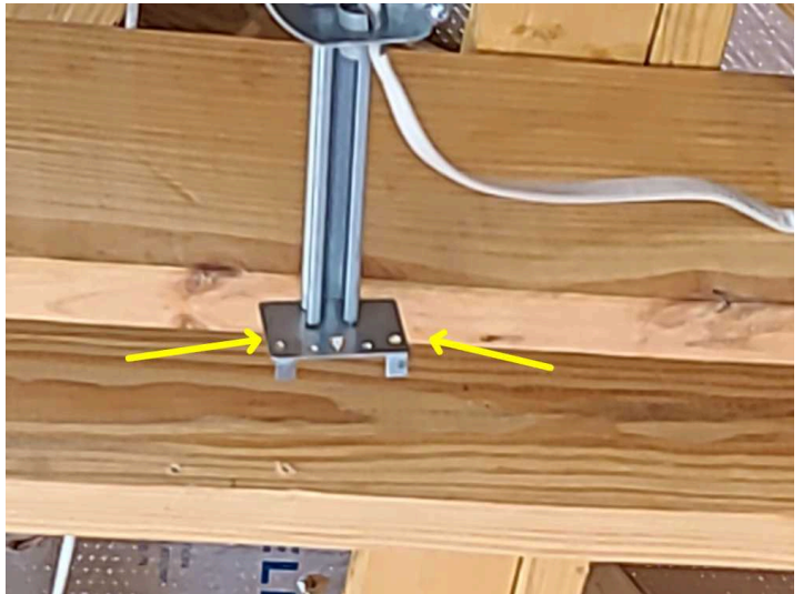
Fixture boxes are not properly secured in place, pulled loose for added framing; bonus/ flex room ceiling.
