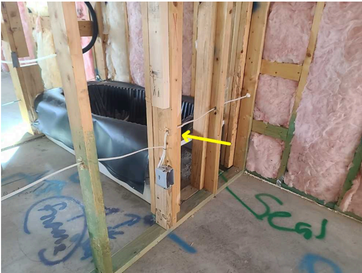
Nail plates missing at office near tub
