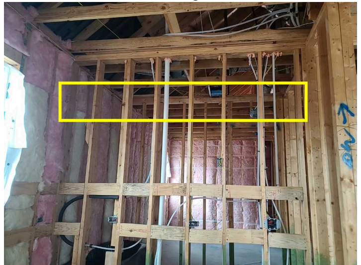
Kitchen cabinet blocking is missing along West wall. Additional blocking is needed to properly attach/ support cabinetry.
