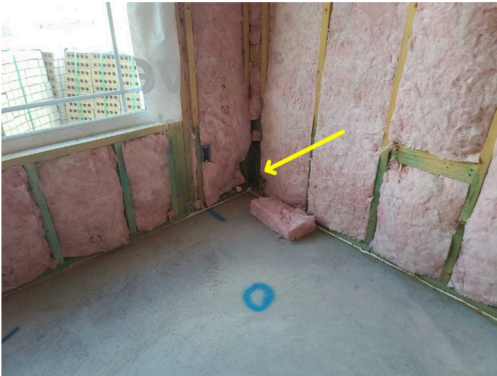
Wall framing not properly attached to foundation, missing a washer, and a nut; Northwest corner/ bedroom
