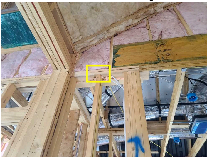
Nail plates missing near kitchen
