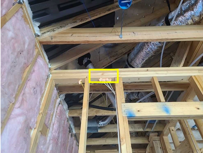
Nail plates missing at Northwest bedroom
