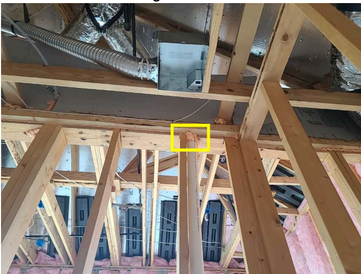
Nail plates missing at half bath
