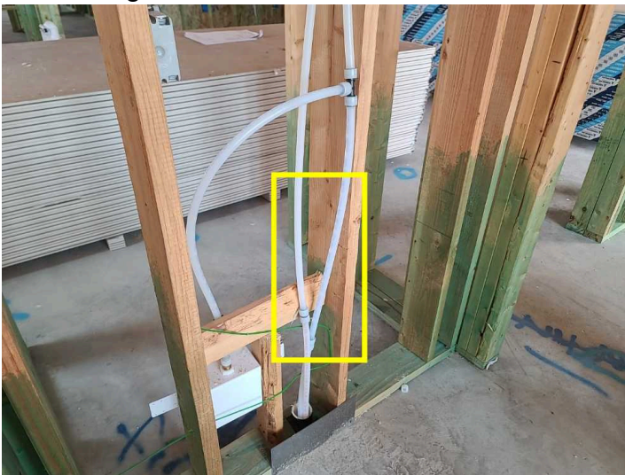
Water supply line not properly secured at; refrigerator area
