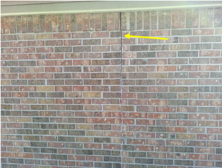
Uneven crack in the left wall
