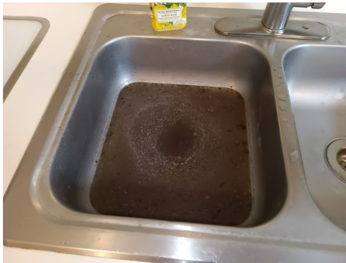
Garbage disposal is non functional and the drain is plugged
