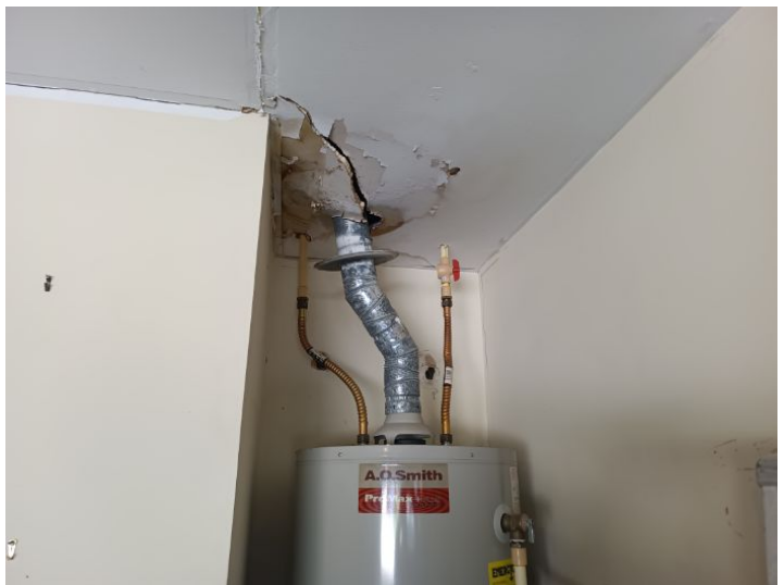
Garage ceiling is detached
