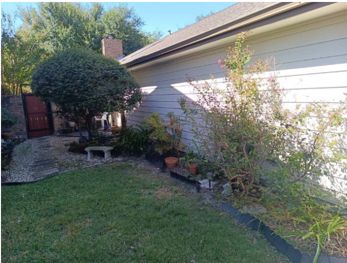
Foliage is <18" from the structure
