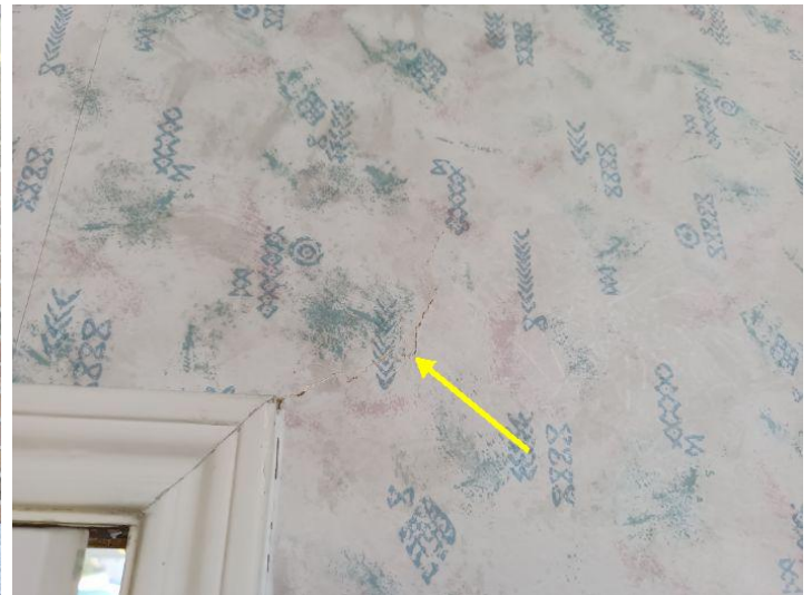
Stress crack in the dining room wall
