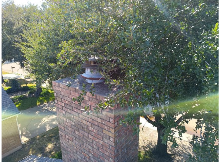
Tree branches are <10' from the chimney
