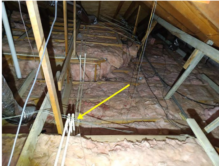
uninsulated pipes in the attic
