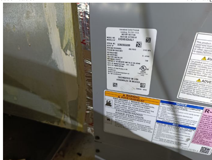
AC evaporator coil label
