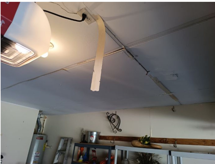
Garage ceiling is not secure
