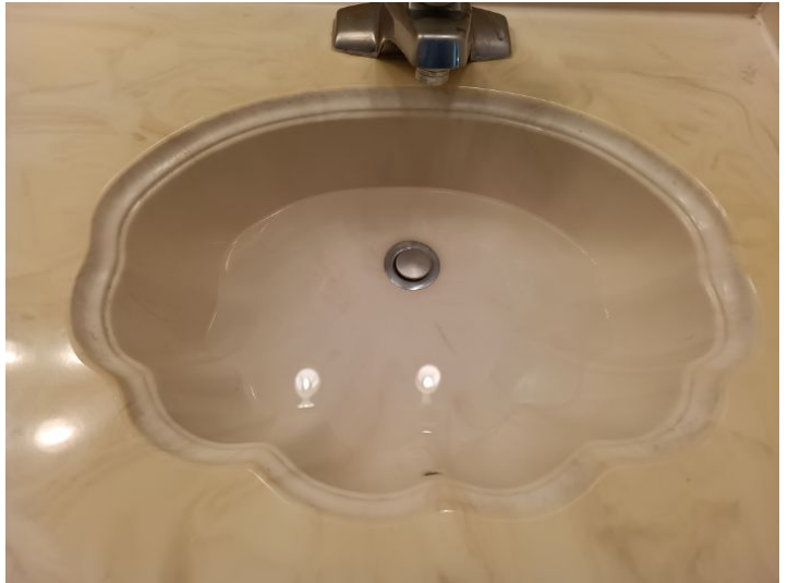
Right sink in the primary bathroom is slow to drain
