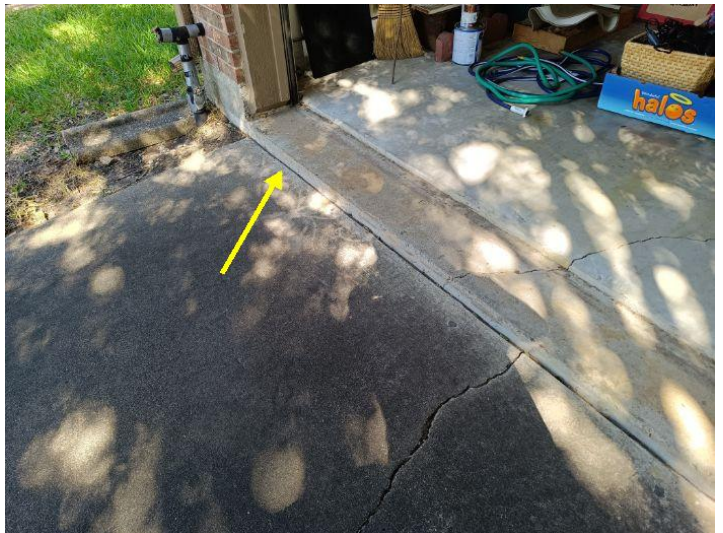
Driveway has settled 4"
