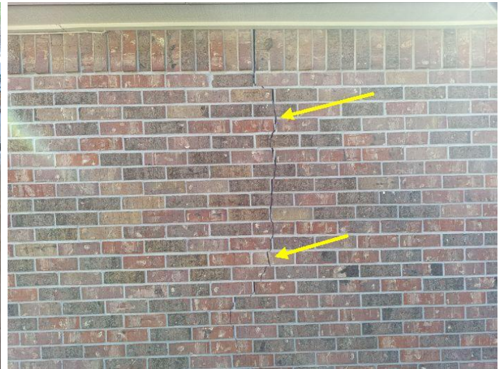
Cracks in the brickwork in the left wall
