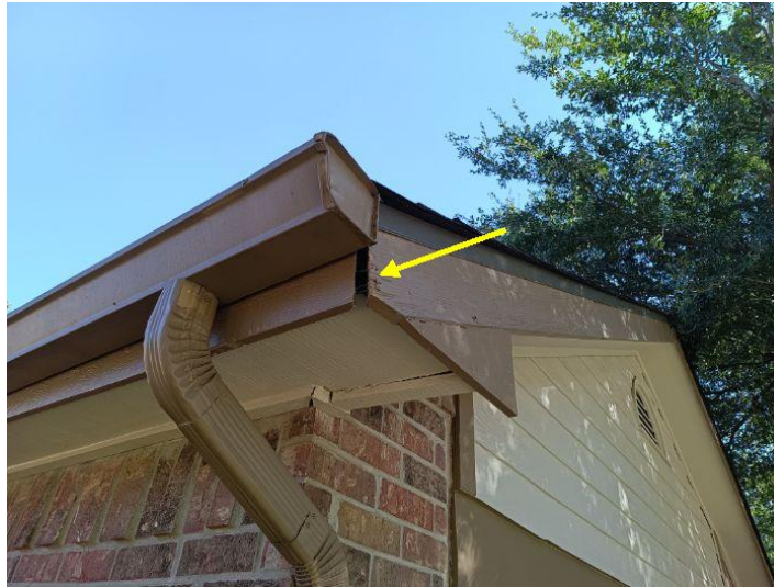
Detached trim by the garage
