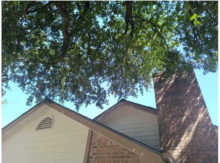
Tree branches are <3' from the structure
