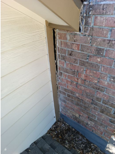
Chimney has separated from the house, leaf buildup
