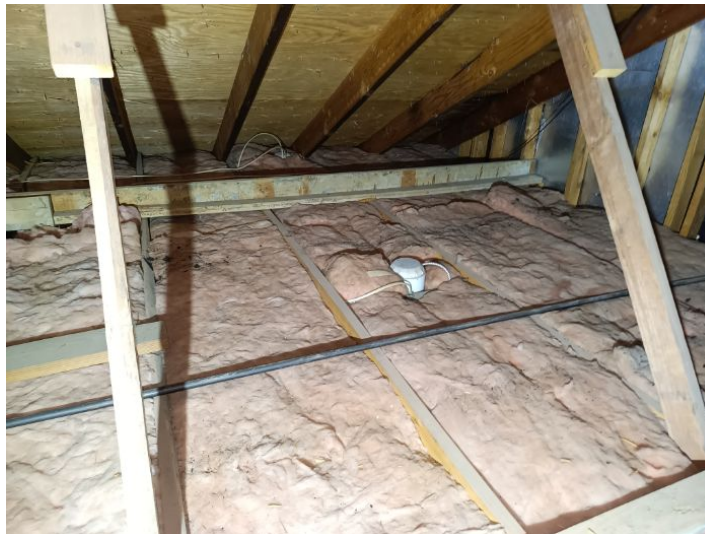
non IC-rated lights are <3" away from insulation
