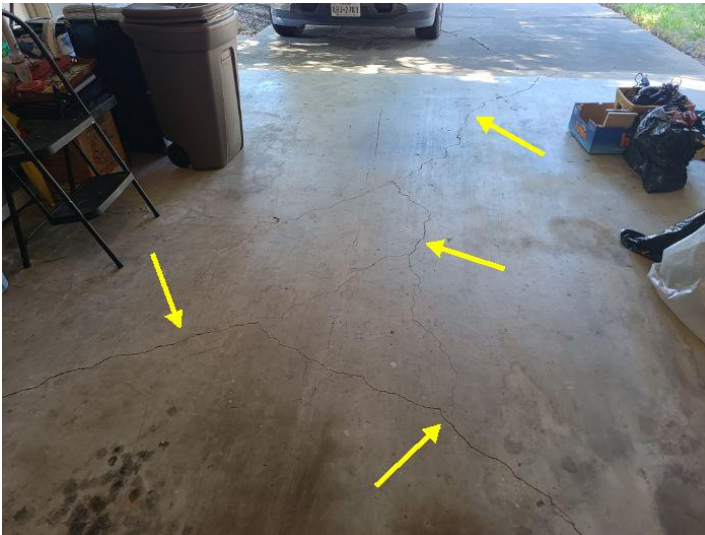
Cracks in the garage floor
