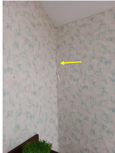
Stress in the wallpaper from the foundation shifts
