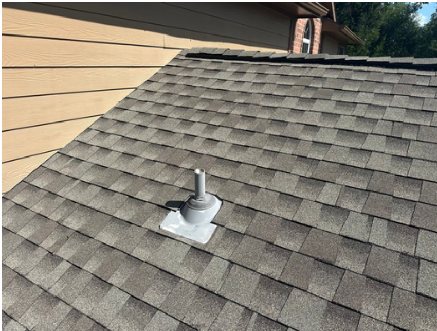
Side pipe jack cover. Excellent condition
