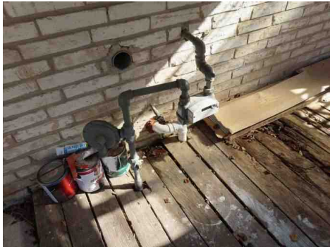
Unit B Gas Meter
