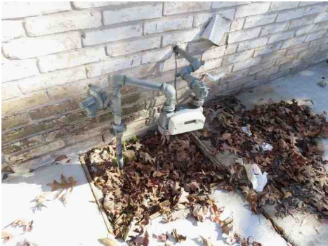
Unit A Gas Meter
