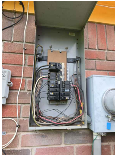
The service panel with the cover removed.
