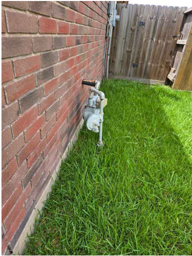
Type of Gas: Natural Gas Type of Gas Distribution Piping Material: Black Steel
