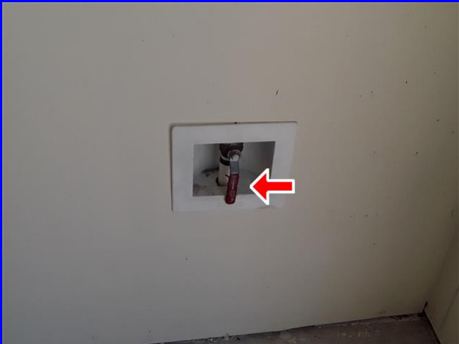
main water shutoff valve located in the garage on the right wall
