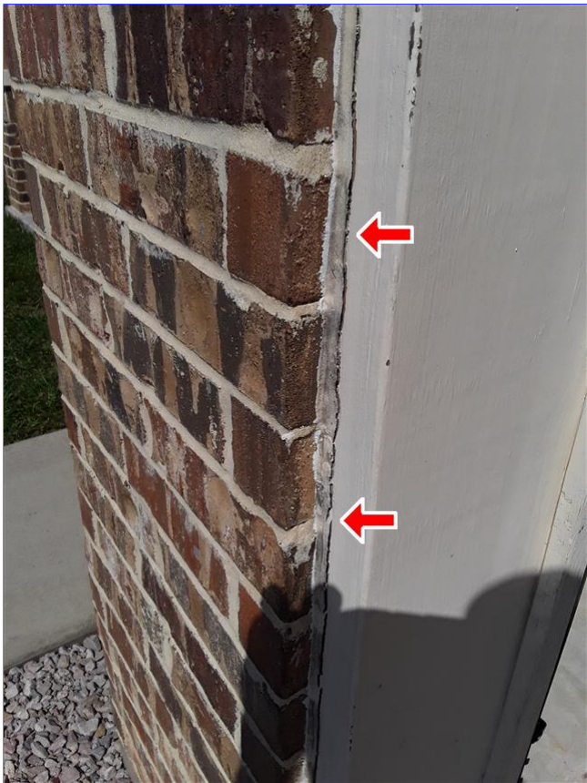
L. Item 4 (Picture) seal around the garage door jambs
