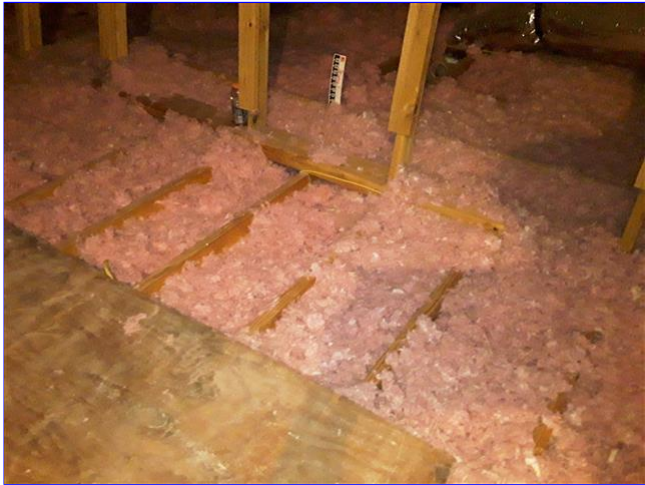
D. Item 1 (Picture) additional insulation needed in multiple locations
