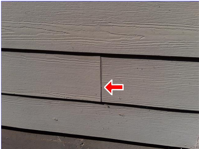
L. Item 3 (Picture) seal all cracks and gaps in the exterior
