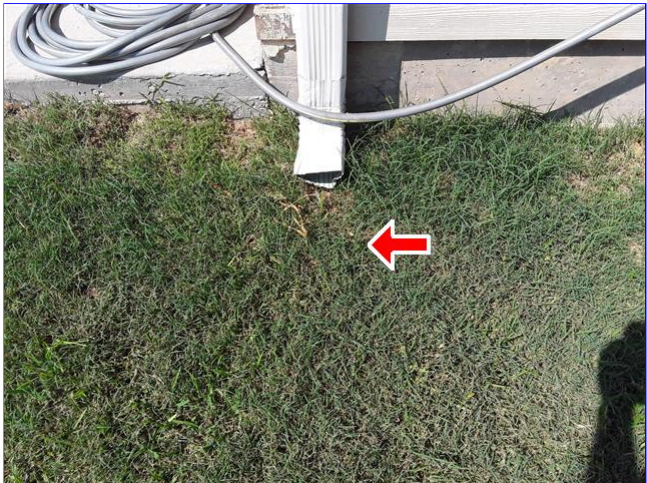
B. Item 1 (Picture) multiple locations
