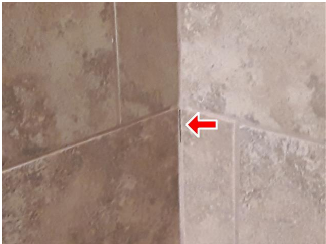
L. Item 1 (Picture) seal around the shared bathroom tub
