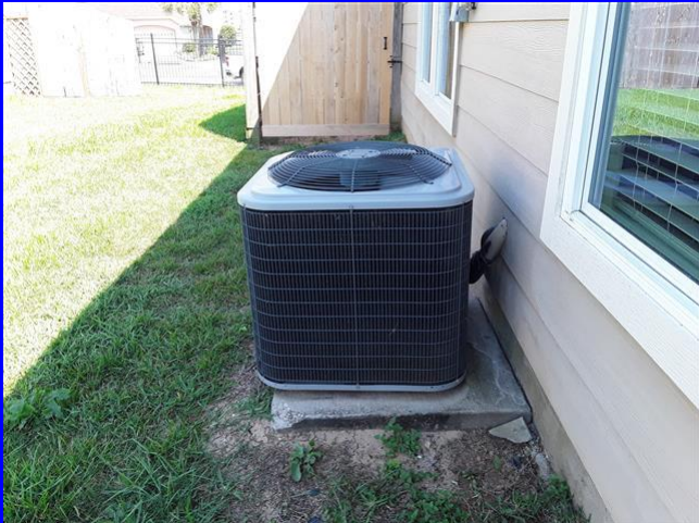
Condensing unit located on the left side of the home
