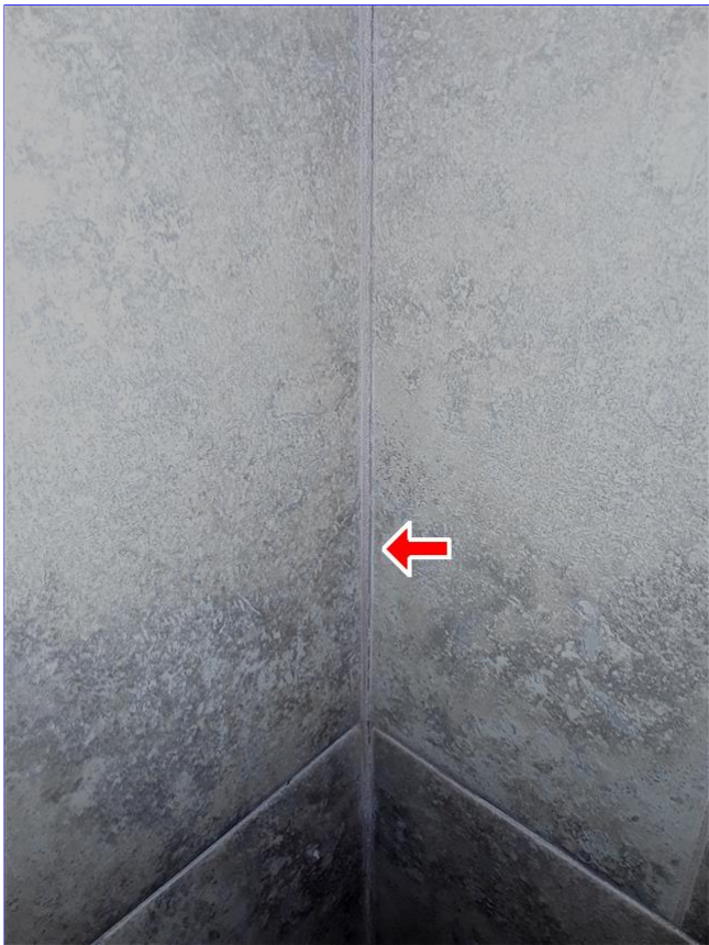
L. Item 2 (Picture) seal around the master shower
