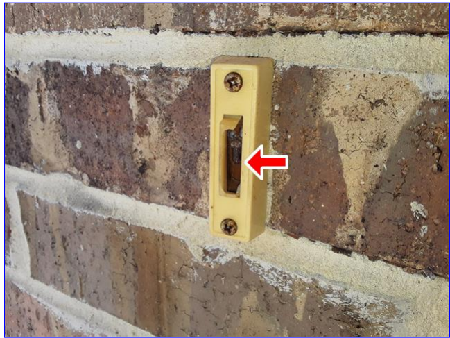
B. Item 2 (Picture) doorbell button is damaged
