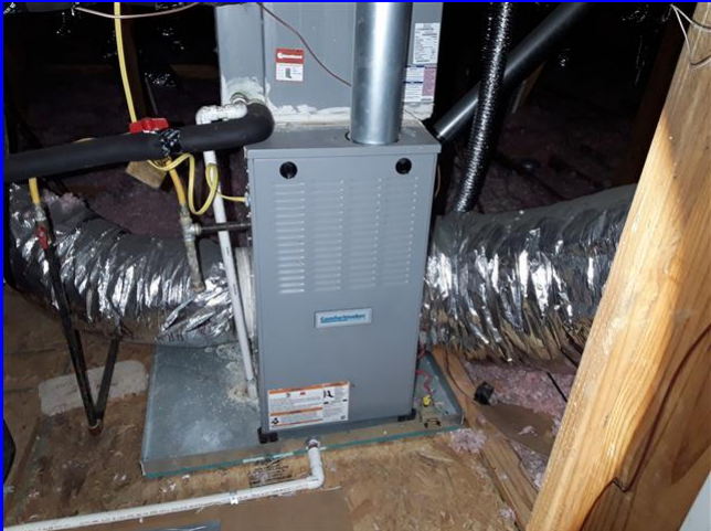
Comfortmaker gas furnace located in the attic
