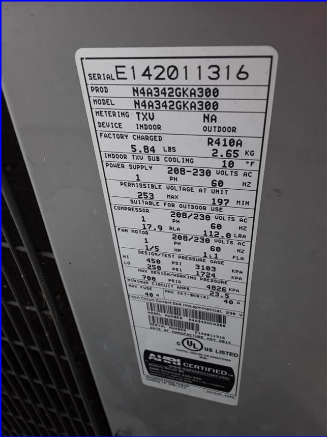
condensing unit label
