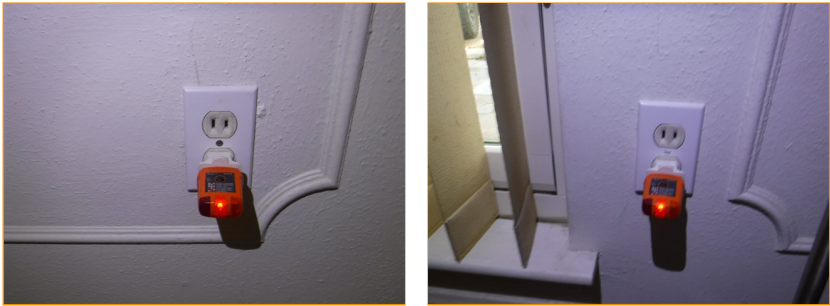
Older two prong outlets with no grounding bare wire observed at various locations around the house.
