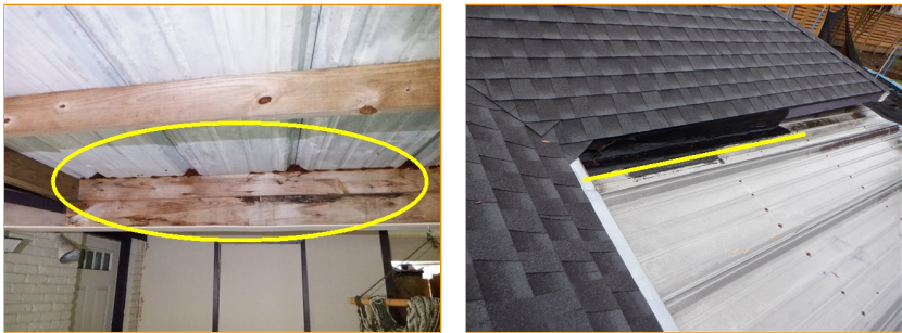
Deficient sealing and evidence of water penetration observed in the carport.
