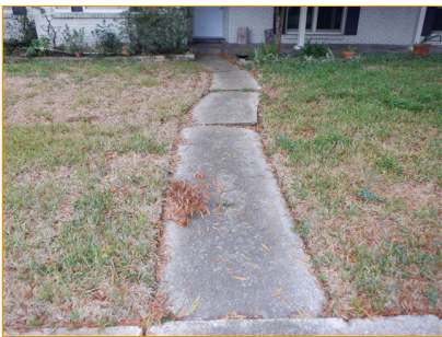
Tripping hazard observed at front of the house; the walkways and/or driveways are uneven.
