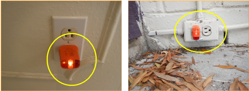
3 prong outlet(s) with an open ground observed at various locations around the house.
