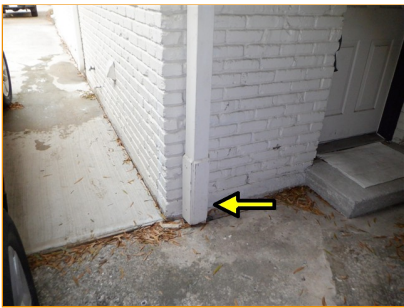
Observed wood support column at the covered garage walkway is loose from the ground.
