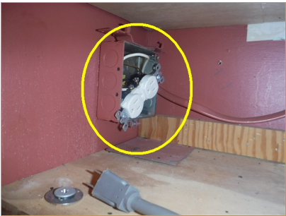
Electrical outlet not properly secured to the wall and/or missing the cover plate observed in the kitchen.
