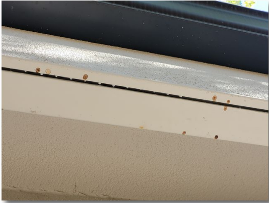
2- 1.11 Dark stains present at drainage relief.
