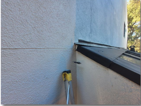
4- 1.5 Test Location G - Soft substrate encountered
