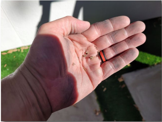
2- 6.1 Damaged substrate from behind the casing bead.
