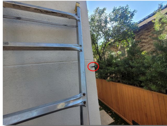
1- 1.2 Test Location J - Soft substrate encountered
