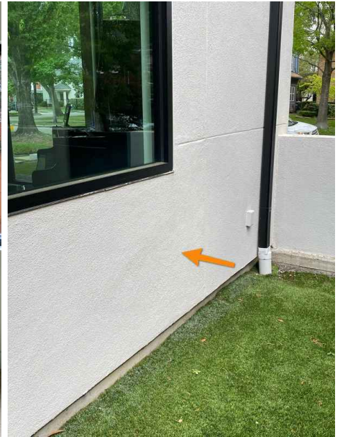
Opposite side of the wall/ possible previous repair
