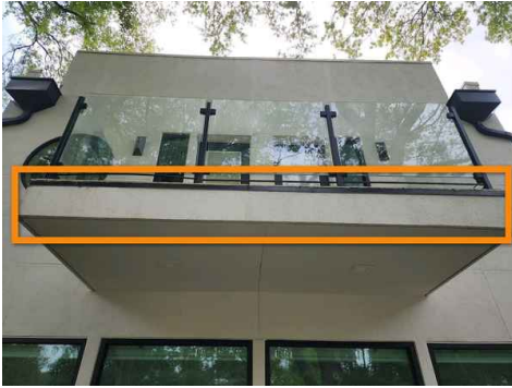
Discoloration: Front Elevation
