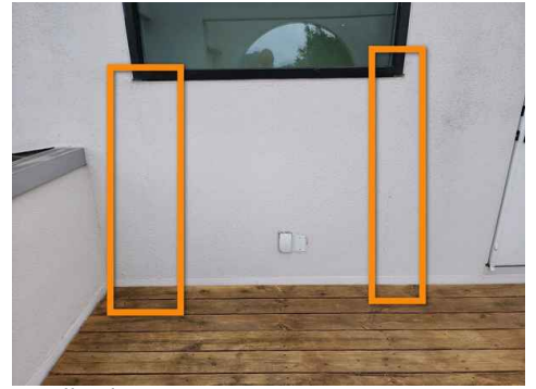
Caulked Over: Terrace
