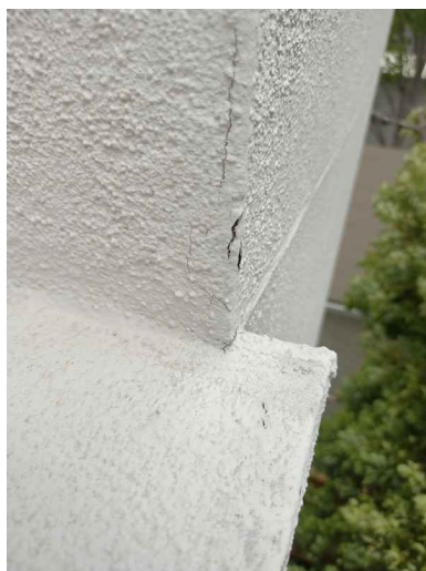
3rd Floor cracks
