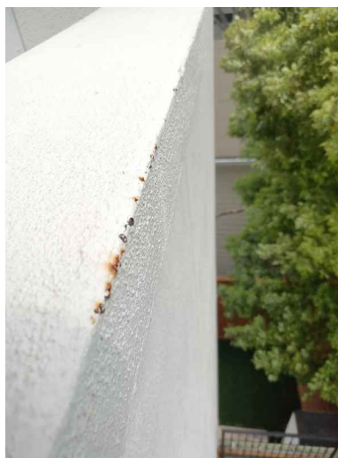
3rd Floor corrosion
