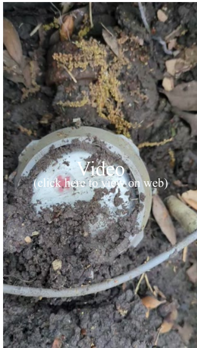
Location of Main Water Supply Valve: Exterior Wall - Right Side
