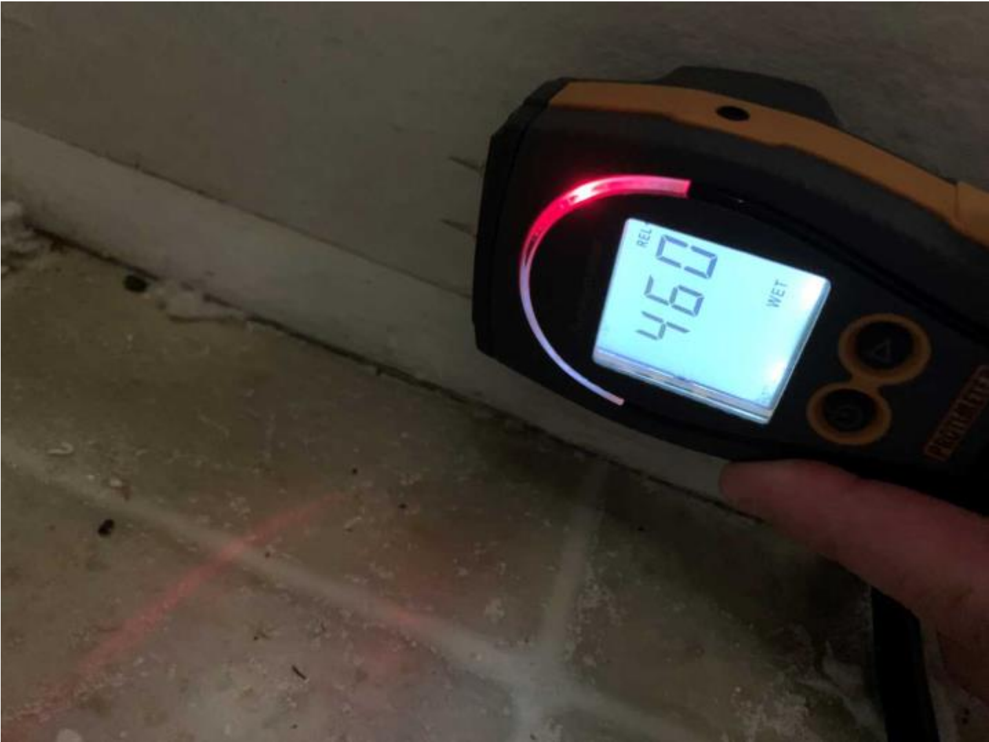
16 16-bathroom after 24hr of drying Date Taken: 9/23/2021
