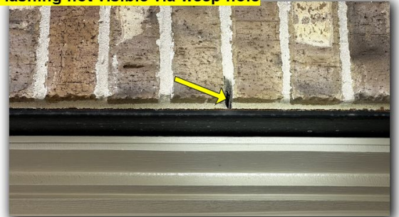
Flashing not visible via weep hole
