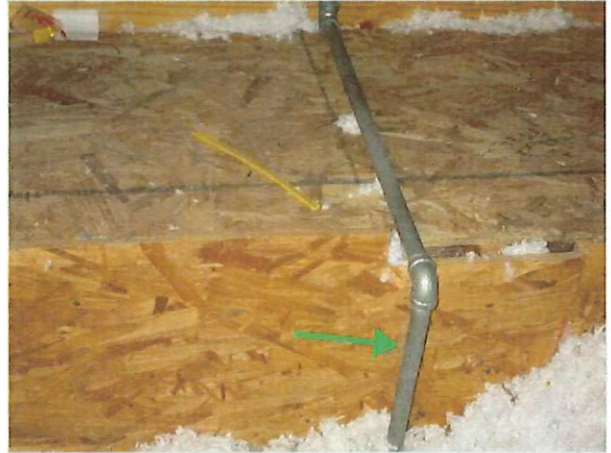
galvanized steel gas line
