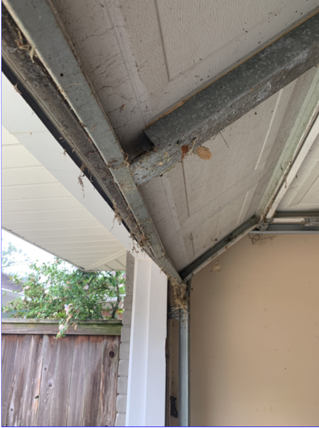
G. Item 1(Picture) Damage was observed to both garage doors. The weather stripping on both is deteriorated. Both doors do open.
