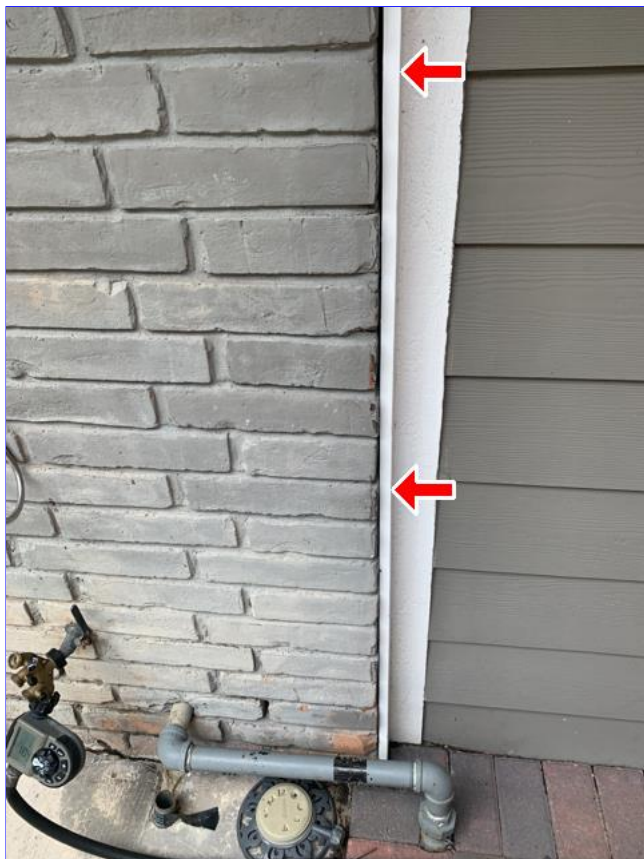
E. Item 8(Picture) Areas around the home where the brick, trim, and siding meet, need to be caulked and sealed.
