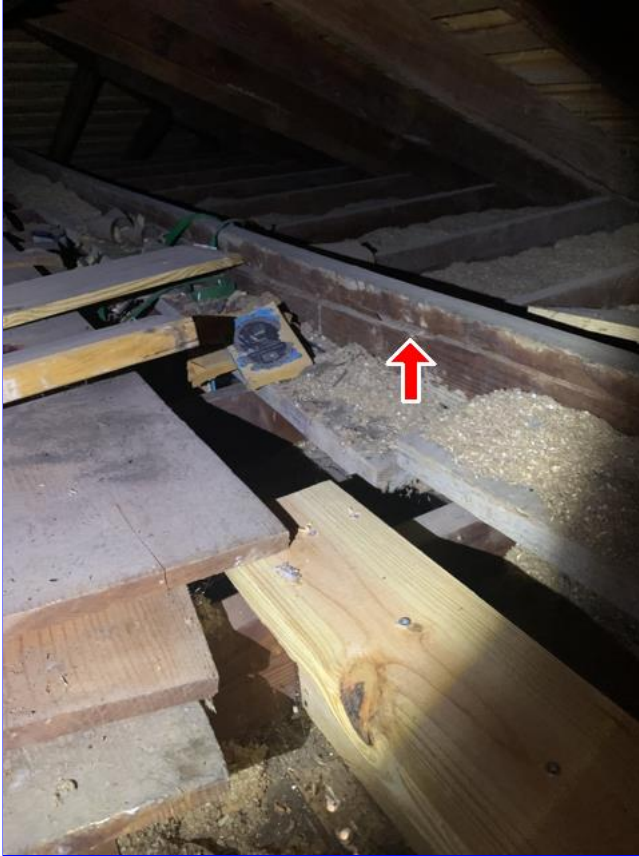
D. Item 3(Picture) The strong back bracing over the garage has a crack or has been cut. Recommend having a contractor to evaluate.
