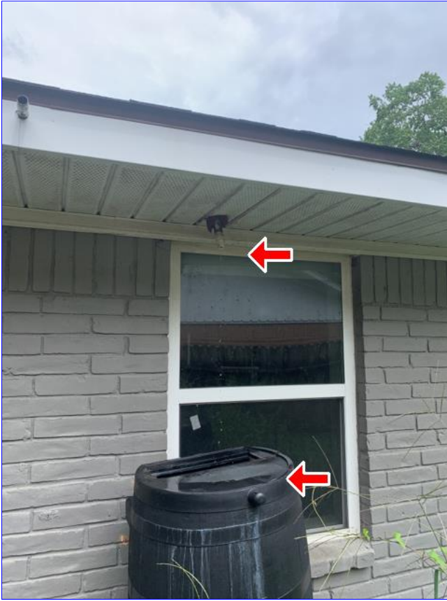
B. Item 3(Picture) The AC drain line was observed to be draining into a barrel outside.
