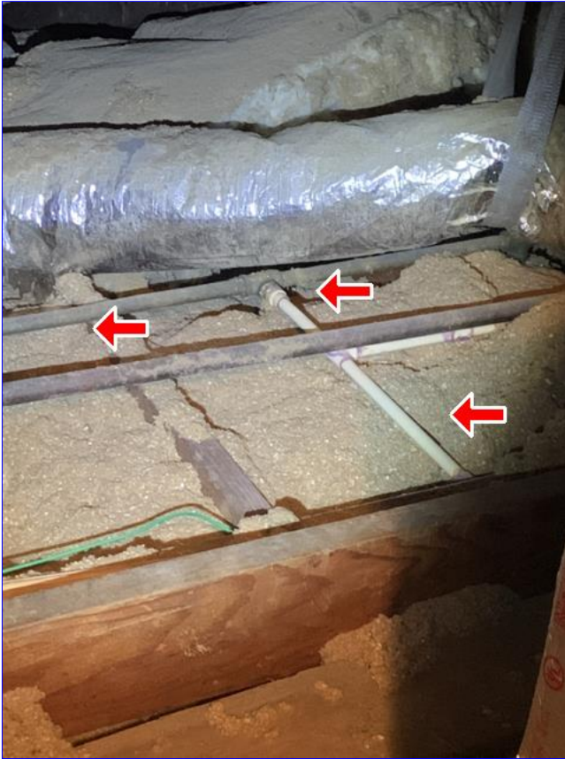
A. Item 7(Picture) Exposed water pipes observed in the attic space are not properly protected from freezing.
