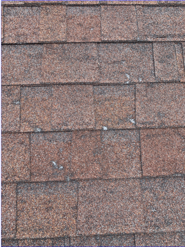
C. Item 2(Picture) The roof covering, is not new and shows signs of wear consistent with its age. Hail damage was observed on the south facing area of the roof.
