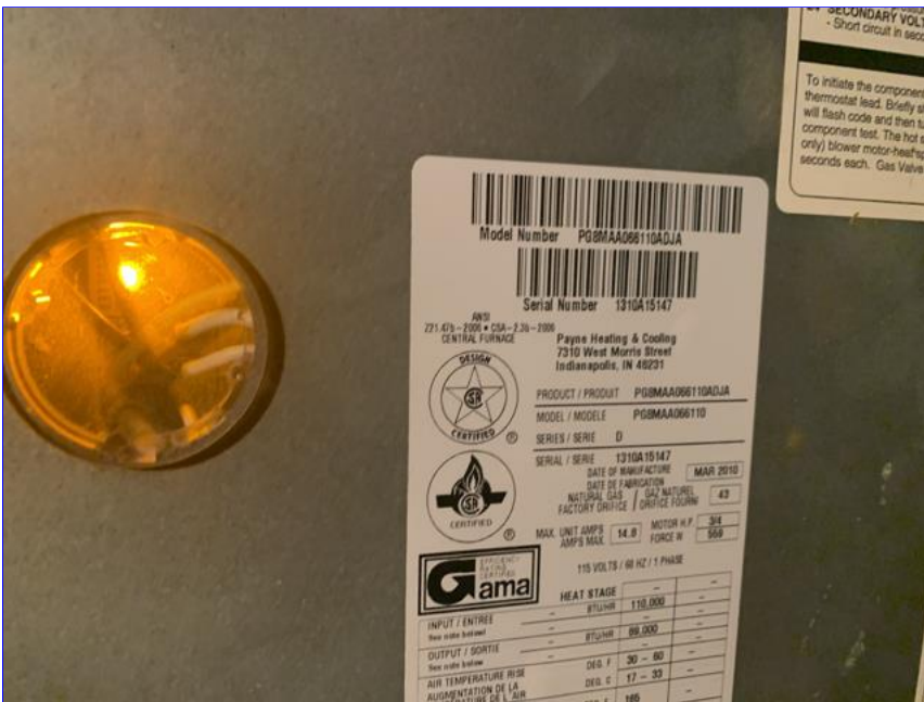
A. Item 2(Picture) Furnace service tag
