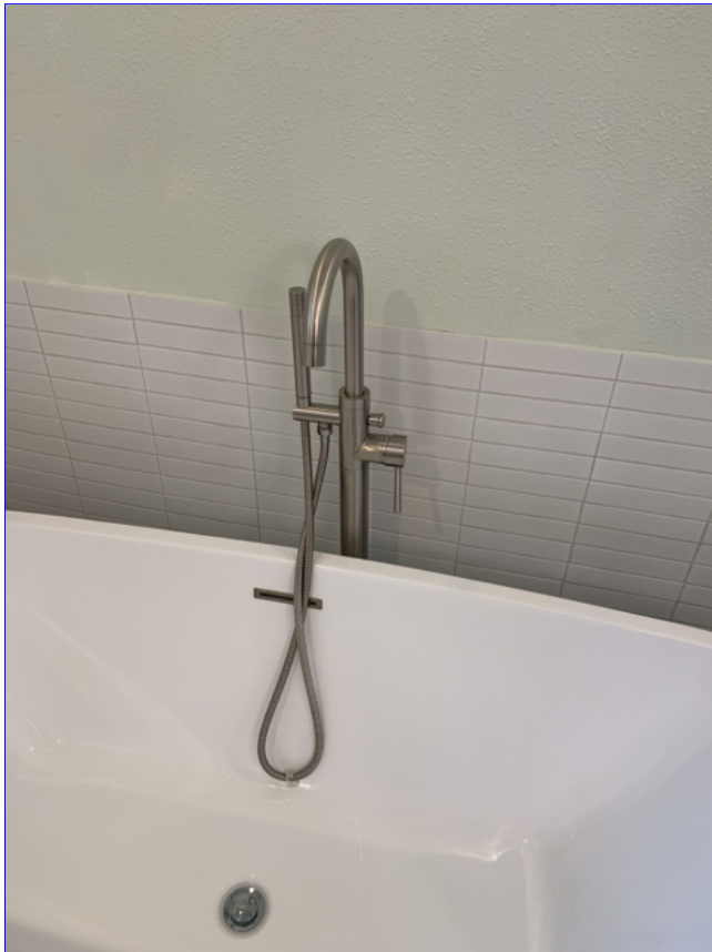
A. Item 6(Picture) The faucet stand for the master bath is loose. Recommend correction.
