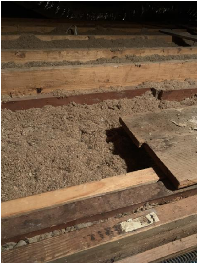
D. Item 5(Picture) The insulation in the attic is very thin. Recommend correction.
