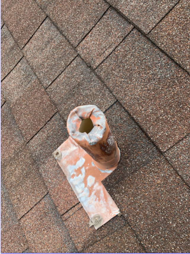
C. Item 9(Picture) Flashing need to be replaced.
