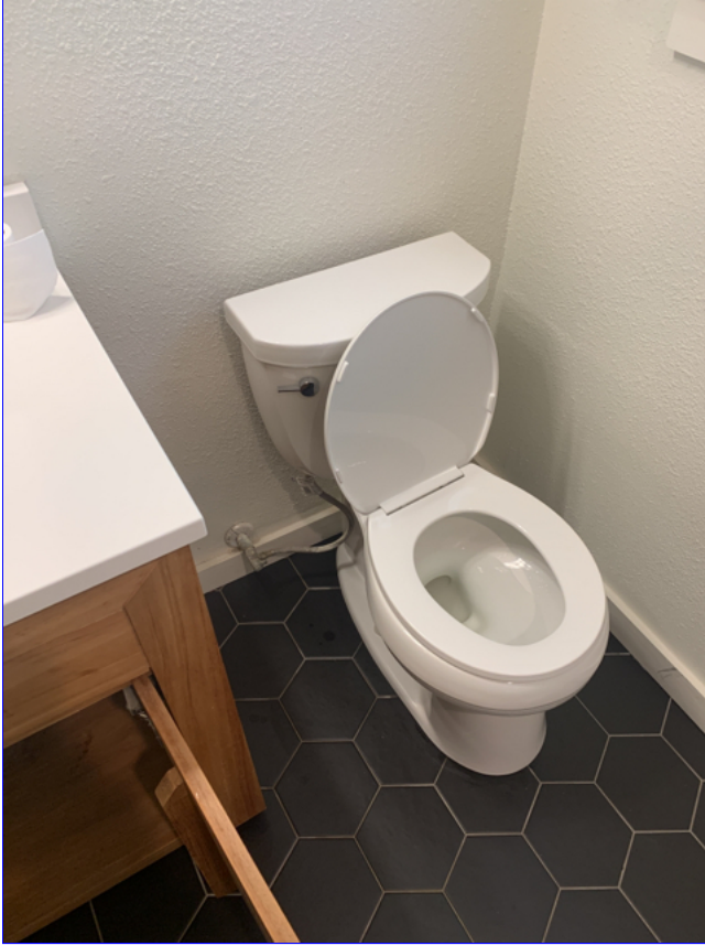
A. Item 2(Picture) The toilet is loose at floor at the bath.
