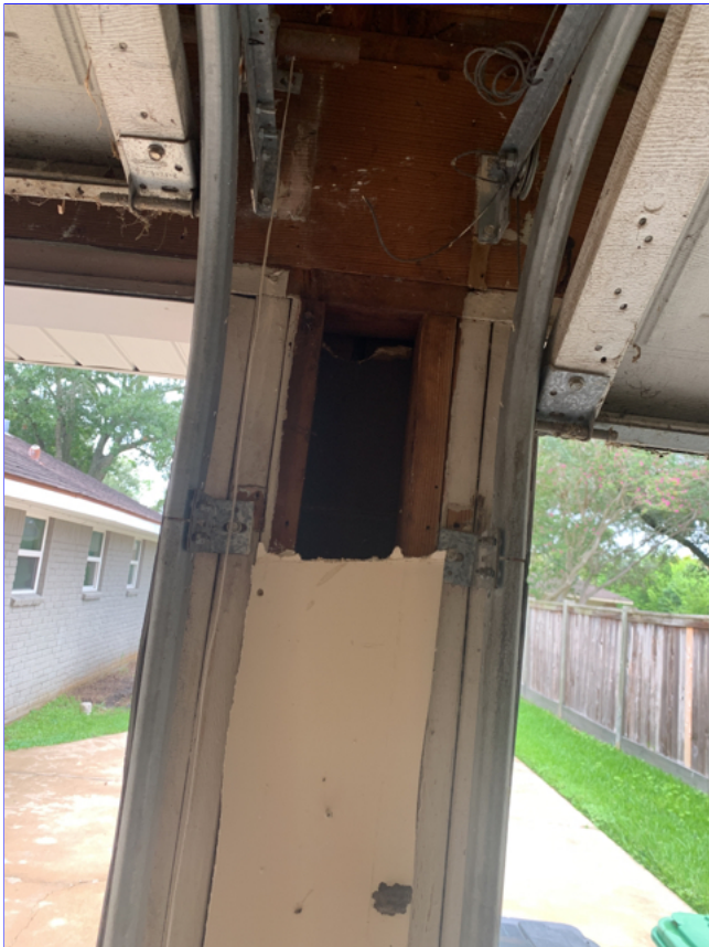
E. Item 2(Picture) Drywall was missing in parts of the garage. Recommend correction.
