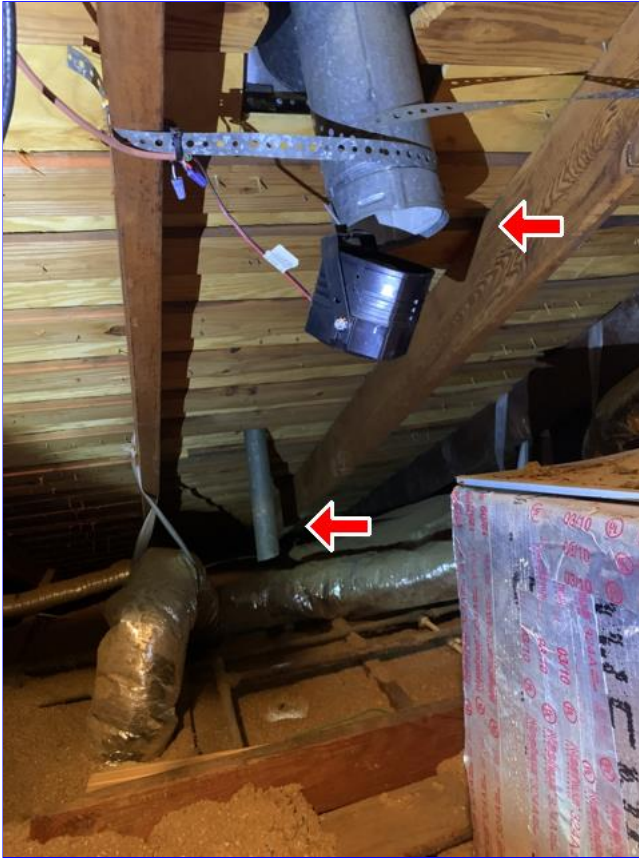
C. Item 11(Picture) Old vents need to be removed.
