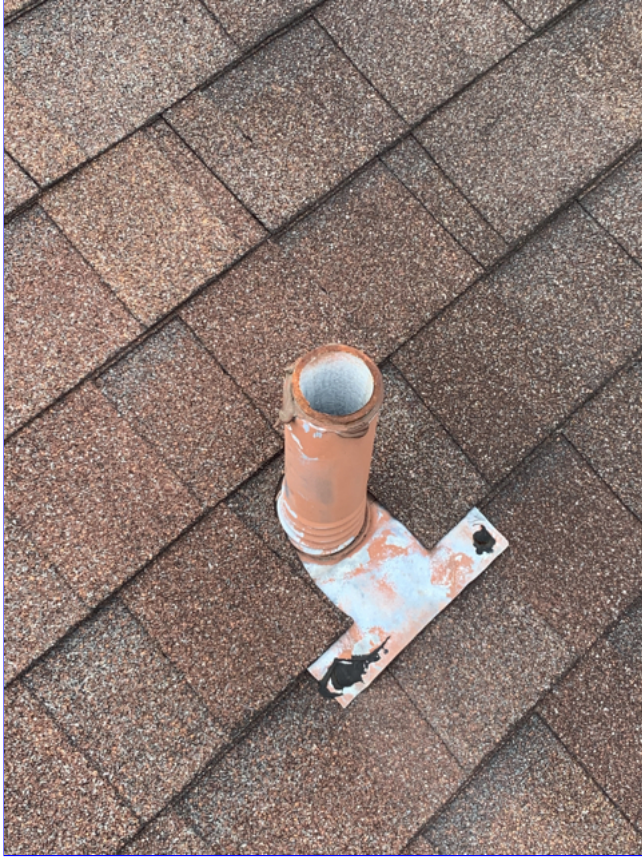
C. Item 7(Picture) Flashing need to be replaced.
