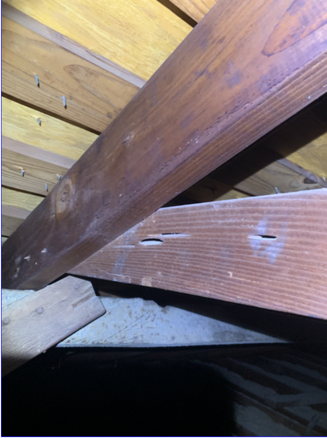
D. Item 1(Picture) Termite damage observed over garage.
