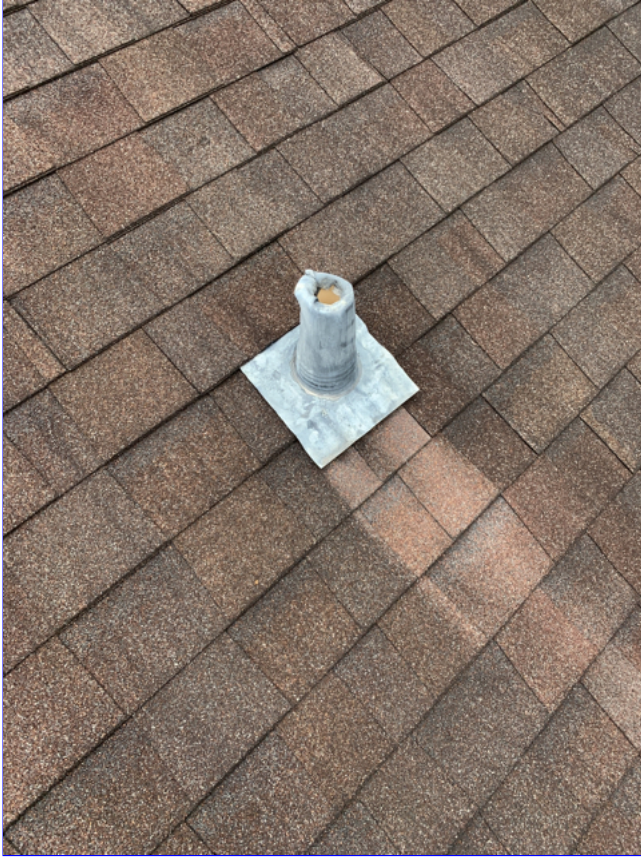
C. Item 8(Picture) Flashing need to be replaced.
