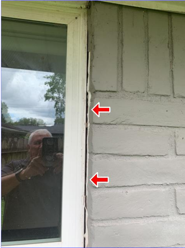
H. Item 1(Picture) The perimeter sealant, has failed on some windows. Recommend caulking.
