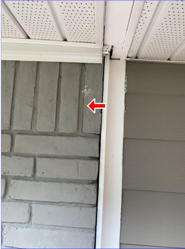
E. Item 4(Picture) Brick veneer mortar cracks were observed.
