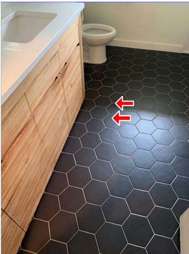
F. Item 2(Picture) Some floor tiles are not fully set to slab.
