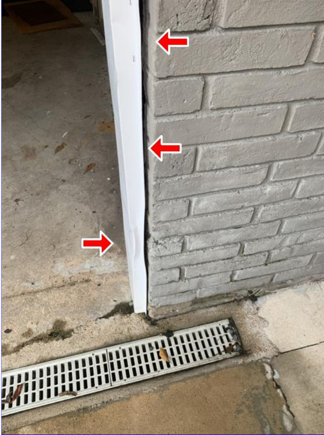
G. Item 3(Picture) Damage to the garage door trim and areas that need to be caulked were observed.
