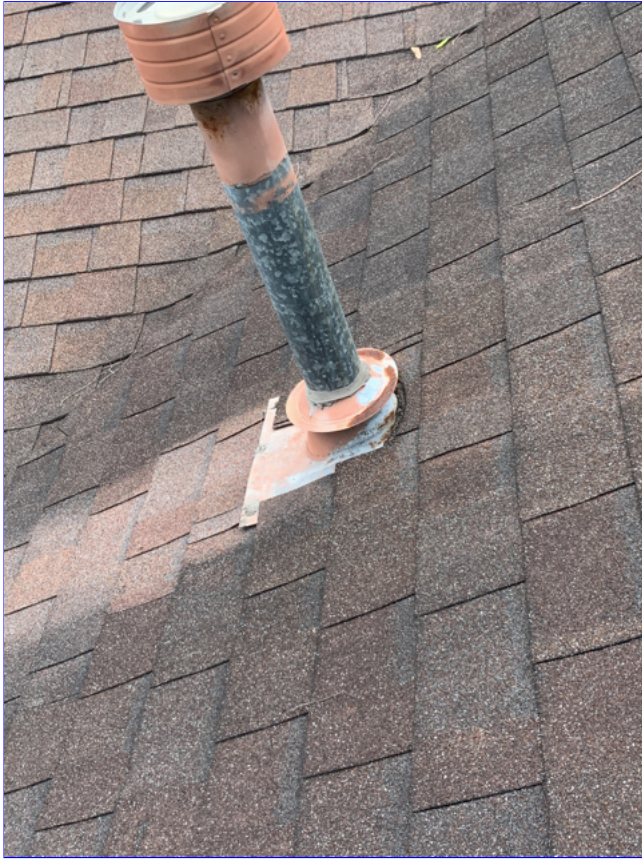
C. Item 10(Picture) Flashing need to be replaced.
