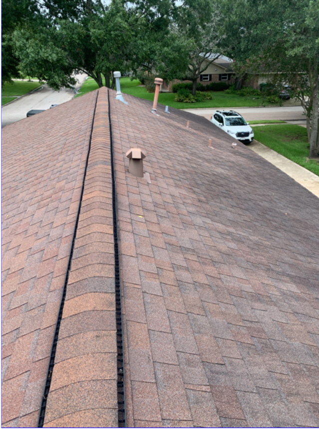
C. Item 5(Picture) The roof covering, is not new and shows signs of wear consistent with its age. Hail damage was observed on the south facing area of the roof.
