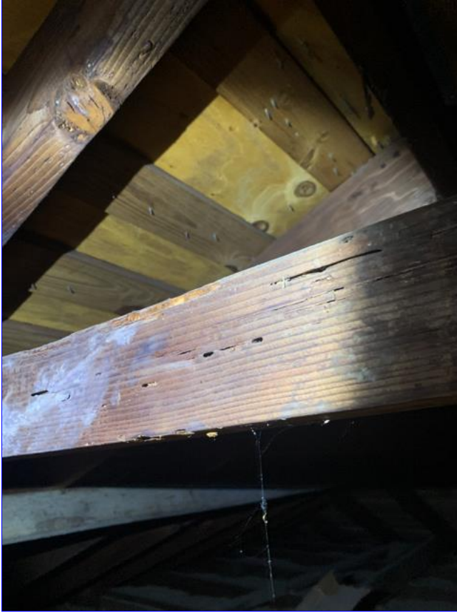
D. Item 2(Picture) Termite damage observed in the attic over garage.
