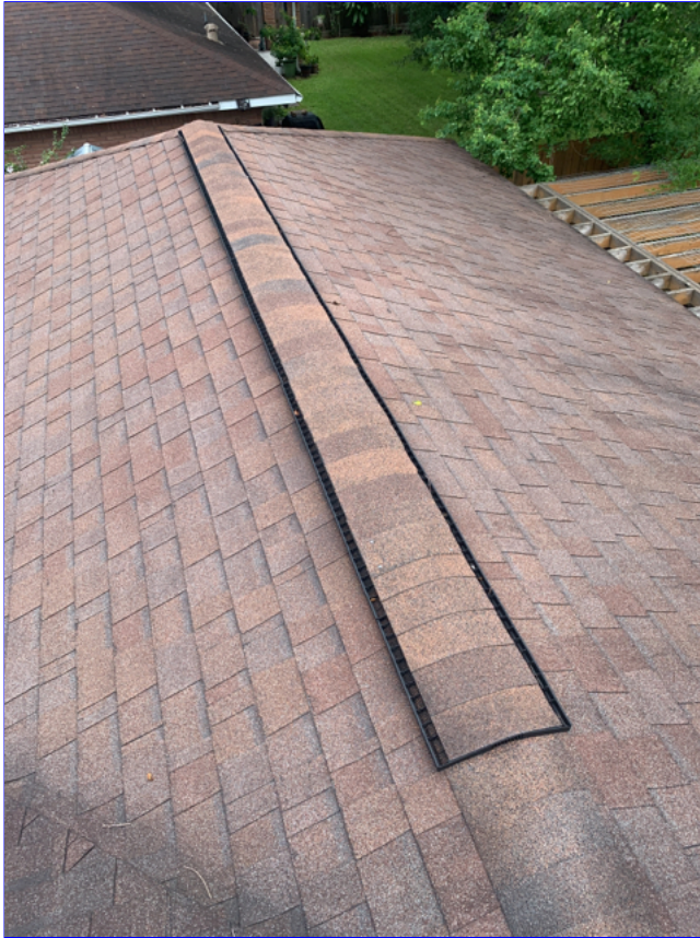
C. Item 6(Picture) The roof covering, is not new and shows signs of wear consistent with its age. Hail damage was observed on the south facing area of the roof.
