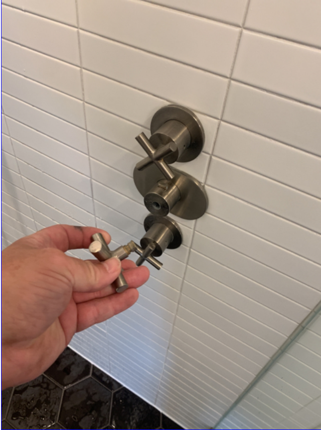
A. Item 4(Picture) Faucet handles at the master shower are loose and in need of adjustment. Recommend correction.
