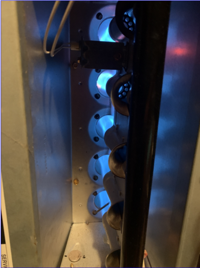
A. Item 1(Picture) Furnace burners
