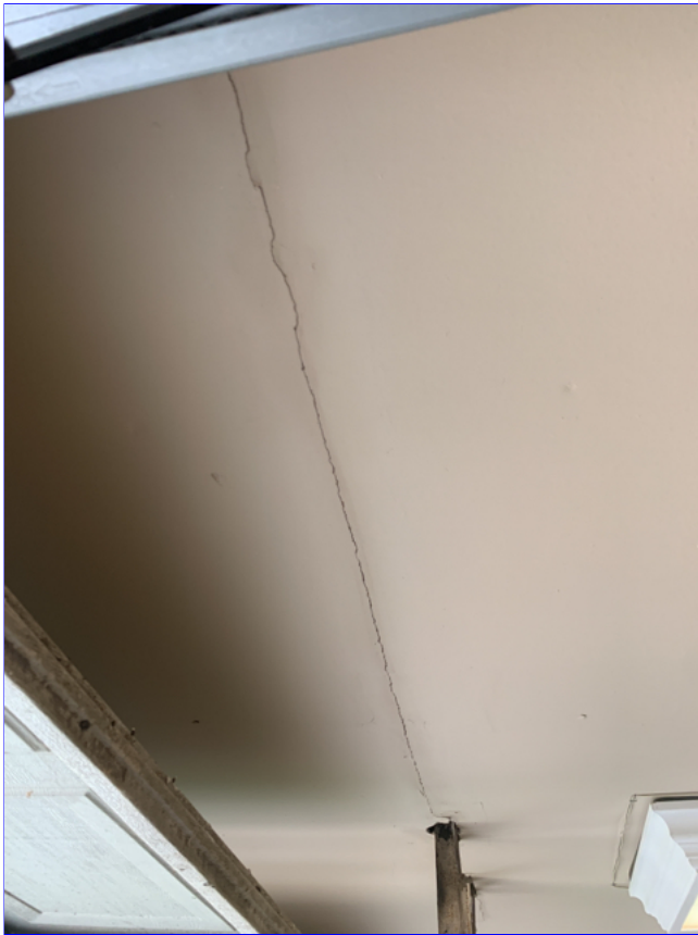
F. Item 1(Picture) Drywall tape joint cracks observed in the garage ceiling. Recommend correction.
