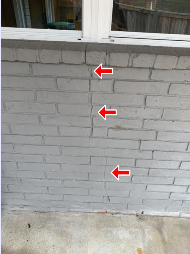
E. Item 5(Picture) Brick veneer mortar cracks were observed.
