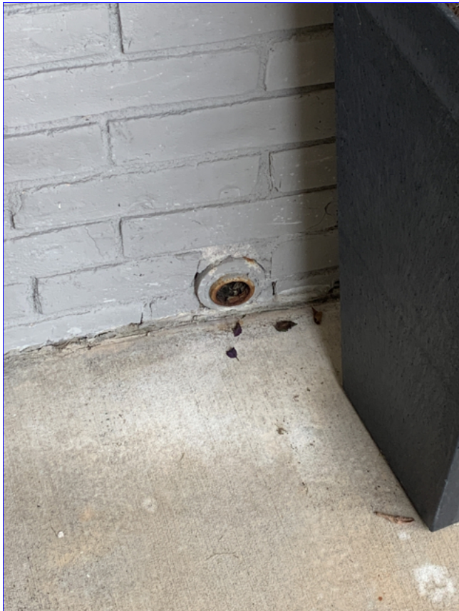
B. Item 1(Picture) Cast iron pipe that is not capped.
