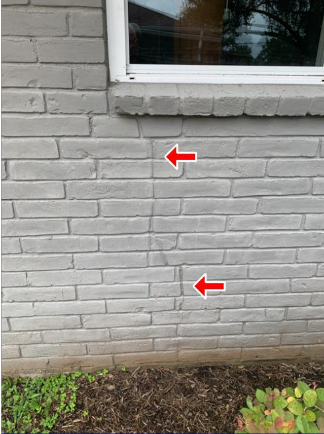
E. Item 6(Picture) Brick veneer mortar cracks were observed.
