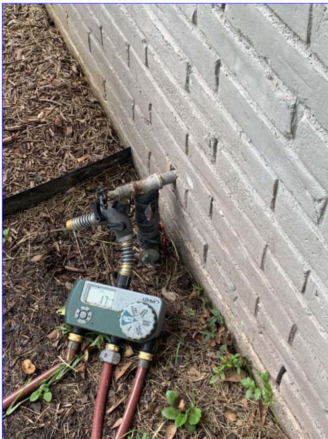
A. Item 1(Picture) The main water supply line at the exterior, is not properly protected from freezing.
