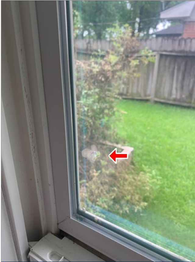
H. Item 4(Picture) There is cracked glass in some windows. Recommend correction.
