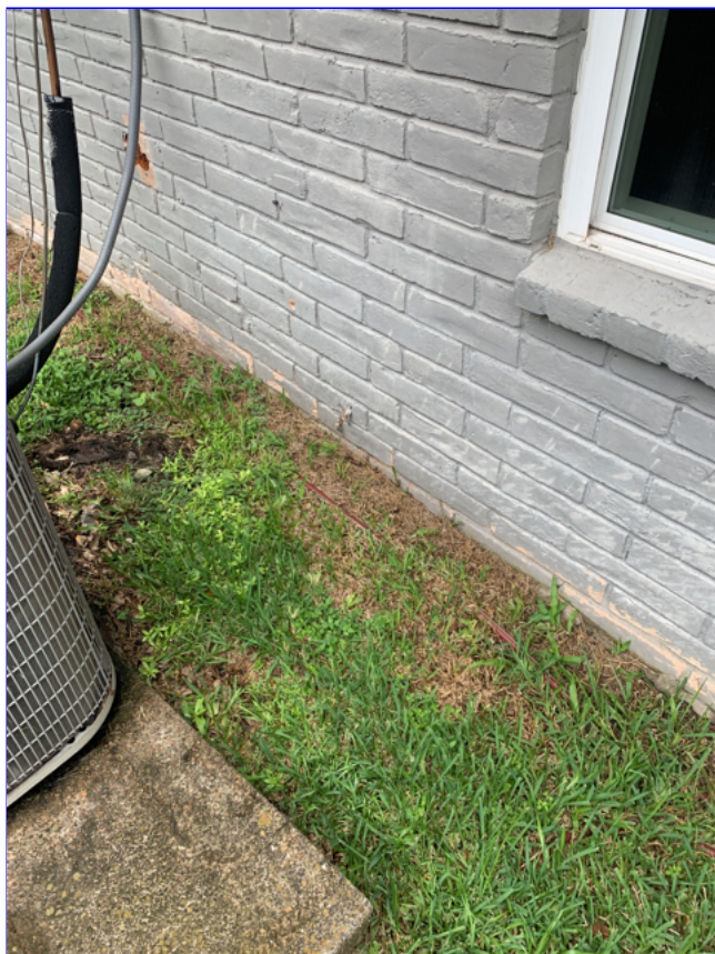
B. Item 1(Picture) High soil conditions observed at front of home left side and right side.
