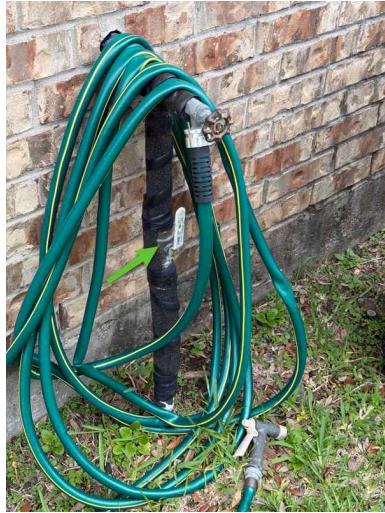
Location of Water Meter: STREET
