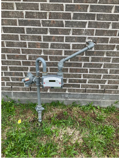
Type of Gas Distribution Piping Material: Black Steel Pipe Comments:
