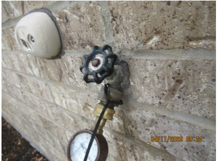
Leaky hose bib
