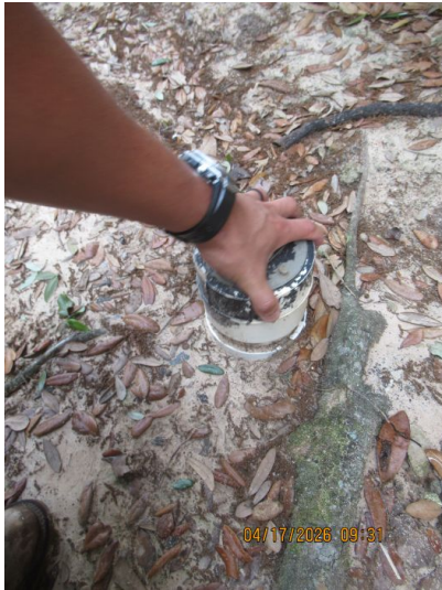
Movement noted in main cleanout - Recommend evaluation by licensed plumber
