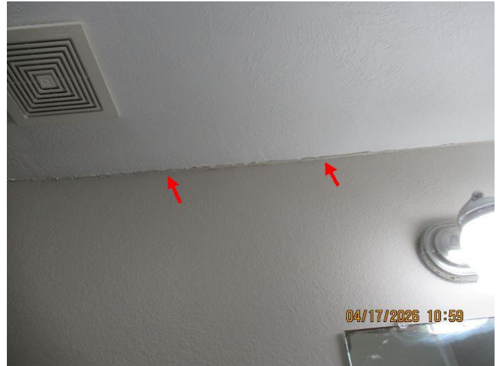
Ceiling cracks were observed
