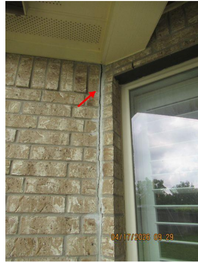
Brick cracks observed.
