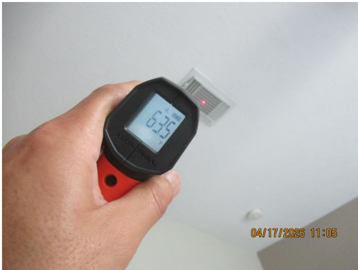
Unit #1 Supply Air Temp
