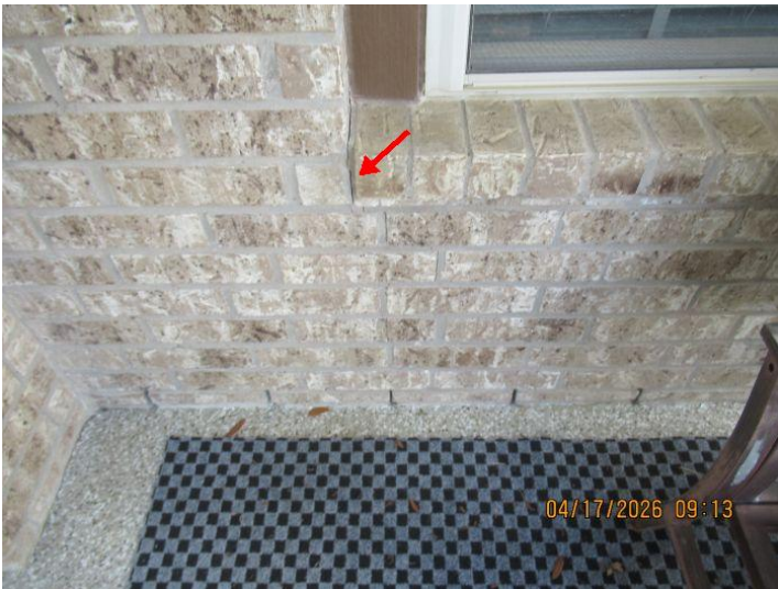
Brick cracks observed.
