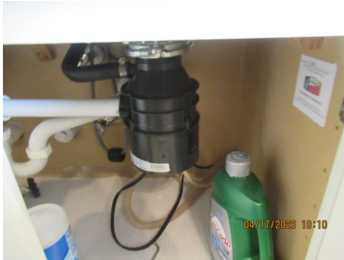
Delay in response for disposal to switch noted.
