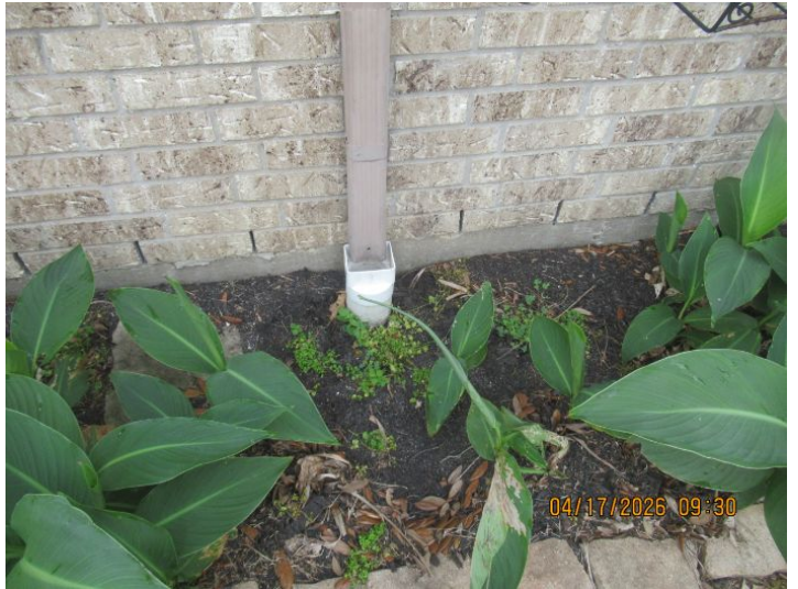
Home displayed signs of gutters terminating in the soil indicating the presence of french drains. Inspecting French drains is not within the scope of standard home inspection because they are typically located underground and not visible. Recommend periodic maintenance/clearing of french drains.
