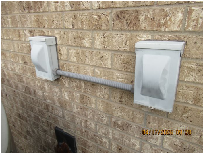
Two disconnects noted with only one A/C - Inquire on reasoning
