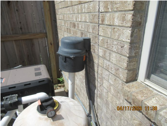
Spa Blower resting on the home.
