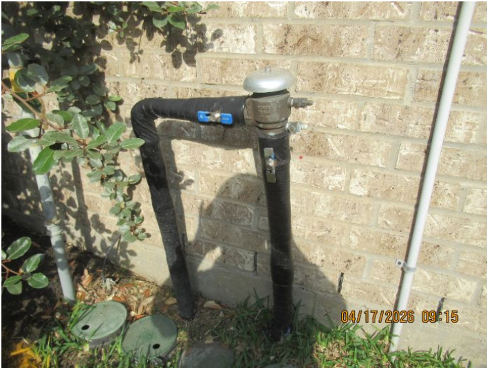
Backflow Preventer Location
