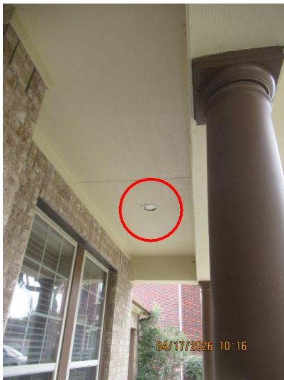
Locations of inoperable bulbs/light fixture. Recommend appropriate correction.
