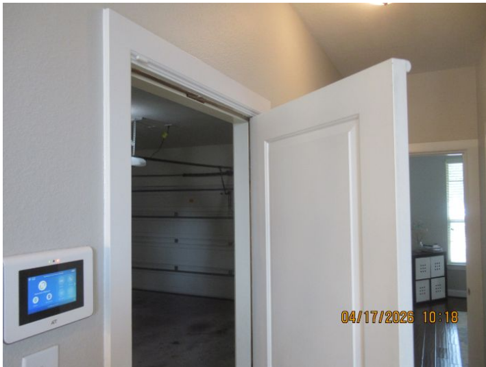
Attached garage doorway is equipped with either missing or non-functioning self-closing hinges. Recommend correction.
