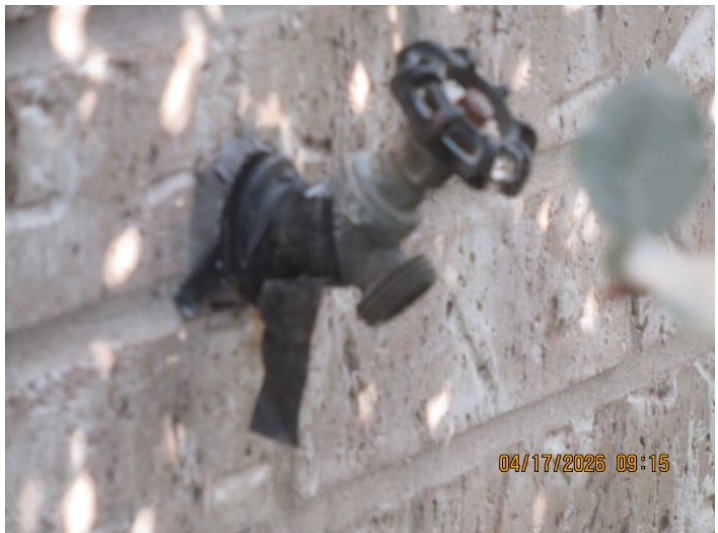
Hose bibs are missing back flow preventers
