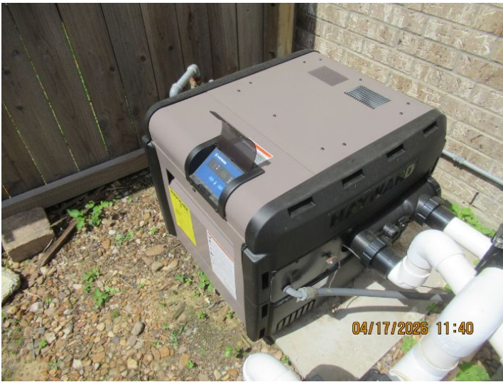
Pool Heater Operational at time of inspection
