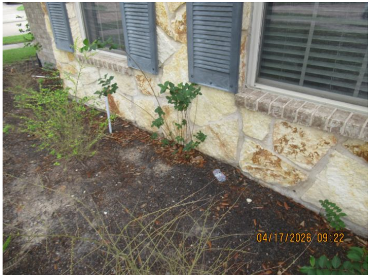
The top of the foundation wall had inadequate clearance from grade. The top of the foundation wall should be a minimum of six inches above soil. Inadequate clearance may result in moisture intrusion of the structure. Excessively high moisture levels can result in damage to the home structure or materials from decay or deterioration and may result in conditions which encourage the growth of microbes such as mold fungi. The Inspector recommends re-grading around the home perimeter to provide increased clearance from grade.
