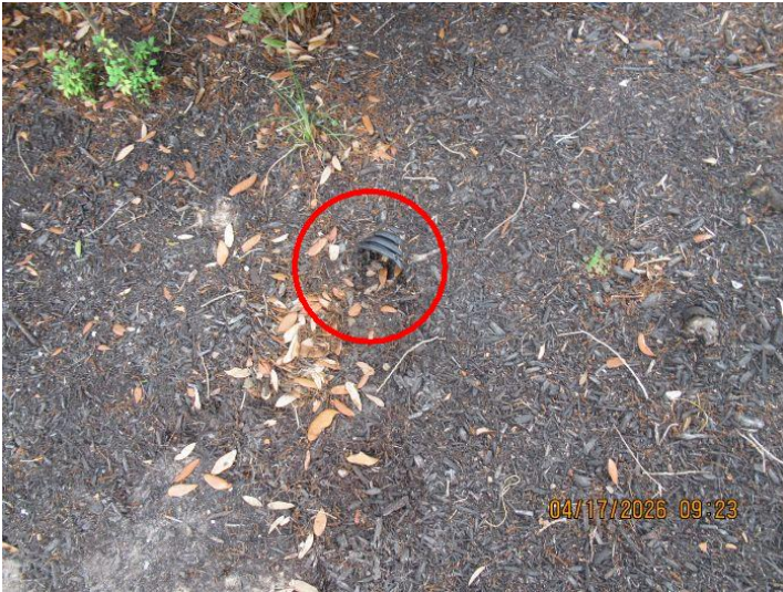
One or more gutter terminations appeared to be blocked. This condition does not allow for proper drainage.
