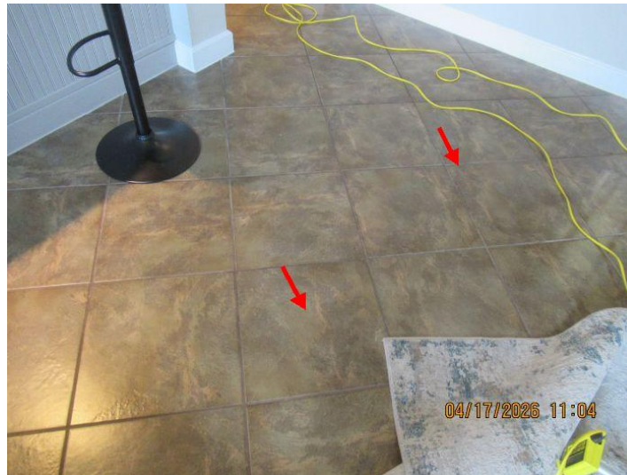
Locations of damaged tiles.
