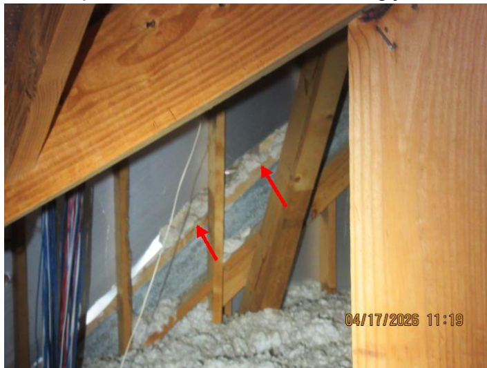
Front - Visible step flashing missing
