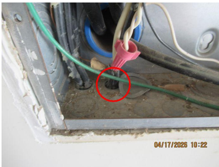
Electrical conductors were not protected from the edges of electrical cabinets, gutters, or cutout boxes
