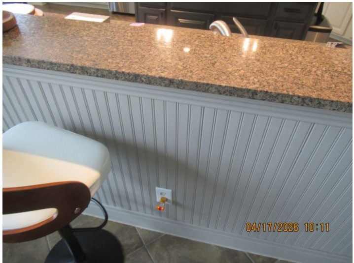
GFCI (Ground fault circuit interrupter) outlets were noted to be missing or did not operate properly in required locations. GFCI outlets should be located in Bathrooms, Garages, Exterior, Crawlspace/Basements, outlets that serve a kitchen countertop, outlets within 6ft of a sink, bathtub, shower. Recommend correction by a licensed electrician. (kitchen)
