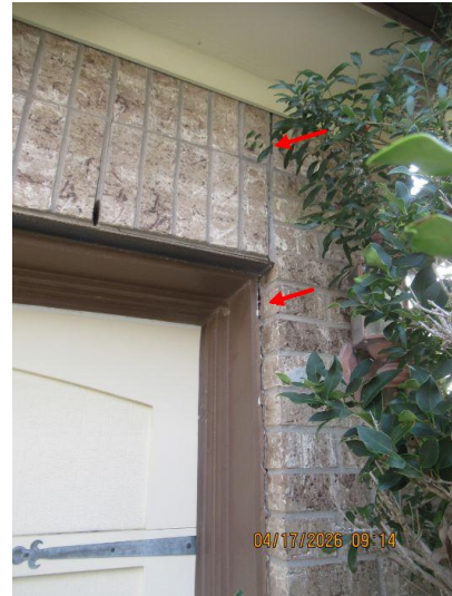
Brick cracks observed.
