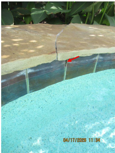
Gap in tile noted - Spa
