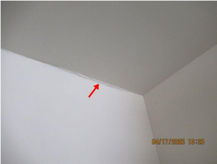
Ceiling cracks were observed (Garage)
