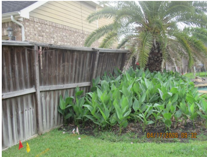
The inspector observed fence work in poor condition or in need or repairs.
