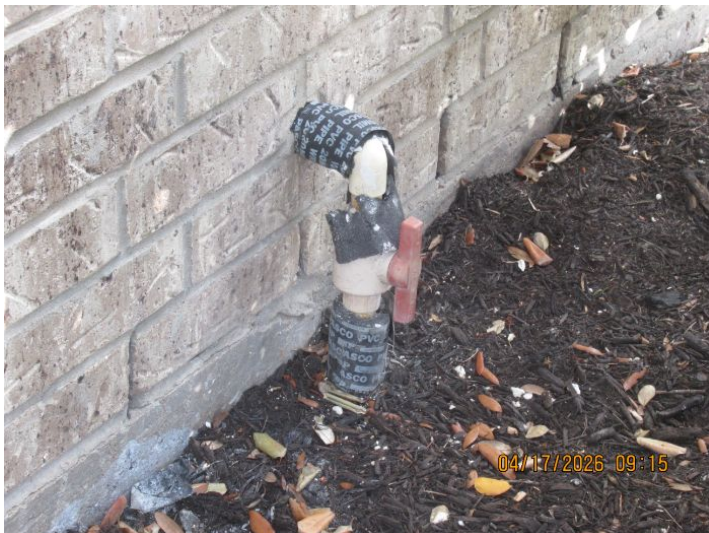
Recommend insulating all exterior piping to protect against the elements
