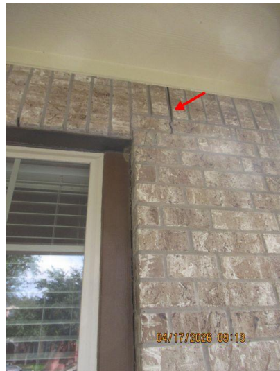
Brick cracks observed.
