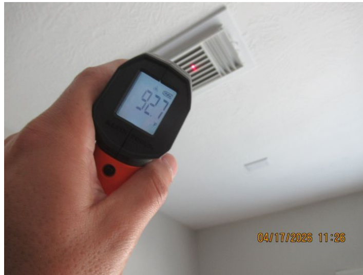
This furnace responded adequately to the call for heat.
