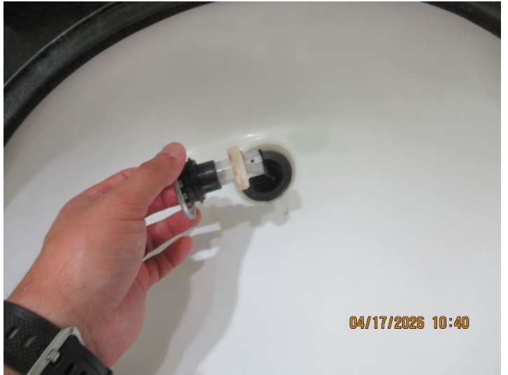
One or more sink drain stoppers did not operate as intended. Recommend correction/repair.
