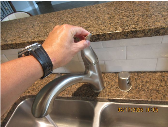
Loose plumbing fixture
