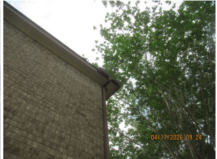
Its was observed that one or more tree branches were either to close or in contact with the roof. Tree branches typically damage shingles when they come in contact with them reducing the life of the shingle. It is recommended to trim the branches back and contact a reputable roofing contractor to replace/repair and damaged shingles.
