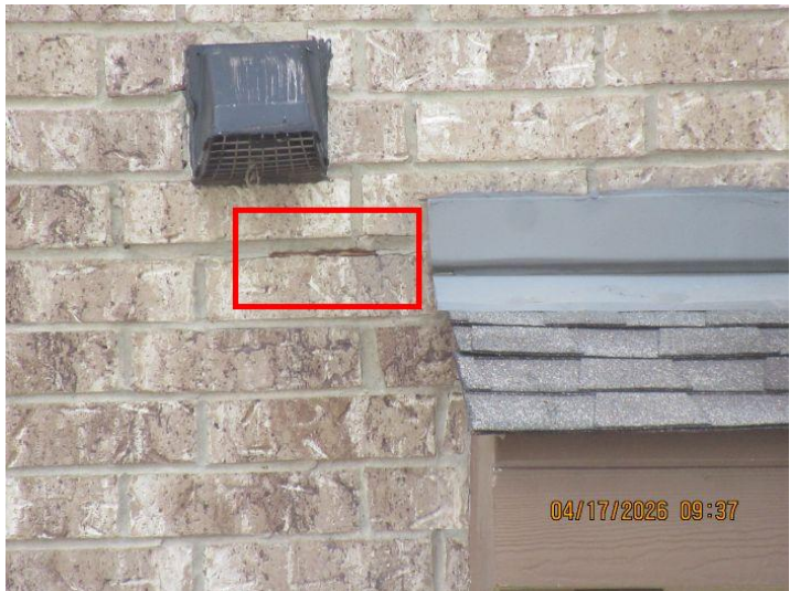
Steel lintel were observed to be exposed and not embedded in the mortar. This causes the lintel to rust and can cause the mortar to crack.
