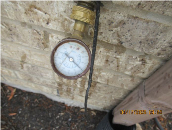
Static Water Pressure Reading: 60psi
