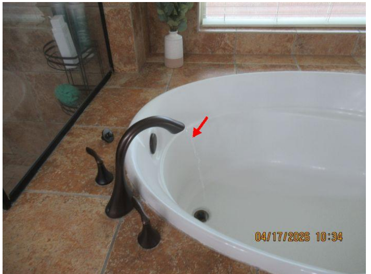
Inspector noted plumbing fixture with low pressure. Recommend further evaluation/correction.
