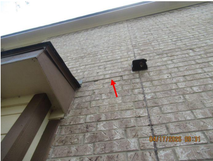
Brick cracks observed.
