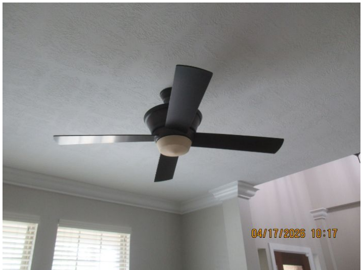
No remote present for front ceiling fan
