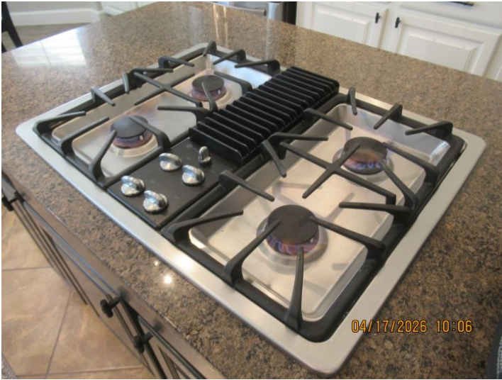
All stove top gas burners operated when tested - Improper flame color noted.
