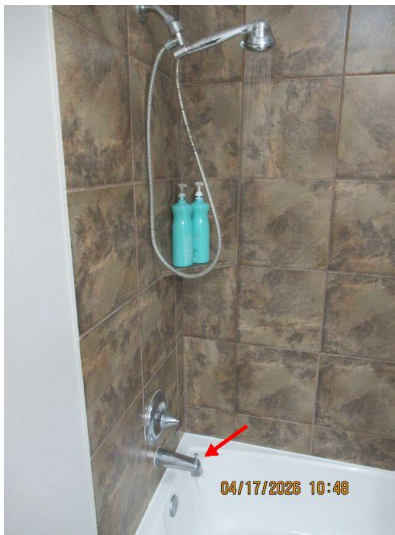
Tub fixture diverter handle did not operate properly
