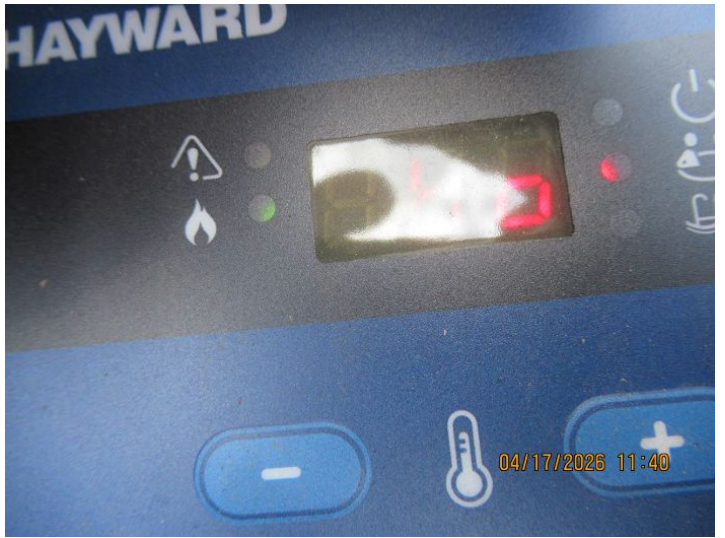
Pool Heater Operational at time of inspection
