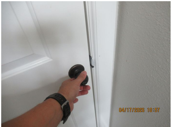
Inspector noted one or more interior doors that do not latch properly in strike plate.
