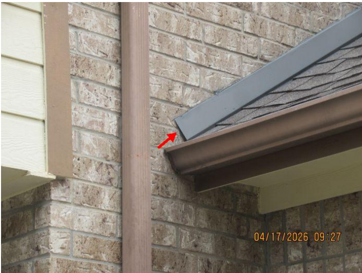
The home had no kick-out flashing installed or missing in appropriate locations. Kick-out flashing is designed and installed to divert water from behind the exterior wall covering at areas of the home where a sidewall extends out past a connecting roof eave. This condition may allow moisture intrusion of the exterior wall covering.
