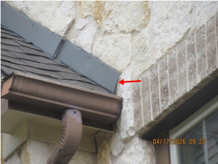
The home had no kick-out flashing installed or missing in appropriate locations. Kick-out flashing is designed and installed to divert water from behind the exterior wall covering at areas of the home where a sidewall extends out past a connecting roof eave. This condition may allow moisture intrusion of the exterior wall covering.
