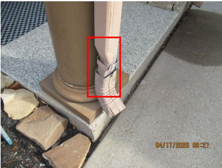
One or more locations at gutter downspouts showed signs of damaged.
