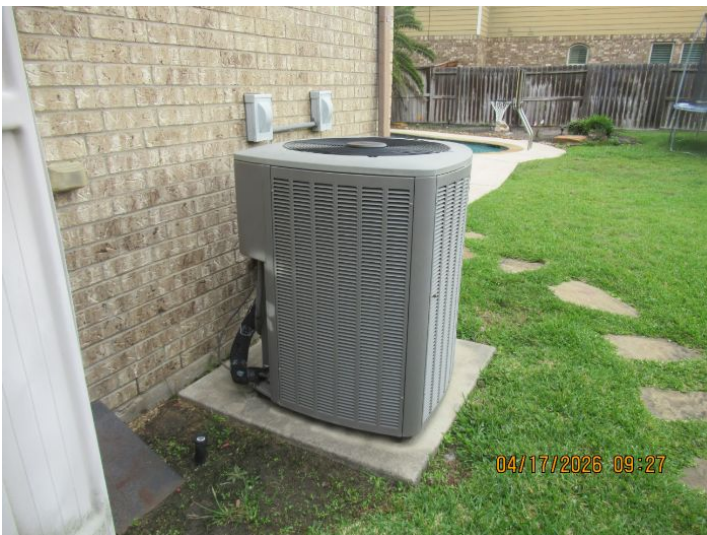
Exterior Compressor/Condensing Unit(s)
