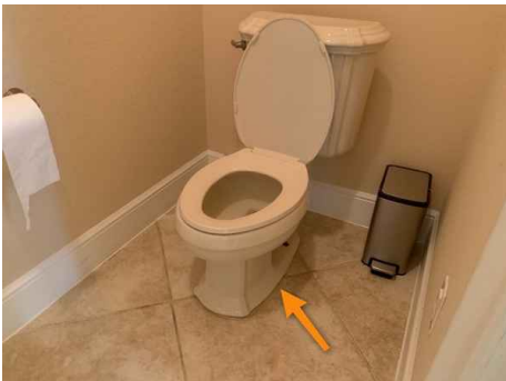
Example Primary Bathroom
