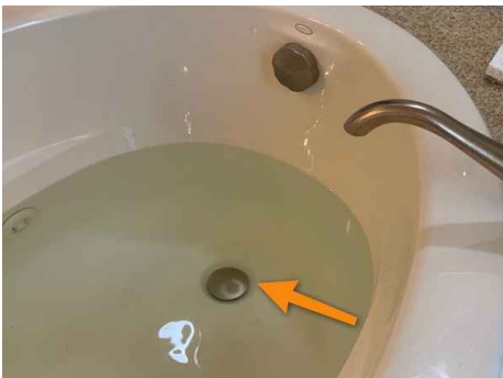
Example Primary Bathroom
