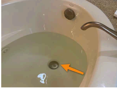
Example Primary Bathroom
