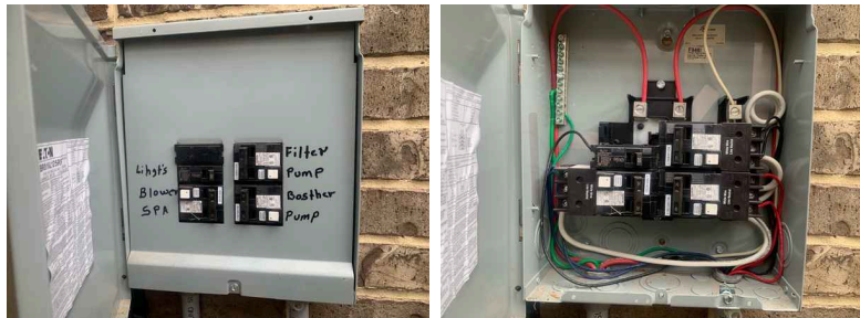
Location of Main Panel: Right exterior
