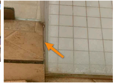
Example Primary Bathroom
