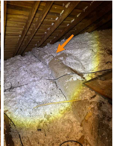
Ducts buried/not supported
