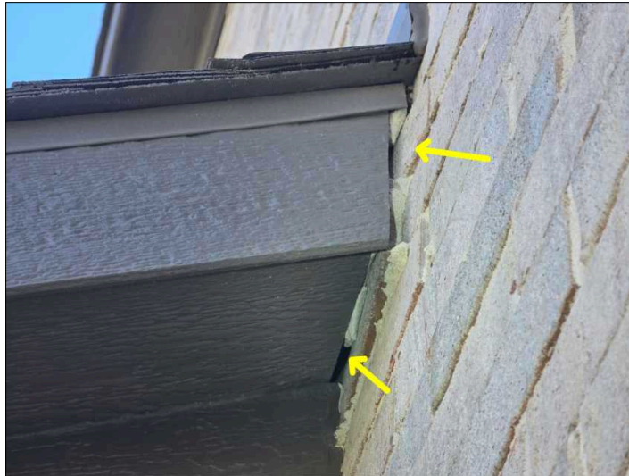
Open holes around porch large enough for pest entry.
