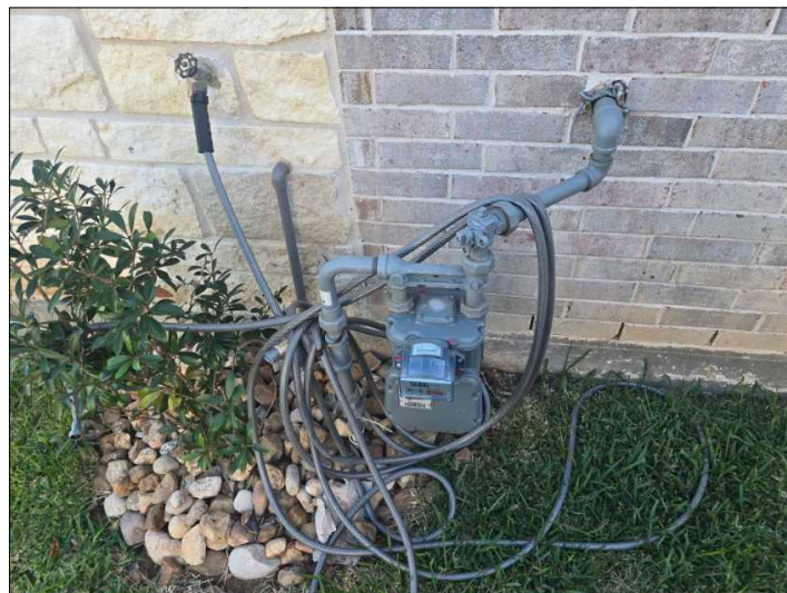
Gas Meter and Shutoff Location.
