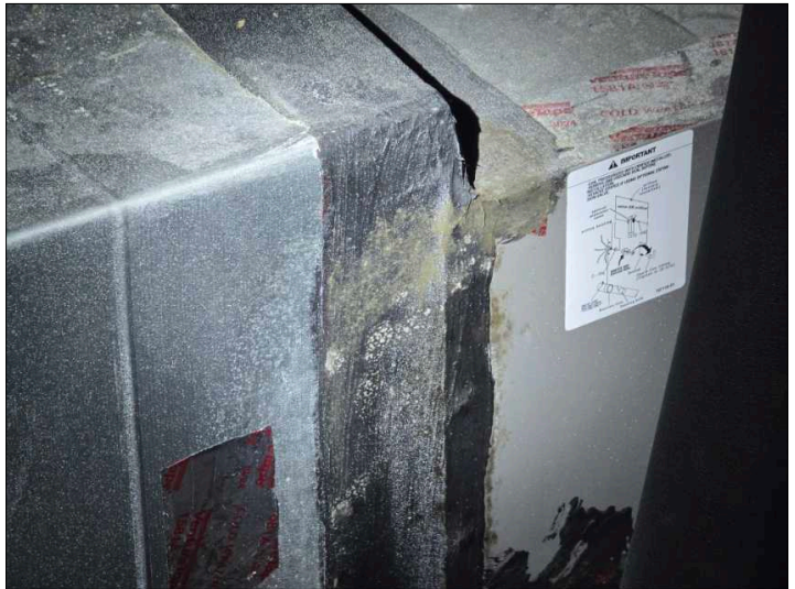
Microbial growth found on outside of HVAC unit. Likely caused by air leakage.
