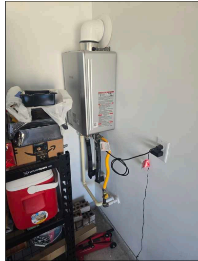
Drip pan missing from under unit. Pan and drain should be installed when house damage can occur from a leaking water heater.
