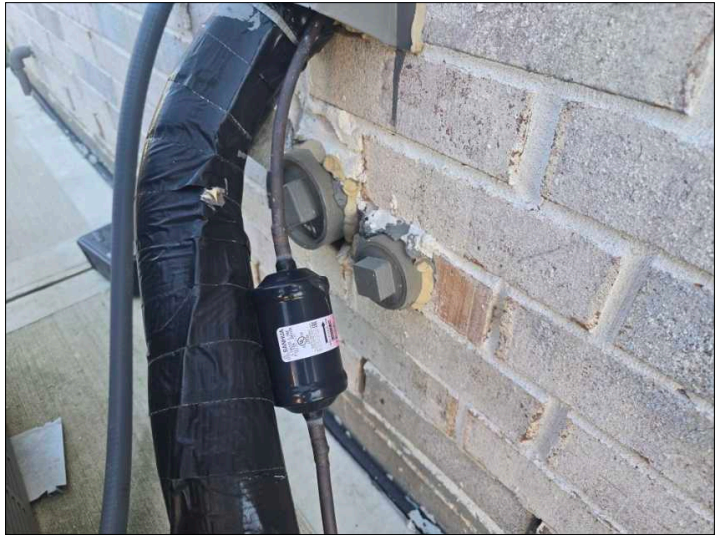
Poorly placed plumbing cleanouts.
