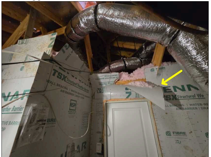
Insulation holding panel loose.
