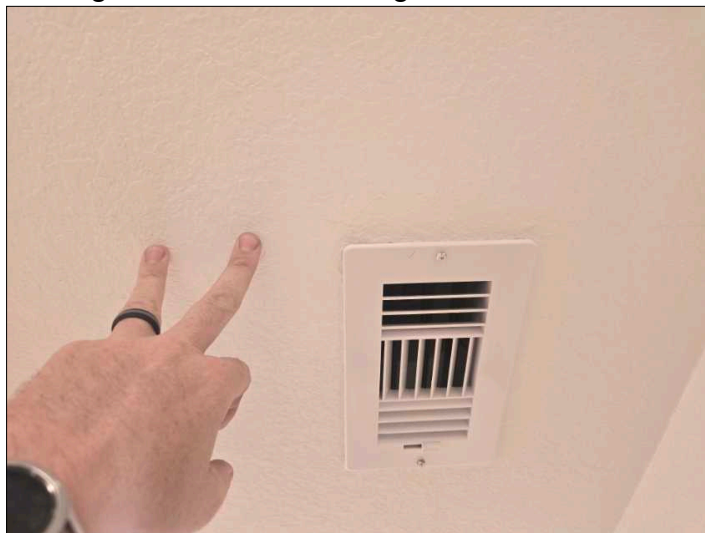
Minor ceiling crack noted near register in master bathroom.
