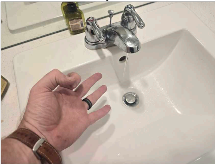
Master bath faucet has reduced flow. Repairs needed for blockage / internal damage.
