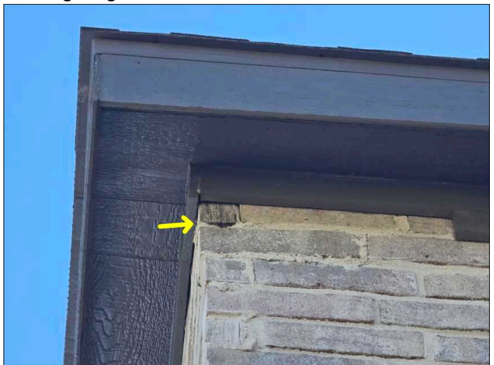
Loose brick found at top corner near garage.
