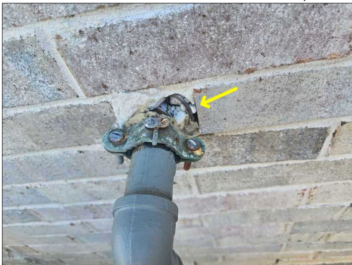
Open hole in brick around gas line.
