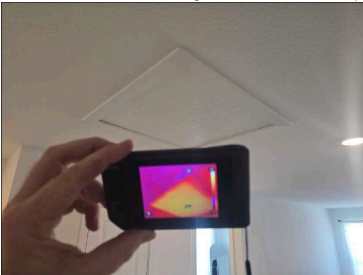
Missing insulation at access panel. Suggest batt insulation stapled to backside.
