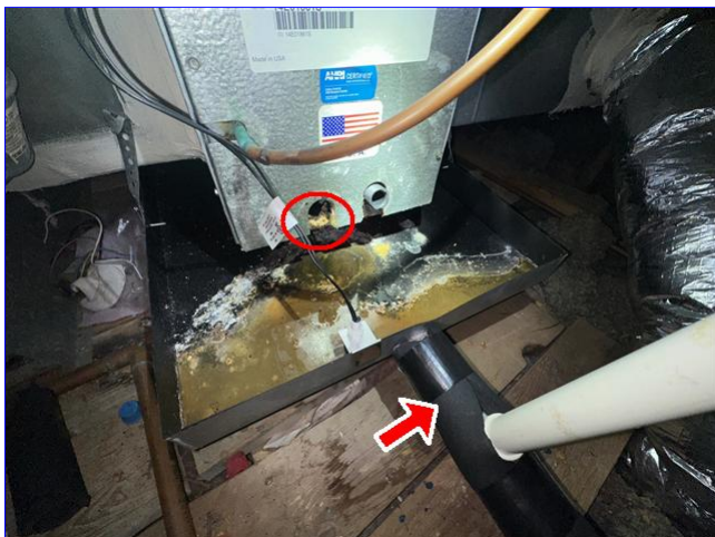
B. Item 1(Picture) Primary condensate draining into the pan, pan drain carries water to exterior
