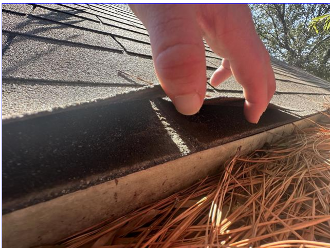
C. Item 17(Picture) left side
