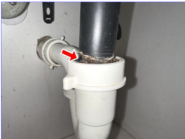
B. Item 1(Picture) very small leak
