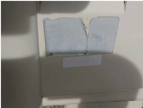
The heater data plate was not legible at the time of the inspection.
