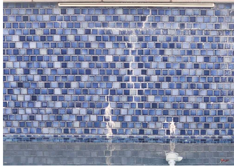
Calcium buildup observed on the tiles.
