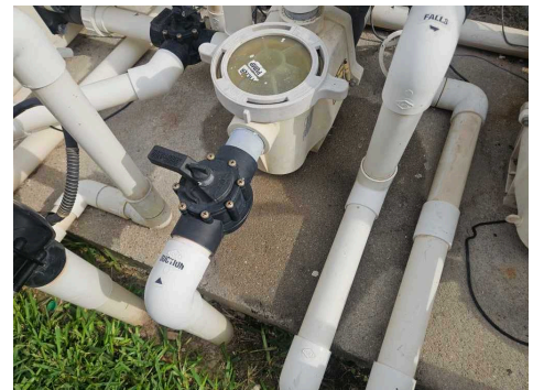
The pool equipment pad was wet underneath the water feature pump at the time of the inspection.
