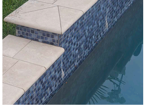
Calcium buildup observed on the tiles.
