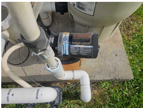
The pool cleaner booster pump was noisy at the time of the inspection.
