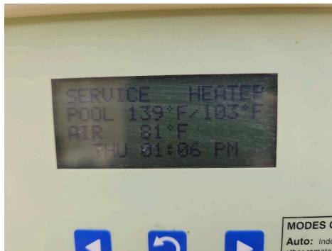
The pool heater is not responding to any of the control panel commands.
