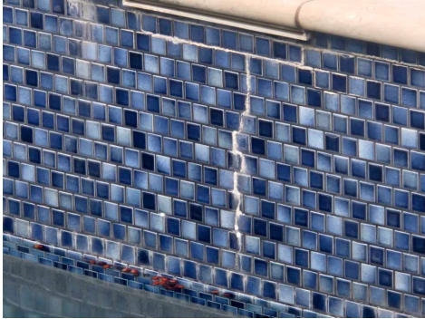
Calcium buildup observed on the tiles.
