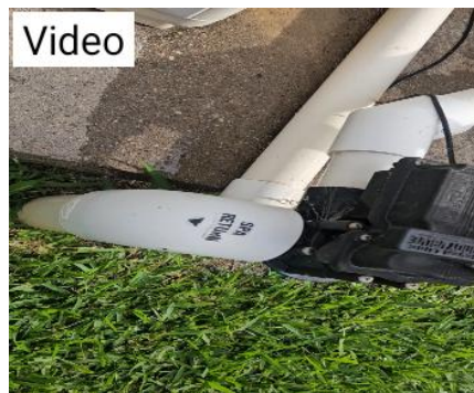
The spa valve was leaking at the time of the inspection.
