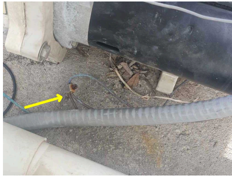
The pool filter motor was not bonded at the time of the inspection period
