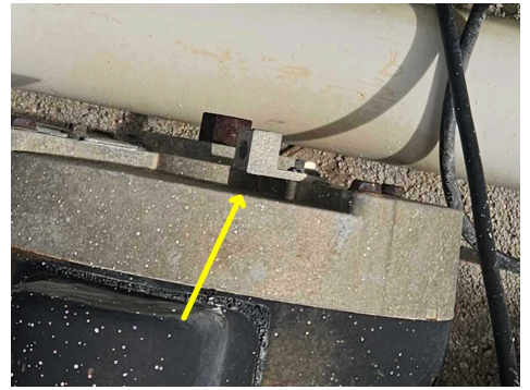
The water feature motor was not bonded at the time of the inspection.
