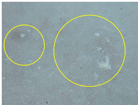
Excessive wear and tear observed on the pool finish.
