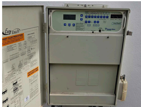
The pool equipment control panel.
