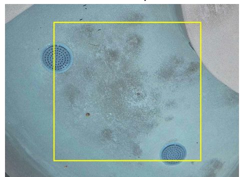
Excessive wear and tear observed on the spa finish.
