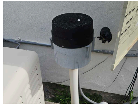
The spa blower did not respond to commands from the control panel.
