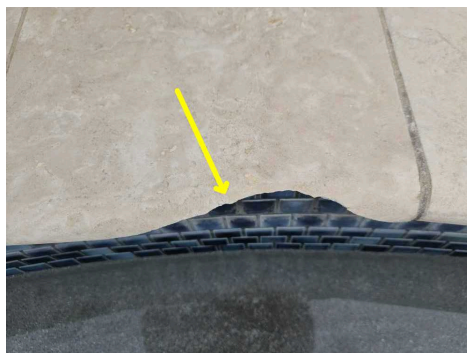
The coping was damaged near the stairs.
