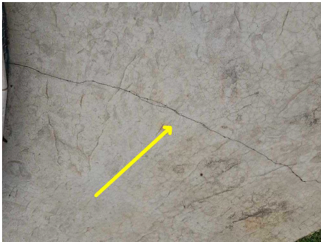
Cracks for observed in the pool deck.
