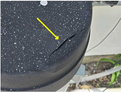
The spa housing was cracked at the time of the inspection.
