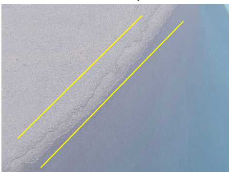
Excessive wear and tear observed on the pool finish.
