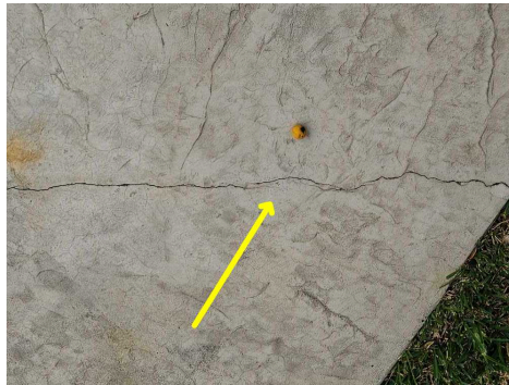
Cracks were observed in the pool deck.
