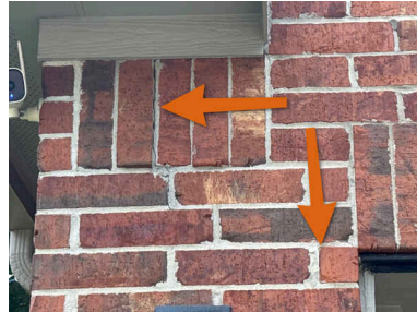
Mortar joint crack
