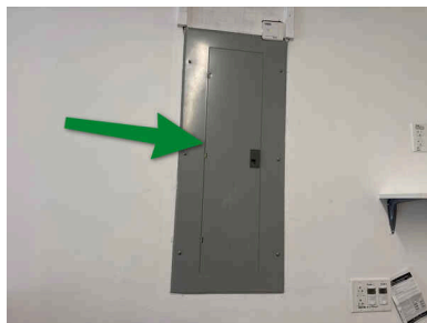
Electrical service panel
