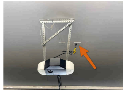
Missing GFCI protection
