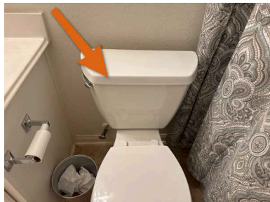
Loose water tank
