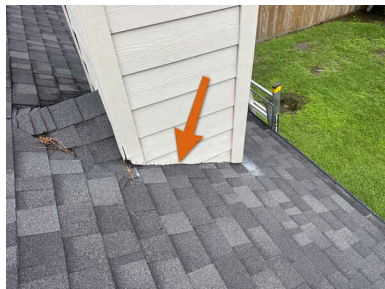
Minor siding deterioration at roof
