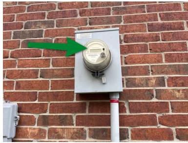
Electrical service entrance
