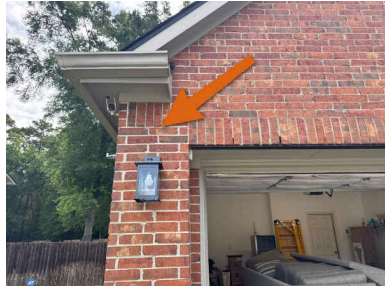
Mortar joint crack
