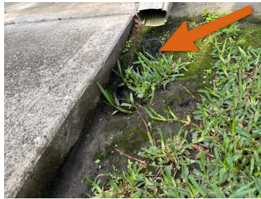
Discharges to foundation
