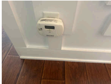
(CO) alarm outside secondary bedrooms
