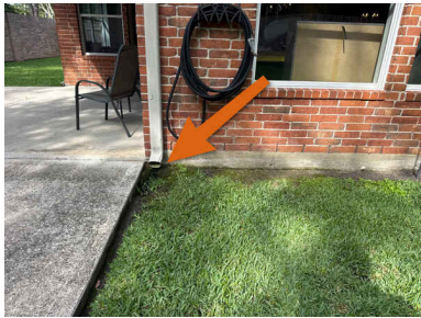
Discharges to foundation
