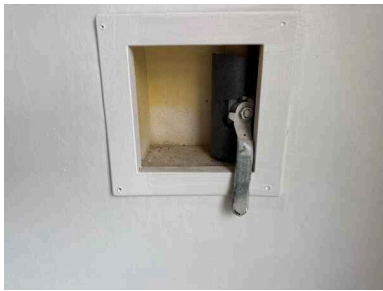
Main water supply valve
