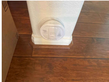
(CO) alarm outside master bedroom
