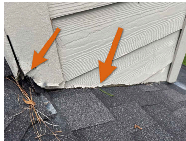
Minor siding deterioration at roof
