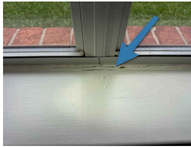
Localized finish damage at windowsill
