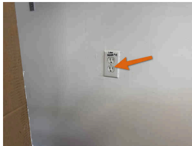
Missing GFCI protection
