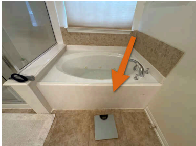
Missing pump access
