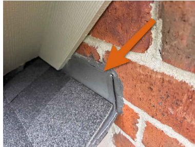
Gaps at wall
