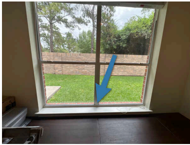
Localized finish damage at windowsill
