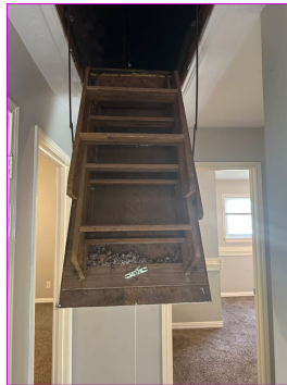
The attic access hatch cover was not insulated.
