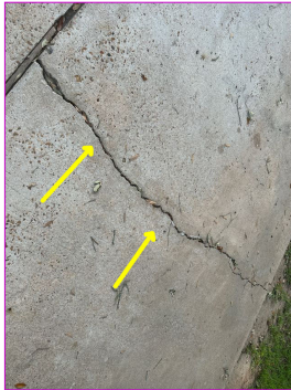
Common cracks (1/4-inch or less) were visible in the driveway. Cracks exceeding 1/4-inch should be filled with an appropriate material to avoid continued damage.
