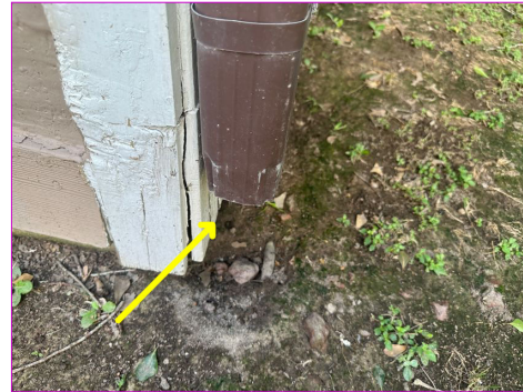
One or more downspouts discharged roof drainage next to the foundation. This condition can effect the ability of the soil to support the weight of the structure above and can cause damage related to soil/foundation movement. The Inspector recommends the installation of downspout extensions to discharge roof drainage a minimum of 6 feet from the foundation.
