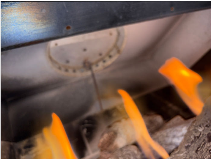
Artificial gas logs were present within the firebox and the damper is required to be permanently blocked in the open position so as to prohibit any accidental spillage of carbon monoxide into the living space.
