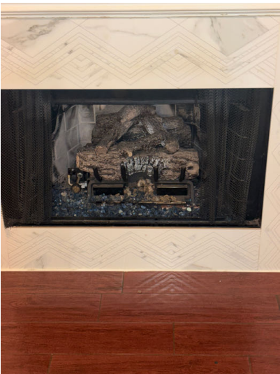
Artificial gas logs were present within the firebox and the damper is required to be permanently blocked in the open position so as to prohibit any accidental spillage of carbon monoxide into the living space.
