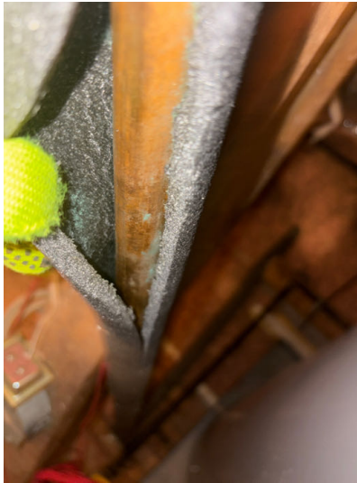
Type of Supply Piping Material: COPPER
