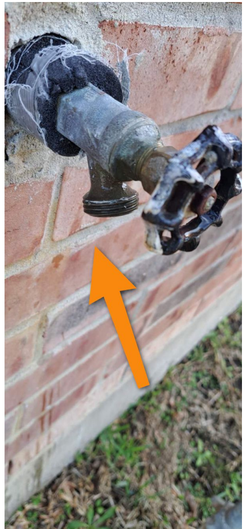
Right exterior faucet
