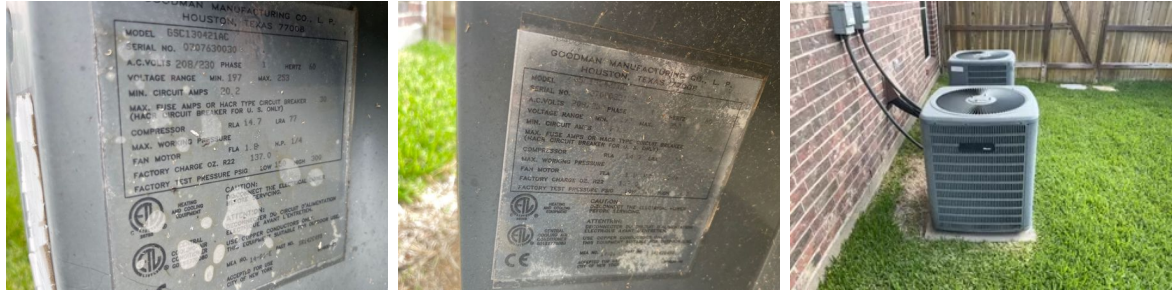
Photos - Temperature Differential Return & Supply Sample Images: upper level, 16
