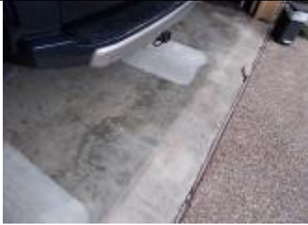
Previous Repairs to Foundation
