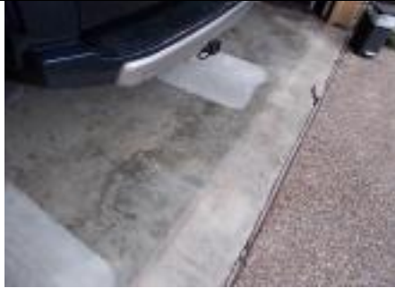
Previous Repairs to Foundation
