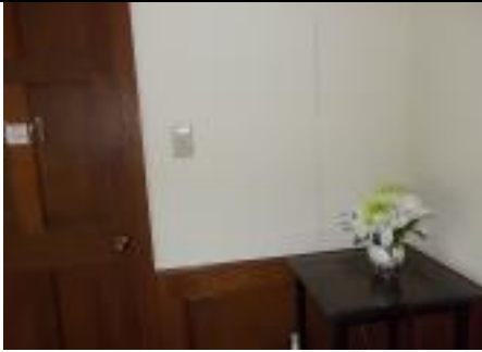
Moisture Damage to Wall Paneling
