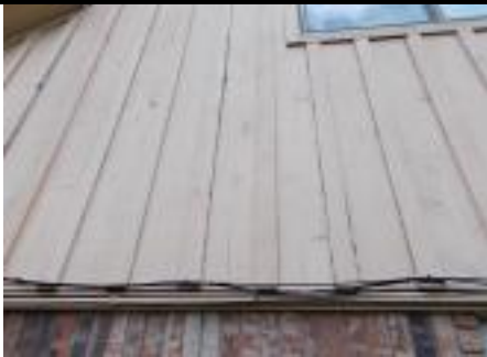
Cracked Wood Siding
