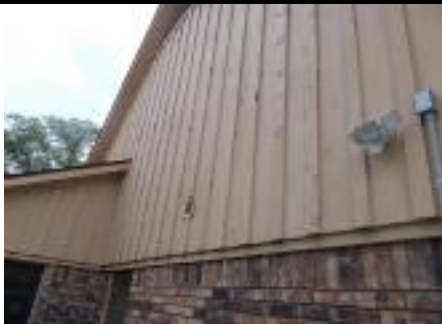
Cracked Wood Siding
