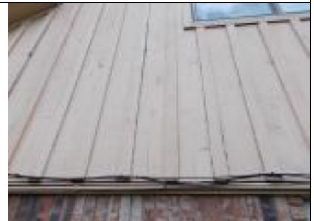
Cracked Wood Siding
