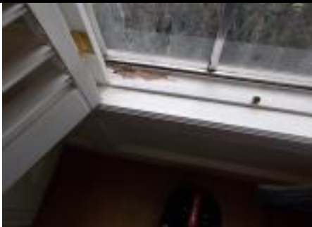
Damaged Window Sill
