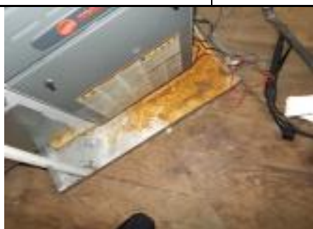
Rust in Condensate Pan
