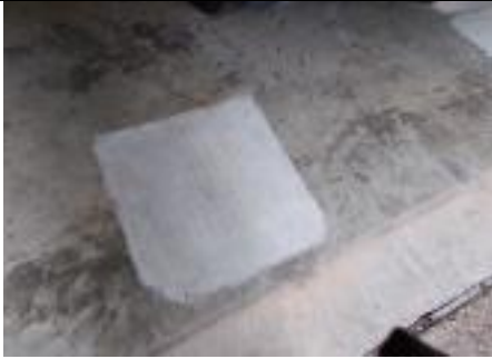
Previous Repairs to Foundation
