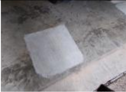
Previous Repairs to Foundation
