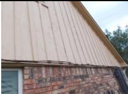
Cracked Wood Siding
