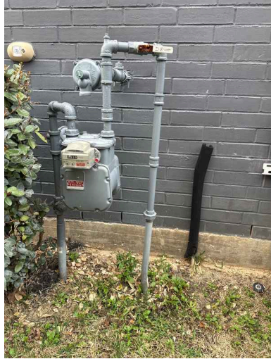
Location of Gas Meter: Exterior Gas Piping Material: Cast Iron
