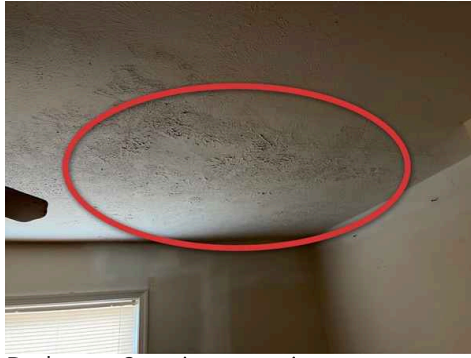
Bedroom 2 moisture stain
