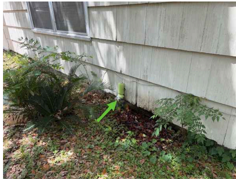
Main shut off the location
