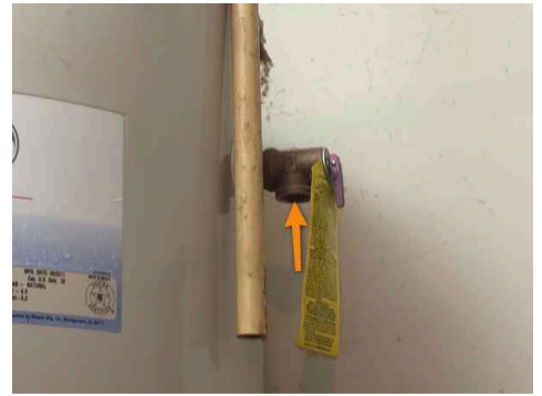
Missing discharge pipe
