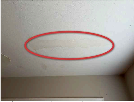
Bedroom 1 moisture stain
