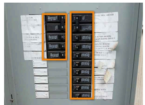
No afci breakers
