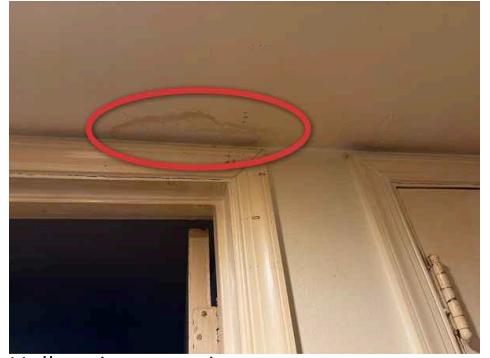
Hall moisture stain
