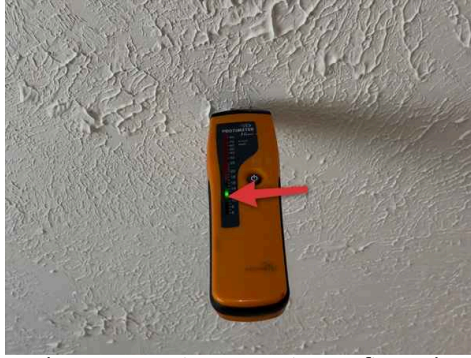
Bedroom 2 moisture stain confirmed dry
