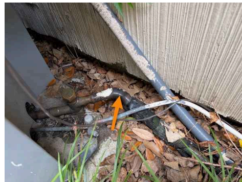
Damage refrigerant line insulation
