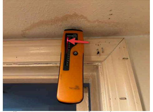
Hall moisture stain confirmed wet
