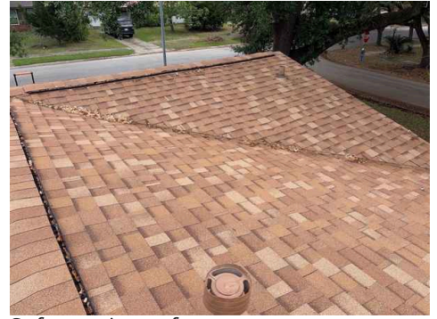
Soft spot in roof
