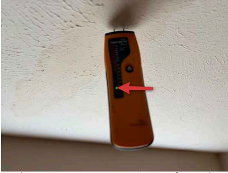
Bedroom 1 moisture stain confirmed dry
