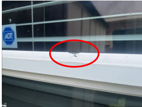
Left: Damaged weatherstripping
