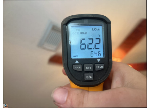
Bedroom 3 vent temperature
