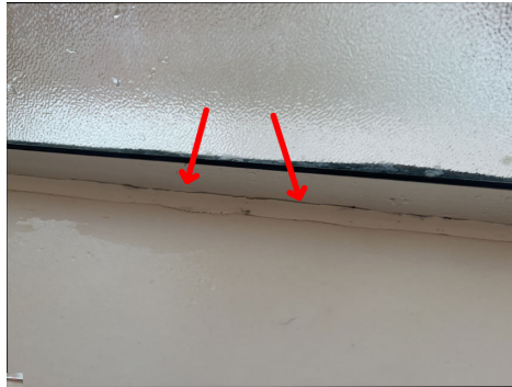
Bathroom 2: Deteriorated caulk
