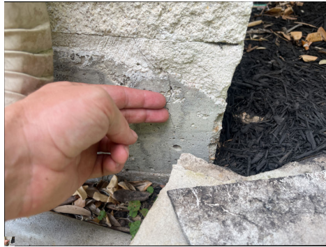
Left front: Corner crack
