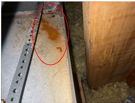
Rust in safety pan
