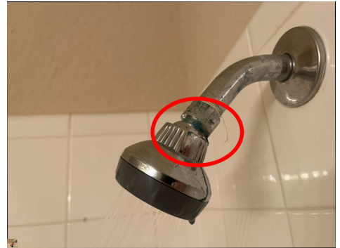
Bathroom 1: Leak at shower head
