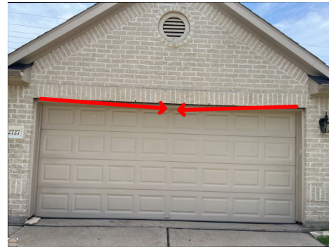
Front: Sagging header
