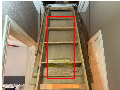
Pull-down stairs lacked insulation
