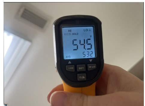
Primary suite vent temperature
