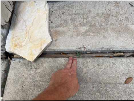
Driveway/walk to foundation: Remove wood boards, Monitor area for insect activity
