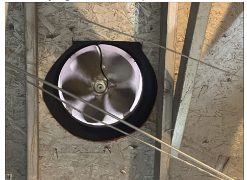
Power ventilator on
