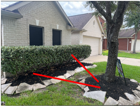
Front: Tree roots adjacent to foundation
