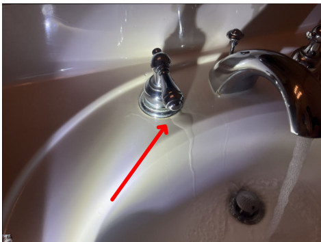
Bathroom 2: Leak at control
