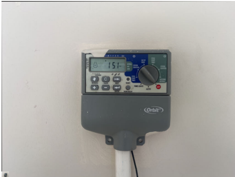
Garage: Controls to sprinkler system
