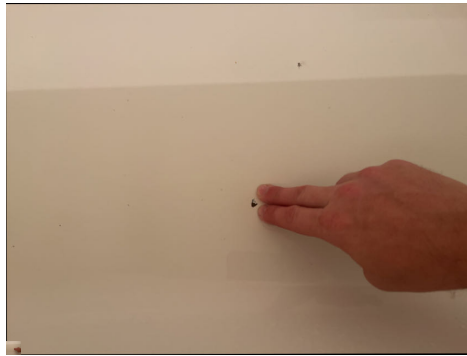
Bathroom 1: Tub damage
