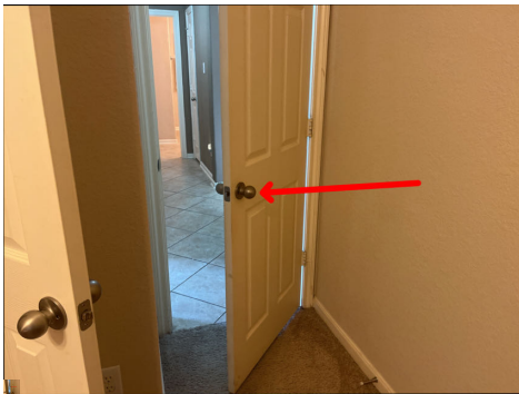
Bedroom 1: Out of plumb
