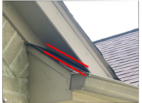
Front: Gaps at soffit/shingles
