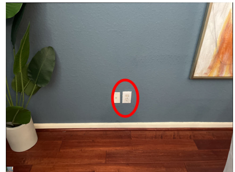
Living room: Loose outlet
