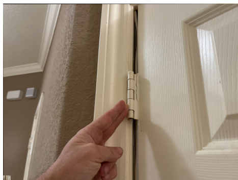
Garage man door: Auto-close device recommended
