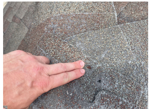
Exposed nail heads
