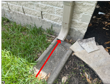
Downspout extension missing, discharge near structure
