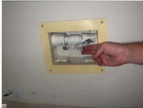
Garage: Main Water Shutoff Valve
