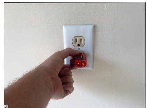
Garage: Outlet not GFCI protected
