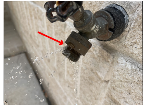
Front: Faulty backflow preventer
