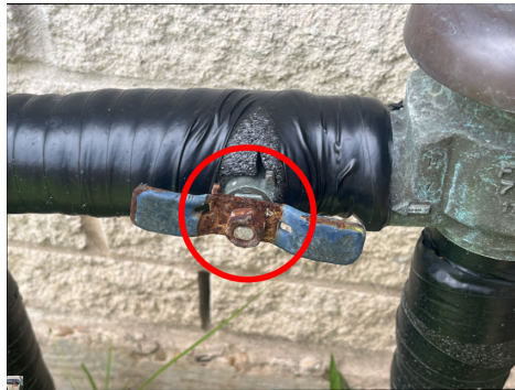
Backflow preventer: Corroded valve control
