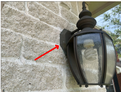
Around House: Caulk missing at fixture to wall connection
