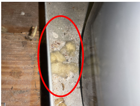
Debris in safety pan
