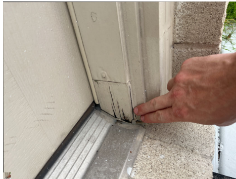
Back door: Wood decay at trim
