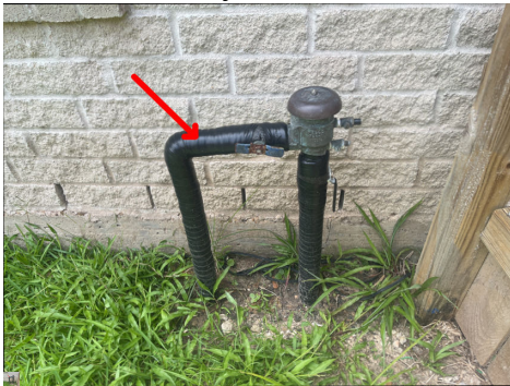
Left: Backflow preventer
