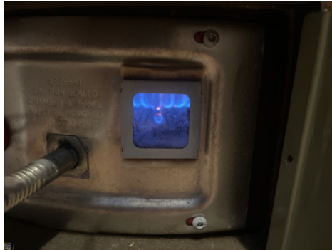
Water heater fired up
