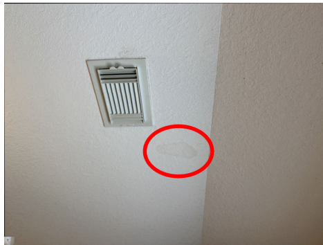
Dining room: Moisture stain
