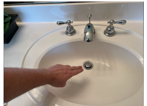
Bathroom 2: Drain stops did not retain water.
