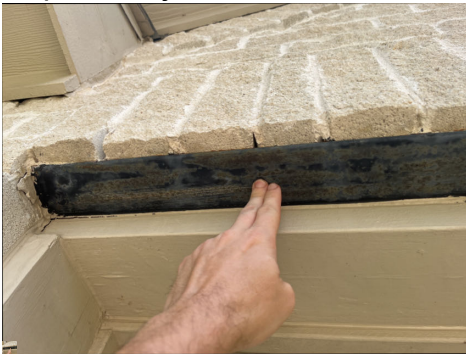
Front: Rust at lintels
