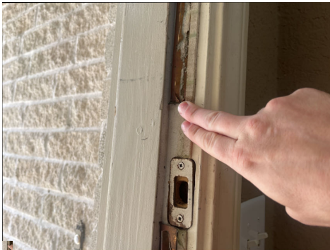
Front door: Damaged weatherstripping
