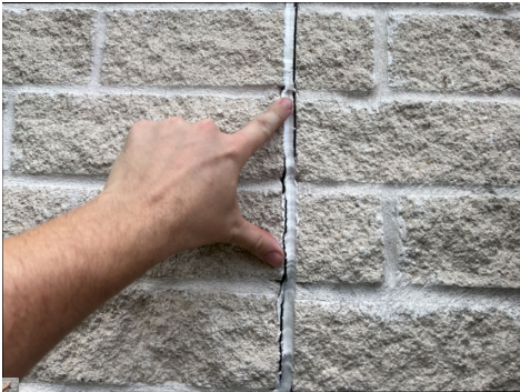
Right: Deteriorated caulk at expansion joint
