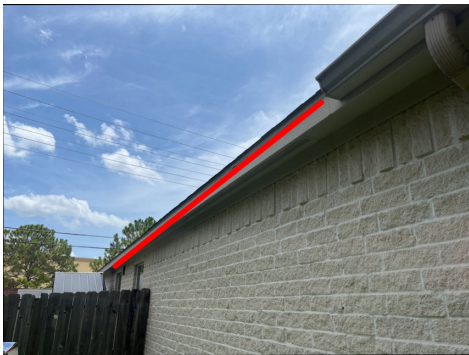
Incomplete gutter system
