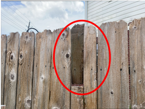
Fence: Damaged picket
