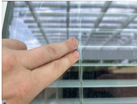
Living room: Evidence of lost seal
