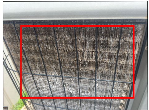
Damaged/deteriorated coil fins
