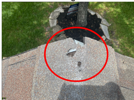
Left front: Damaged shingles with exposed roof deck/structure
