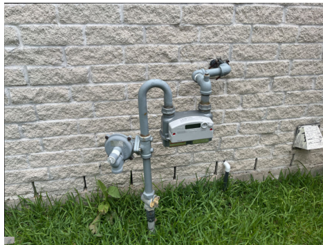
Right: Gas meter
