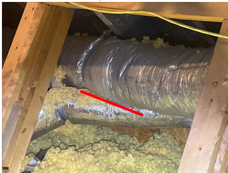
Ducts in contact
