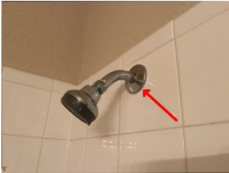
Bathrooms: Caulk needed at shower wall protrusions
