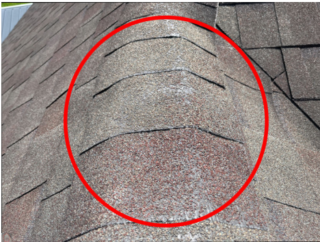
Granule loss/deterioration at ridge shingles
