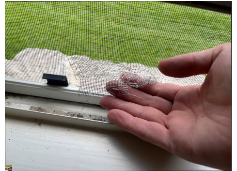
Dining room: Damaged screen
