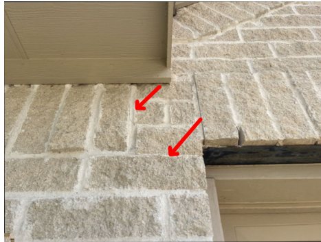
Front: Hairline cracks
