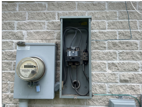
Right: Service panel with deadfront removed
