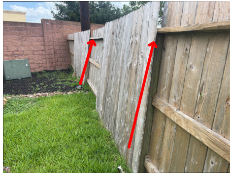
Fence: Tilted posts
