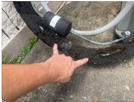
Old and deteriorated refrigerant line insulation
