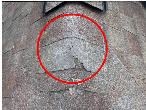
Top ridge: Damaged/deteriorated shingle
