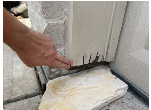
Garage: Wood decay at trim
