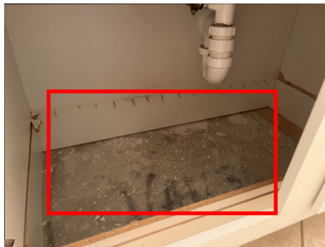
Bathroom 1: Missing/damaged cabinet floor
