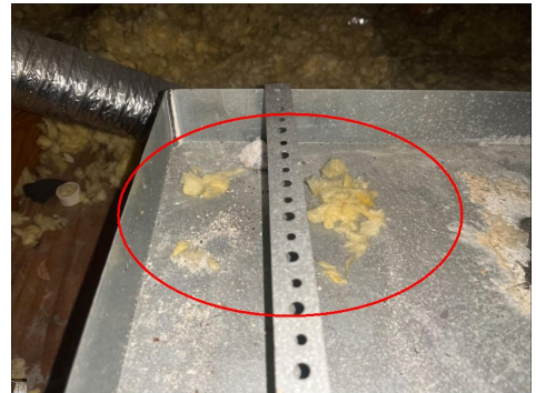
Debris in safety pan
