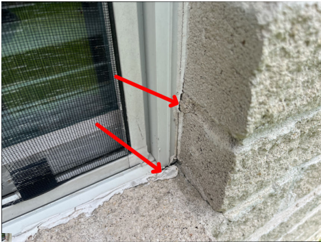
Around house: Deteriorated caulk
