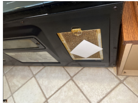
Range hood on, dirty filter
