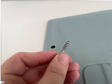
Sub panel: Improper deadfront screws
