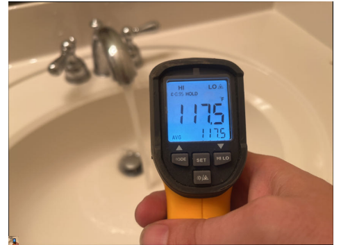
Hot water temperature
