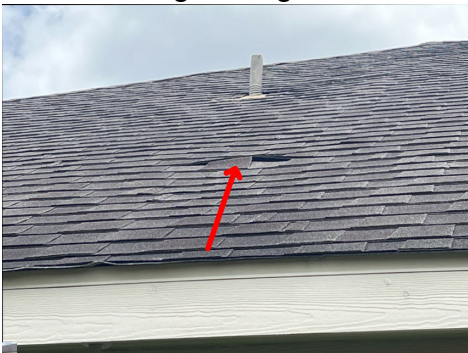
Right: Uplifted shingle
