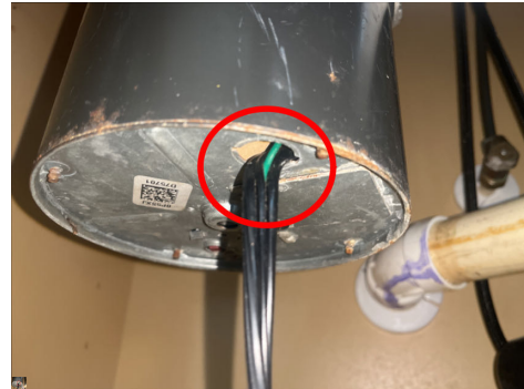
Wire clamp missing
