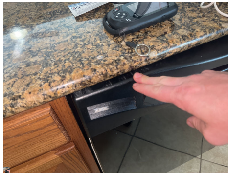
Insufficient clearance at counter/door
