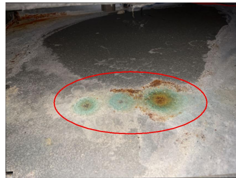
Evidence of coolant leak
