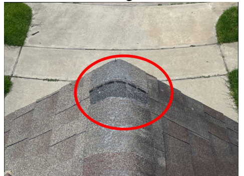
Right front ridge: Torn/damaged shingle
