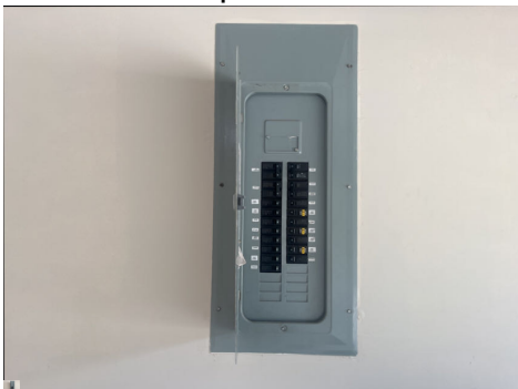
Garage: Cutler-Hammer sub panel
