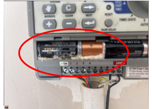
Controls: Corrosion at batteries
