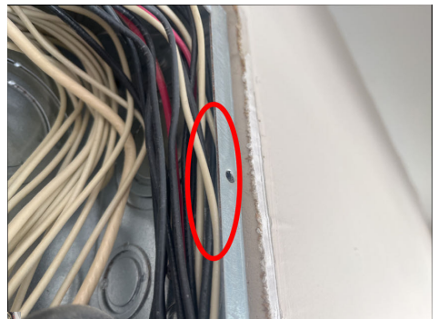
Sub panel: Missing spacer
