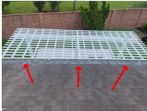
Rear: Evidence of prior repair
