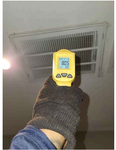
Garage apartment Return Vent
