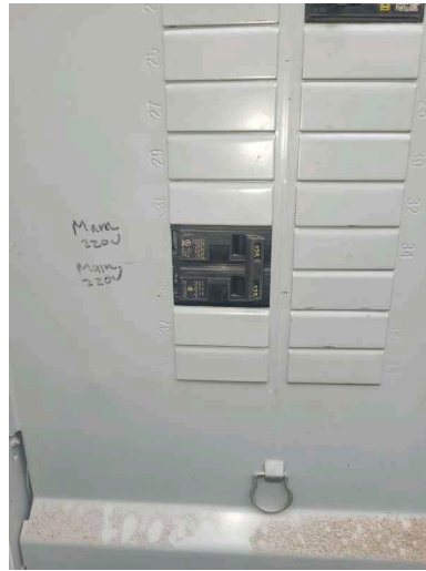
Siemens Panel 125 AMP service[garage apartment)
