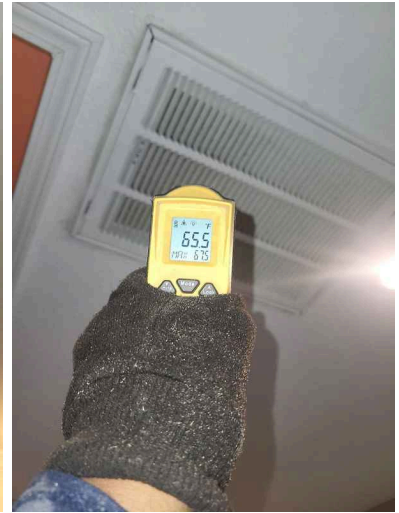
Garage apartment Return Vent
