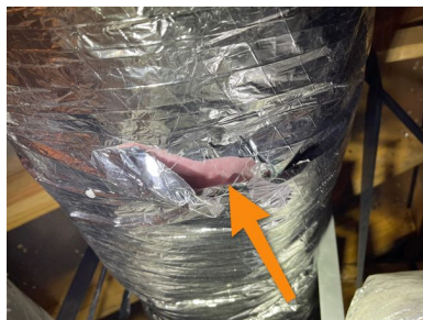
Left of furnace
