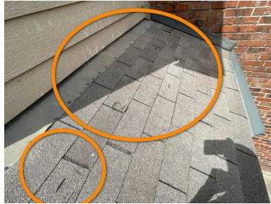
Ladder damage front porch
