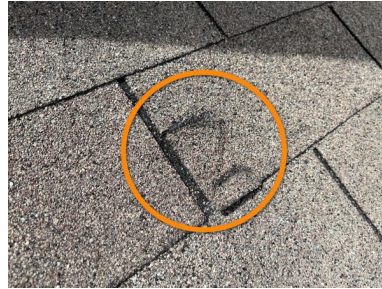
Close up ladder damage front porch
