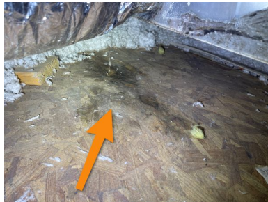
Left of furnace
