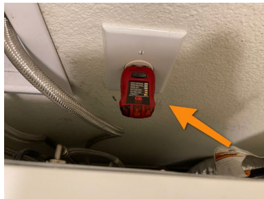
Washing machine outlet
