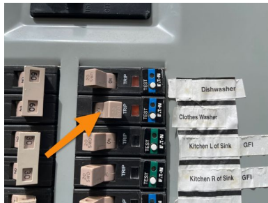
Washing machine breaker
