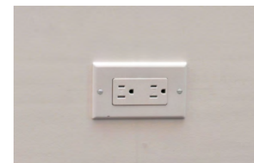
Outlets in baseboards
