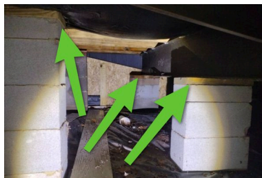
Termite blocks not present
