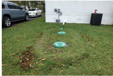
Photo(s) of trash tank(s):
