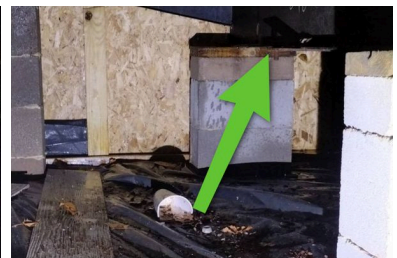
Termite blocks not present
