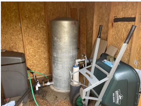
Well equipment general view
