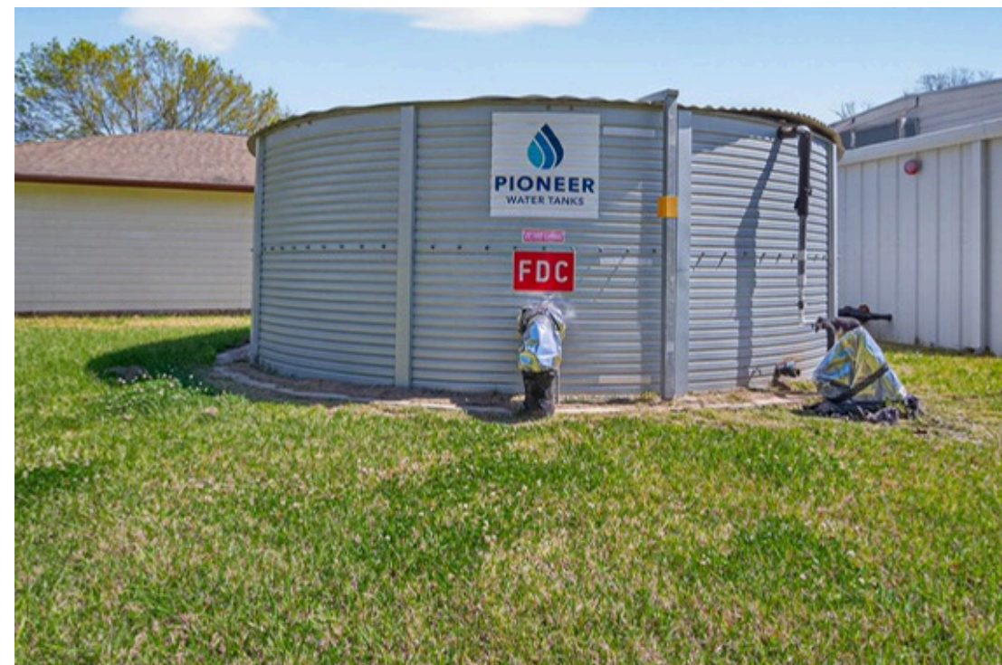
Full infrastructure in place: well water, septic, electricity, internet & irrigation
