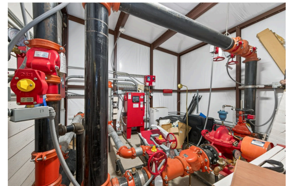
Commercial fire sprinkler & alarm System
