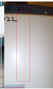
C. Item 2 (Picture) Sign of previous moisture
