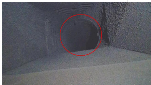
J. Item 4 (Picture) Missing fireplace damper
