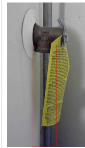
C. Item 3 (Picture) Missing drain line for TP&R valve
