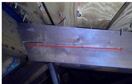
D. Item 7 (Picture) Cracked rafter
