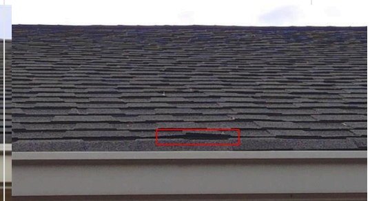
C. Item 9 (Picture) Raised shingle
