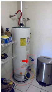
C. Item 4 (Picture) Cold water line installed at the bottom of the water heater, water heater sitting on floor
