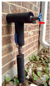
F. Item 4 (Picture) Missing anti-siphon device
