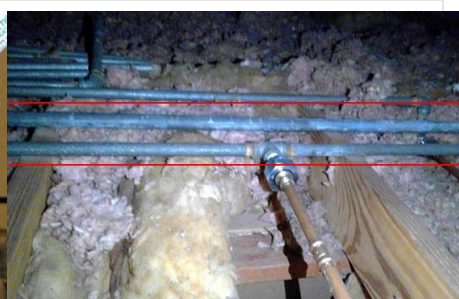
A. Item 2 (Picture) Galvanized plumbing
