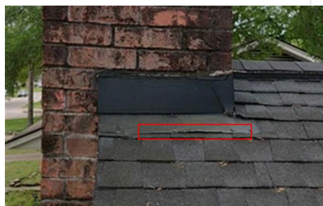
J. Item 1 (Picture) Raised chimney flashing
