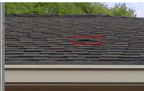
C. Item 8 (Picture) Raised shingle
