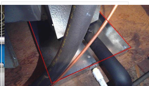
B. Item 3 (Picture) Missing float switch in drain pan
