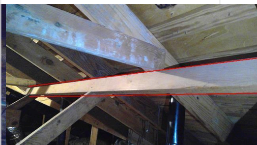
D. Item 3 (Picture) Undersized purlin bracing members
