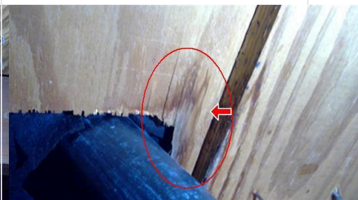
D. Item 8 (Picture) Moisture damaged roof decking
