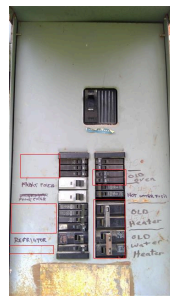
A. Item 2 (Picture) Missing/insufficient labels for breakers
