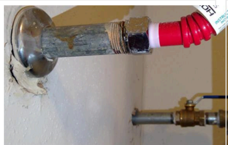
A. Item 1 (Picture) Galvanized plumbing
