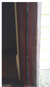
G. Item 4 (Picture) Front entry door weather stripping
