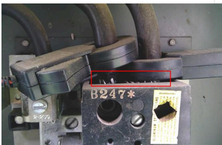
A. Item 4 (Picture) Aluminum main service entrance conductors
