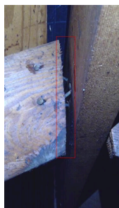
D. Item 4 (Picture) Rafter not attached to ridge beam
