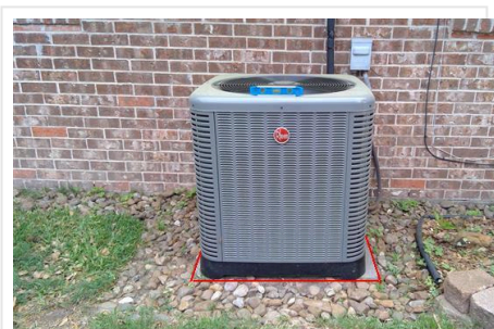
B. Item 1 (Picture) Tilted exterior air handler unit
