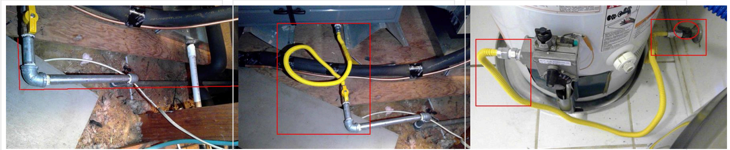
E. Item 1 (Picture) Improperly supported/secured gas line
