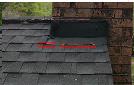
J. Item 2 (Picture) Raised chimney flashing
