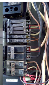
A. Item 5 (Picture) White neutral conductors being used as hot conductors
