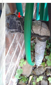
F. Item 3 (Picture) Main water line on left (front facing) side of home
