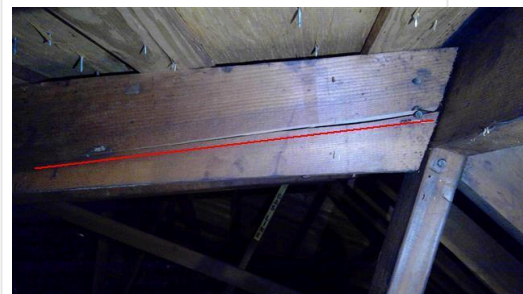
D. Item 6 (Picture) Cracked rafter
