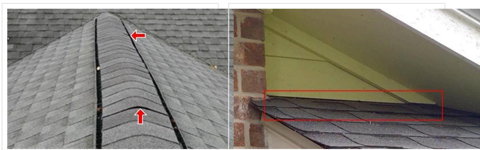
C. Item 10 (Picture) Raised shingles
