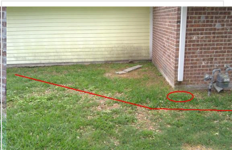
B. Item 2 (Picture) Back of home/missing splash block
