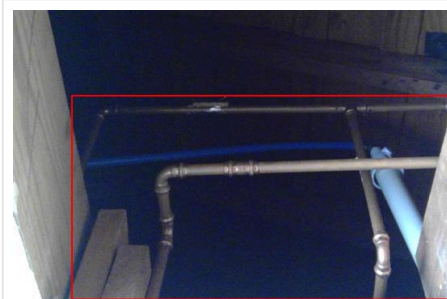
F. Item 2 (Picture) Exposed plumbing lines in attic space above garage
