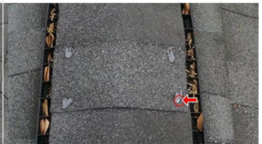
C. Item 3 (Picture) Exposed fastener (nail) head
