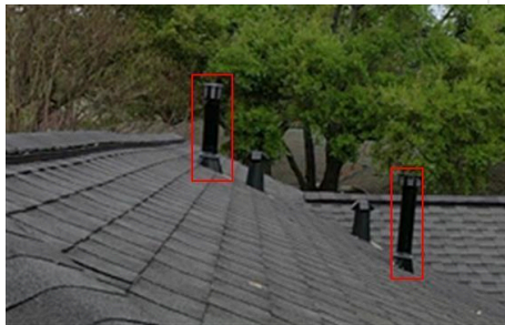
C. Item 4 (Picture) Combustion air vents for water heater and furnace
