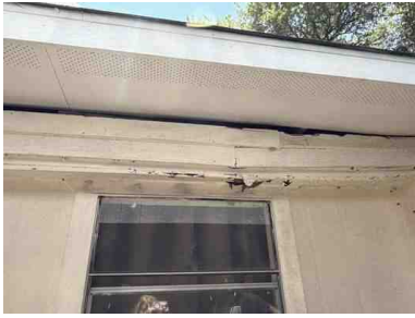
Wood Rot-Front Right
