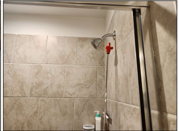
LOW PRESSURE / POOR WATER FLOW
