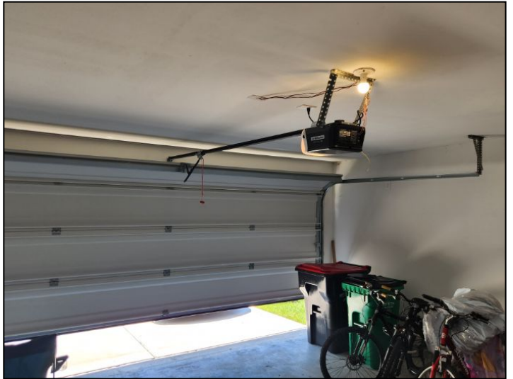
GARAGE DOOR OPENER OPERATIONAL
