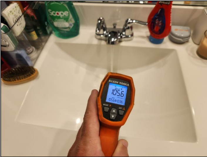
HOT WATER OK
