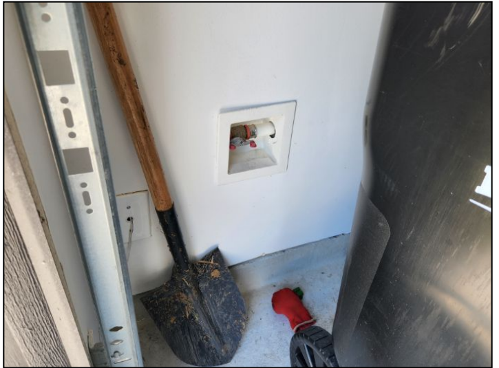
MAIN WATER VALVE OK
