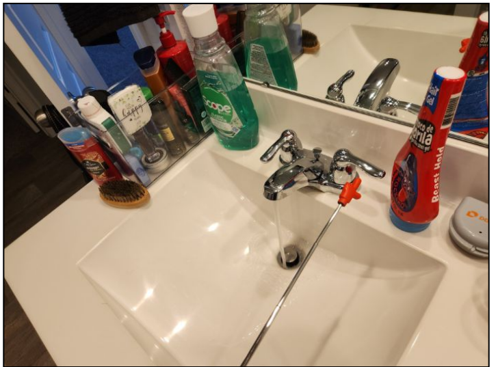
LOW PRESSURE / POOR WATER FLOW
