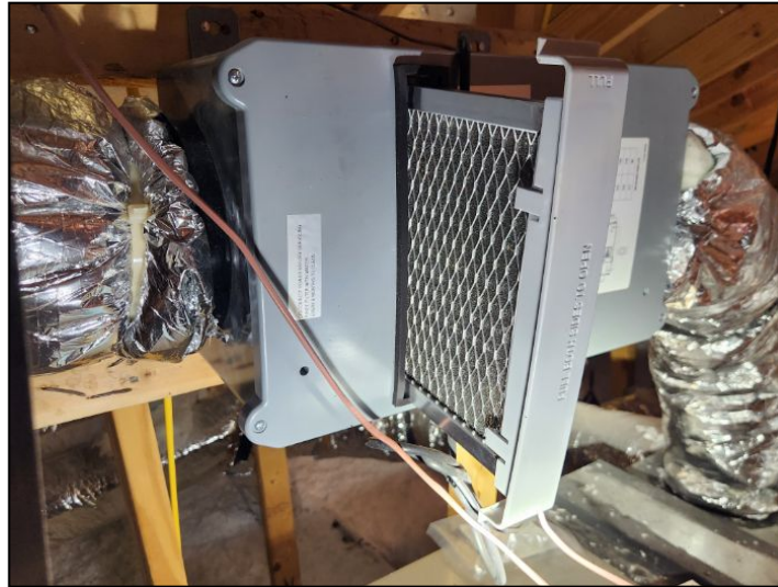
FRESH AIR FILTER OK
