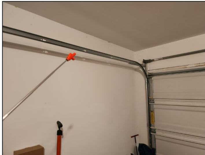
LUBRICATION NEEDED AT RAILING
