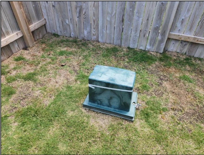
ELECTRICAL TRANSFORMER PRESENT
