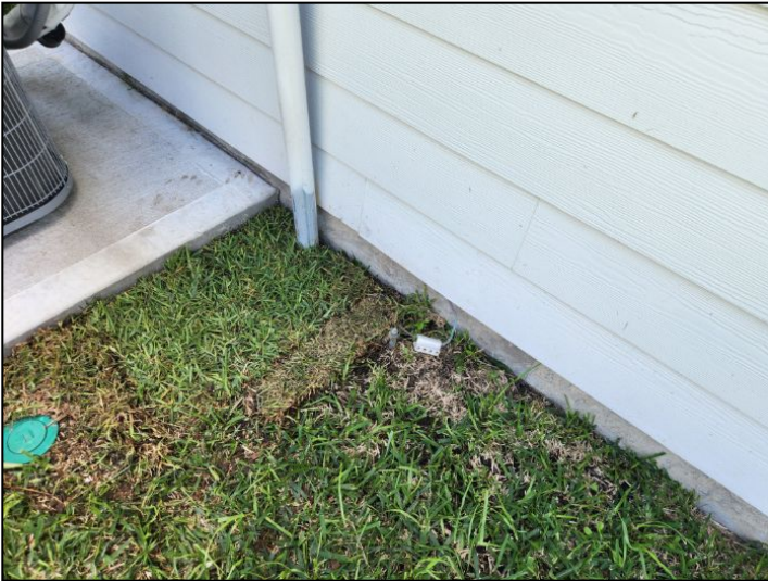
MAIN GROUNDING OK
