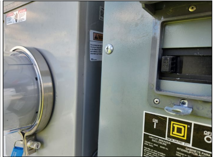
MAIN BREAKER OK
