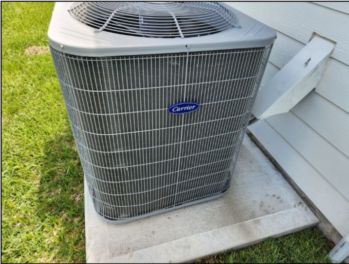
CONDENSING UNIT OK
