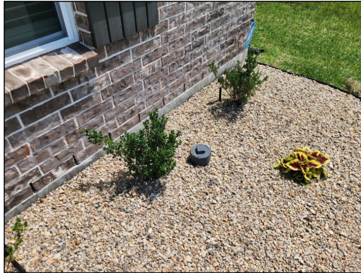
MAIN CLEANOUT OK
