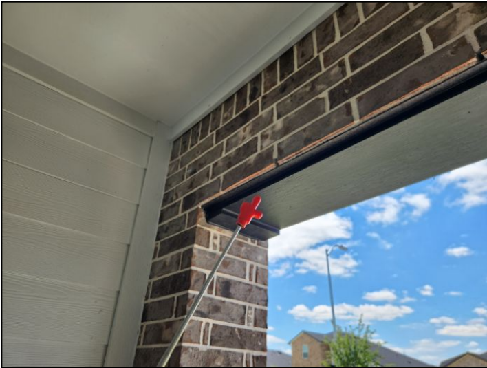
RUST / DETERIORATION AT METAL LINTEL
