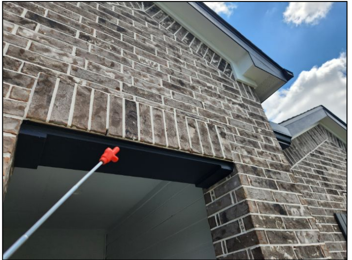
RUST / DETERIORATION AT METAL LINTEL
