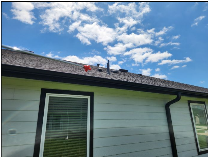
LINT BUILDUP AT DRYER VENT
