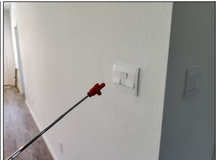
DAMAGED / INOPERABLE 3 WAY SWITCH
