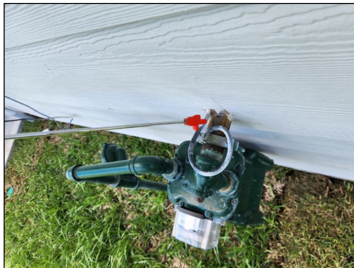
RUST / DETERIORATION AT GAS MAIN
