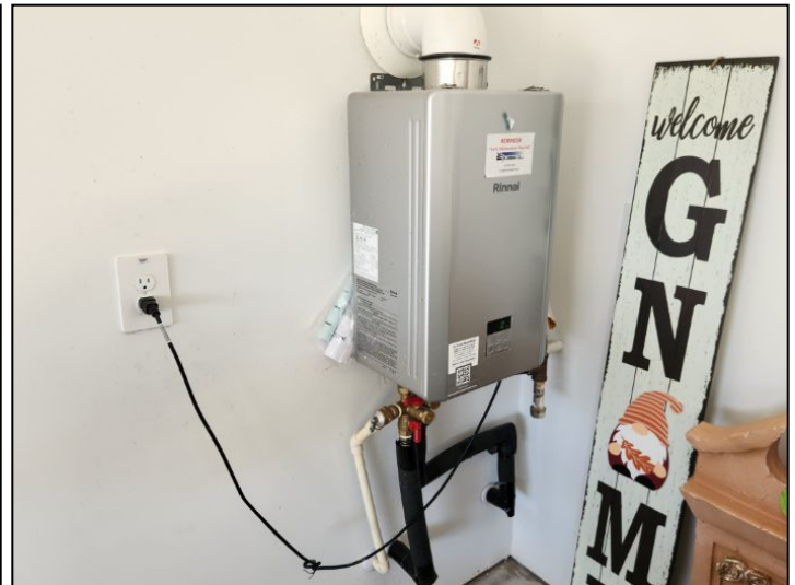
WATER HEATER OK
