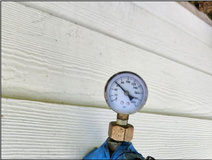
WATER PRESSURE OK; 60 PSI
