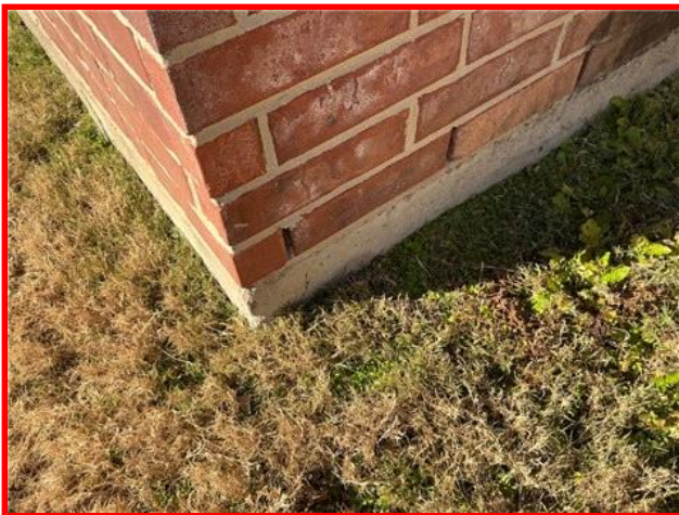
Cracked Corner at Rear Right {atop
