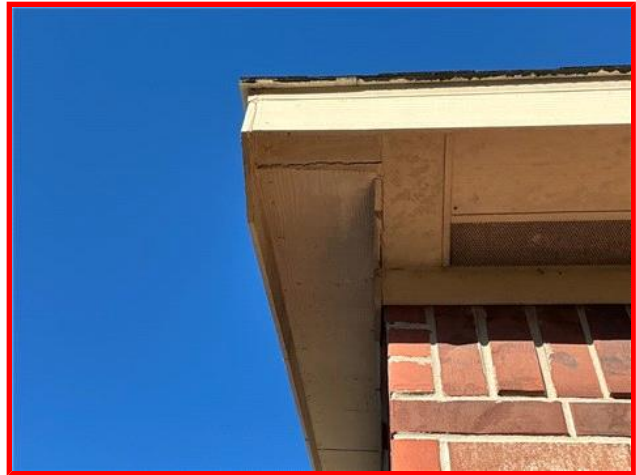
Soffit Separation at Left
