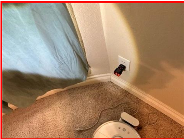
Loose Outlet in Primary Bedroom
