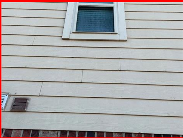
Siding Separation at Left
