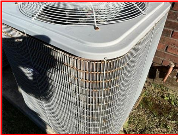
Rust at A/C Housing
