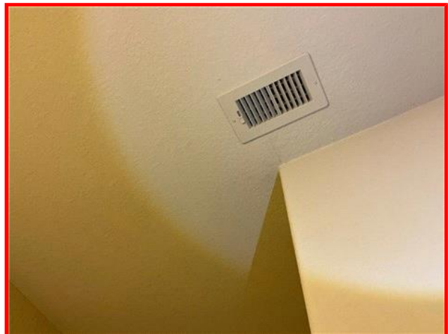
Crack in Ceiling in Upstairs Bathroom
