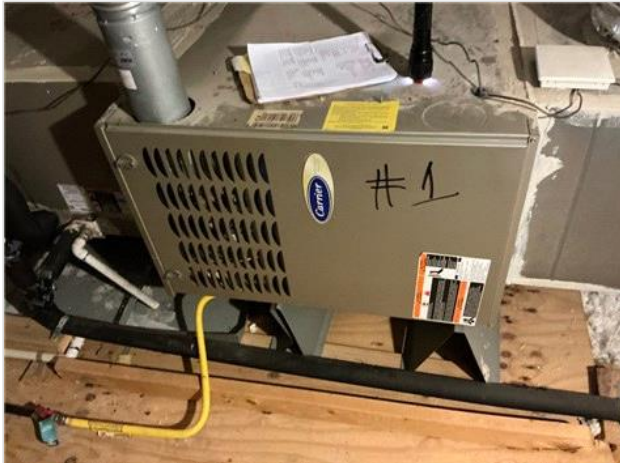
Heating Equipment Cover Not Removed
