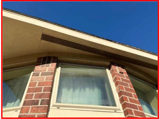
Failed Thermal Seal at Primary Bedroom
