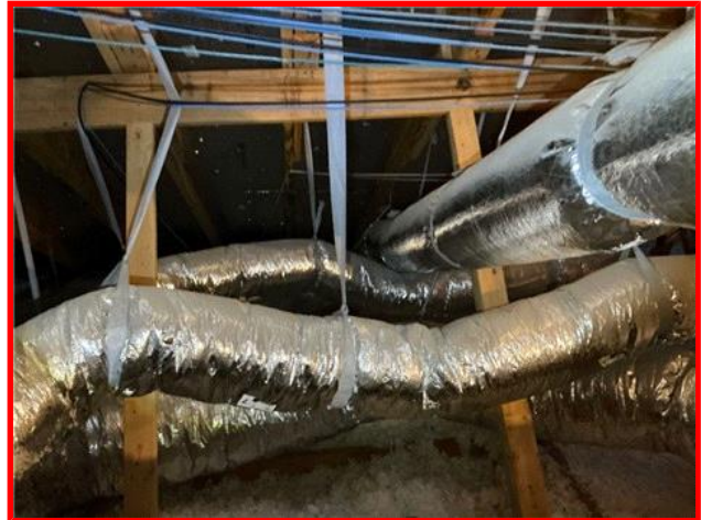
Ducts in Contact
