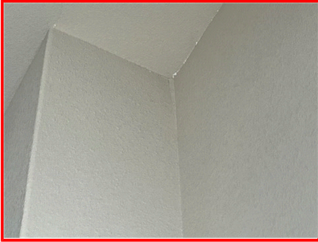
Seam Tape Failure in Downstairs Bedroom
