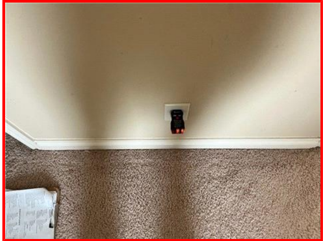
Loose Outlet in Downstairs Bedroom
