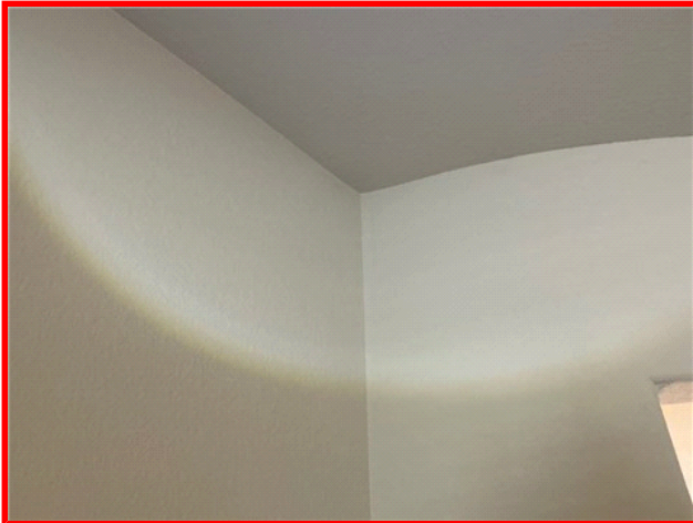
Seam Tape Failure in Game Room
