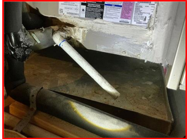
Drip Pan Not Properly Sloped
