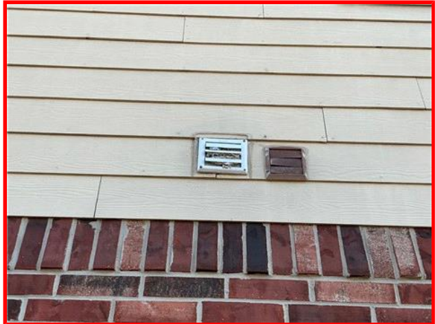
Damage & Debris at Wall Vent
