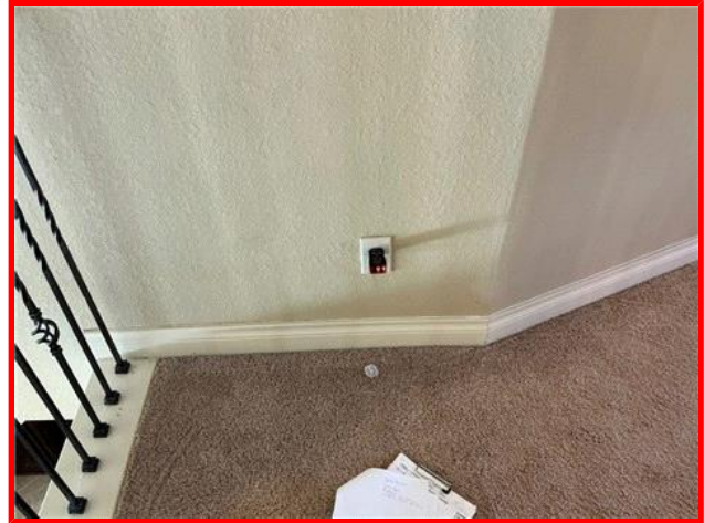
Loose Outlet in Upstairs Hall
