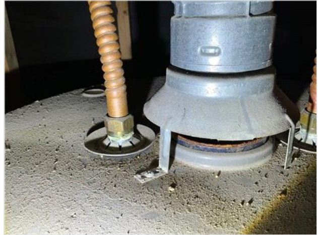
Rust beginning at Water Heater
