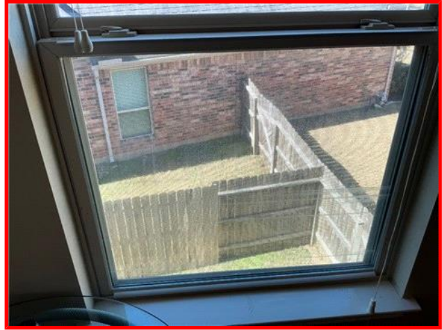
Failed Thermal Seal at Upstairs Rear Bedroom
