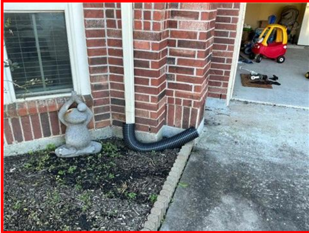
Improper Downspout Discharge
