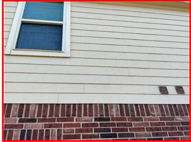
Siding Separation at Left
