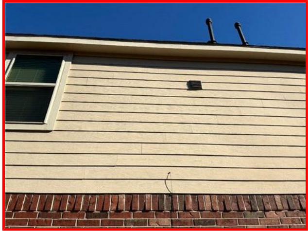
Siding Separation at Right
