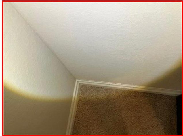
Baseboard Separation in Upstairs Game Room
