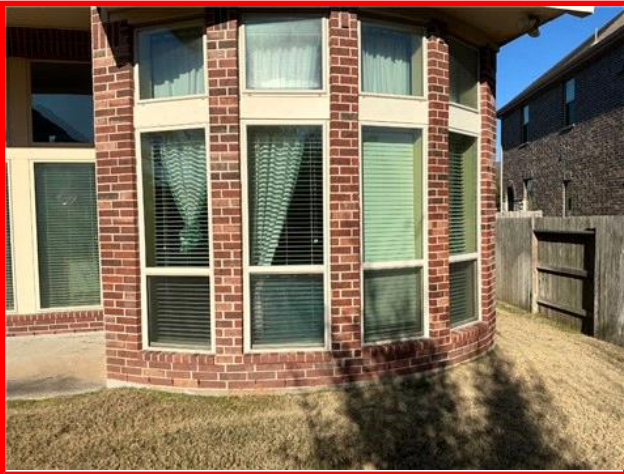
Failed Thermal Seal at Primary Bedroom
