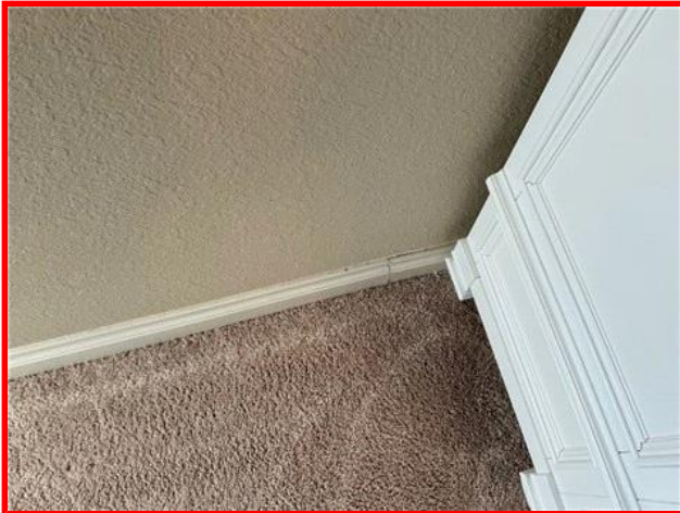
Baseboard Separation in Primary Bedroom
