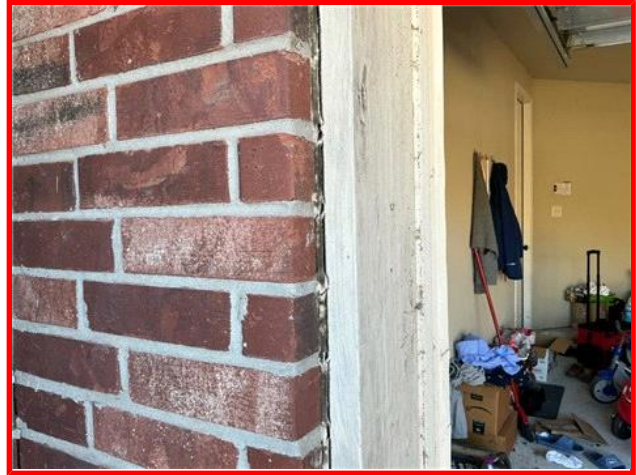
Deteriorated Caulk at Garage
