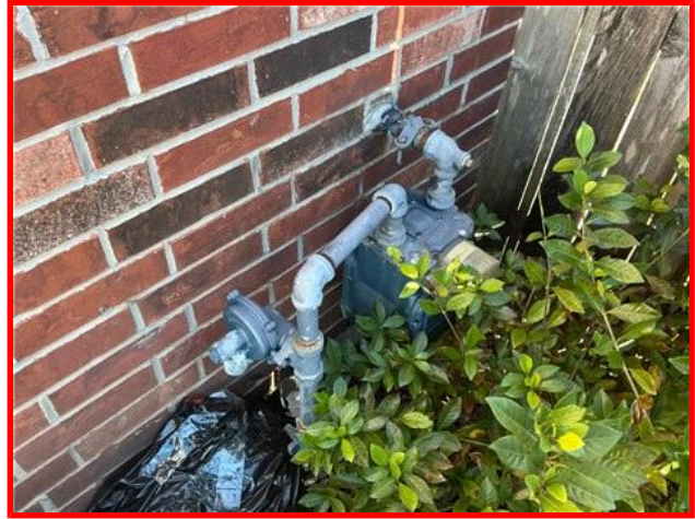
Missing Sleeve and Vegetation in Contact with Gas Meter
