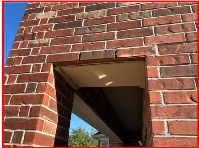
Separation at Garage Trim
