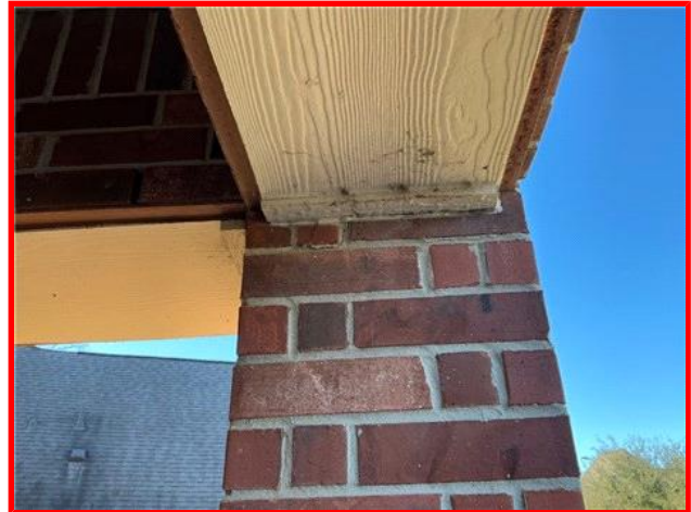
Damaged Brick at Garage
