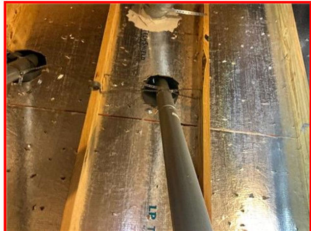
Light Coming Through at Water Heater Vent
