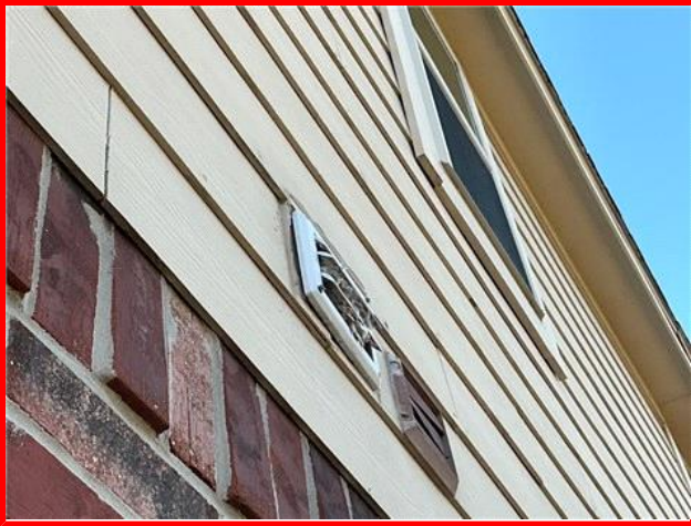
Vent Not Sealed
