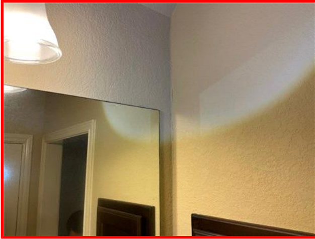
Corner Crack at Jack and Jill Bathroom
