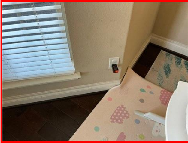
Loose Outlet in Dining Room
