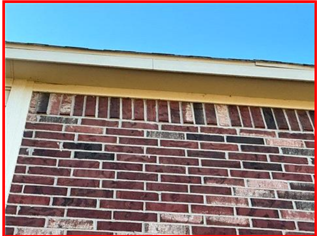
Damaged Drip Edge Flashing at Left
