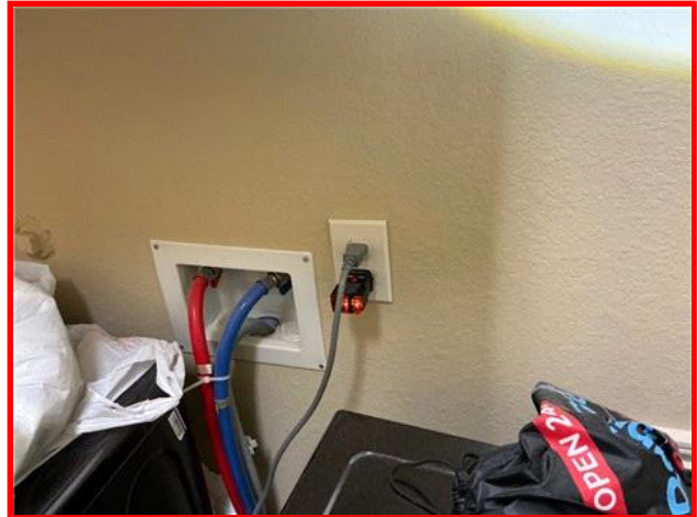
Missing GFCI Protection in Laundry Room
