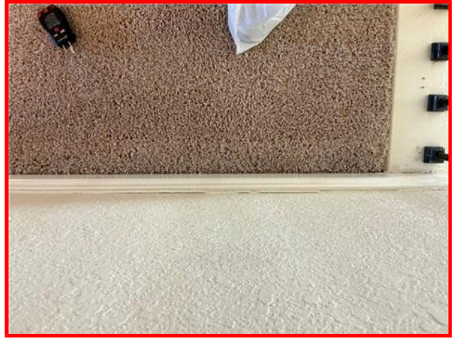
Separation in Baseboard Upstairs Hall
