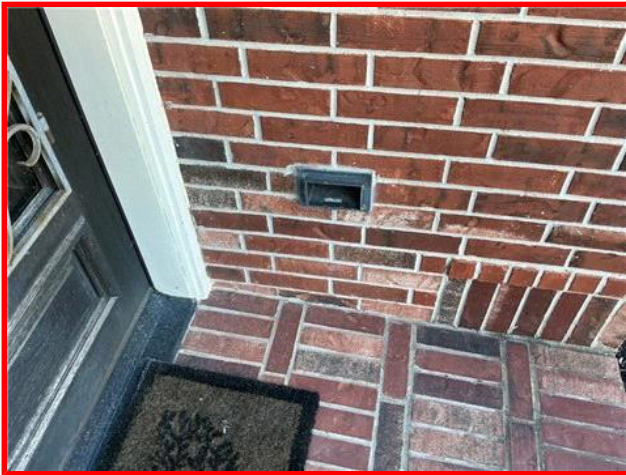
Missing Exterior Outlet Cover
