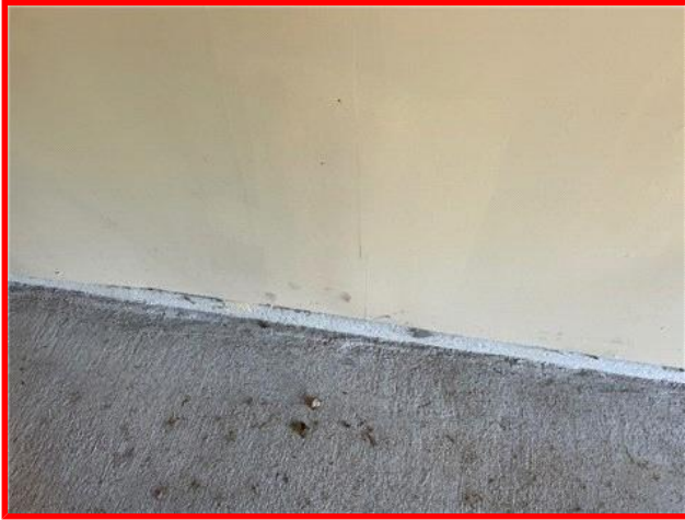
Crack in Garage Wall
