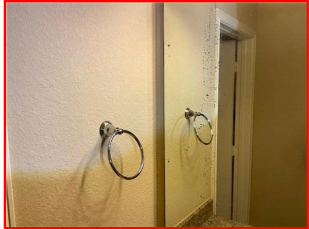
Mirror Damaged in Jack and Jill Bathroom
