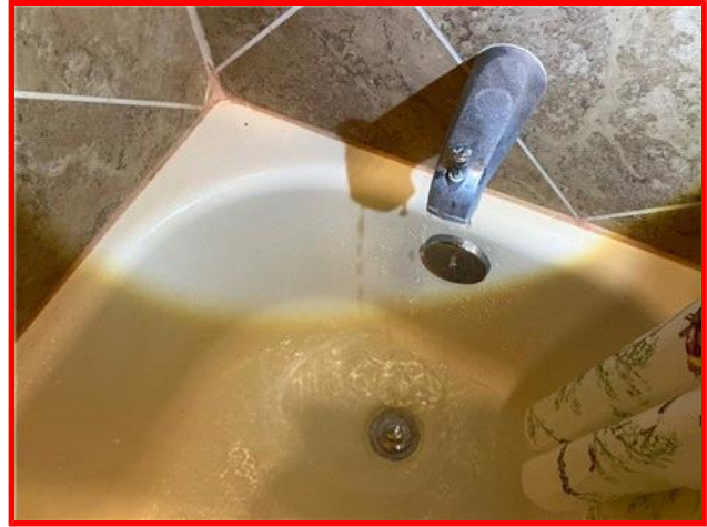
Upstairs Bathroom Diverter Does Not Function Properly
