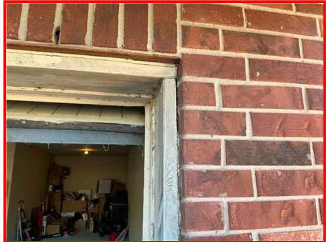
Garage Trim Separation
