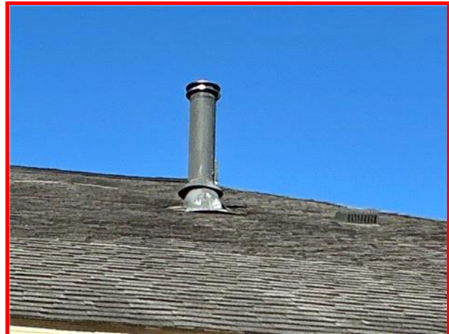
Lifted Chimney Boot
