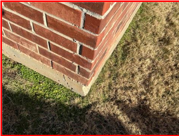
Crack at Right Rear Corner
