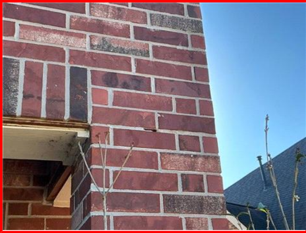
Lintel Exposed Through Wall at Garage
