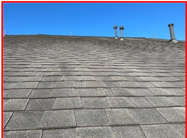
Roof - Granular Loss
