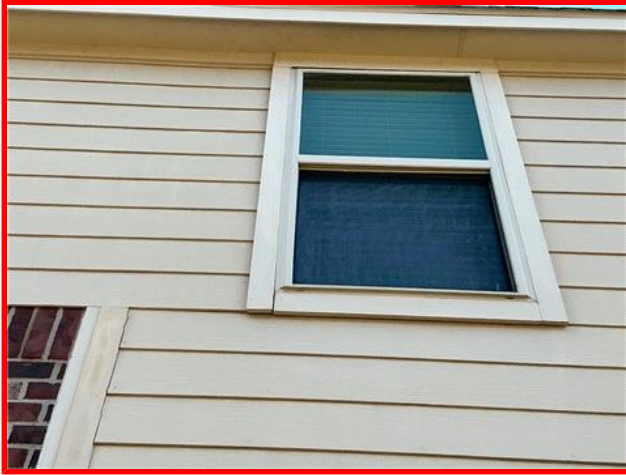
Trim Separation at Left
