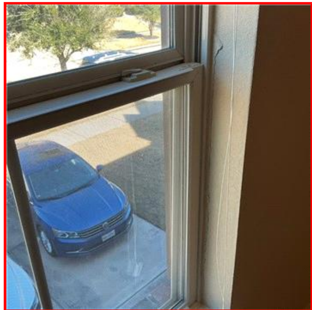
Window Framing Separation / Crack at Upstairs Front Bedroom
