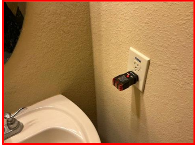
Loose Outlet in Half Bathroom
