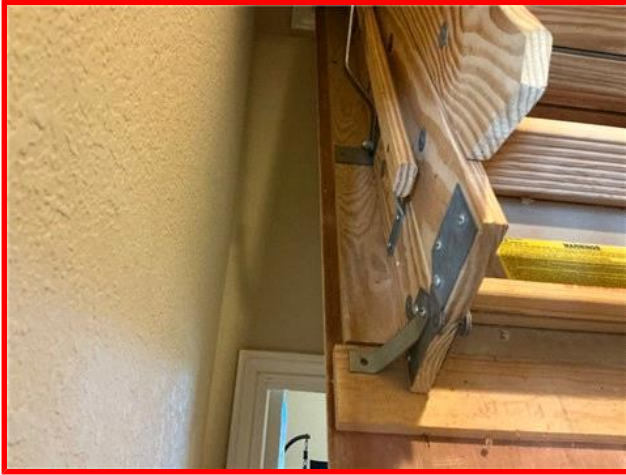
Loose Hardware at Attic Ladder
