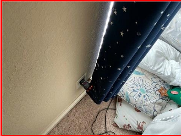
Loose Outlet in Downstairs Bedroom
