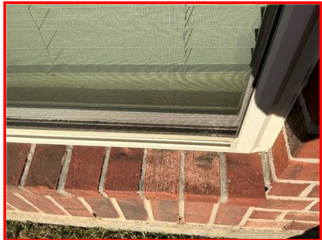
Voids in Mortar at Rear
