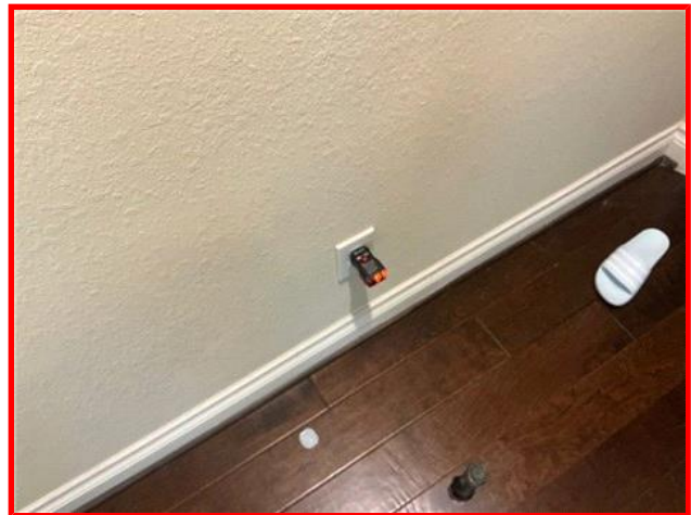
Loose Outlet in Primary Bedroom
