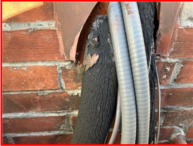
Deteriorated Refrigerant Line Insulation
