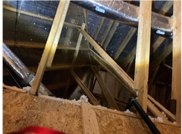
Broken Framing Member in Attic
