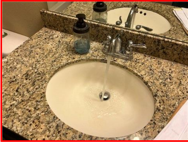
Stopper Does Not Engage in Upstairs Bathroom
