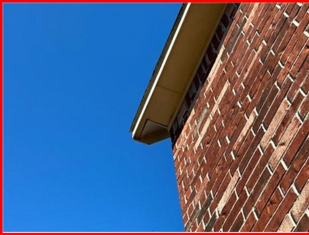
Soffit Separation at Right
