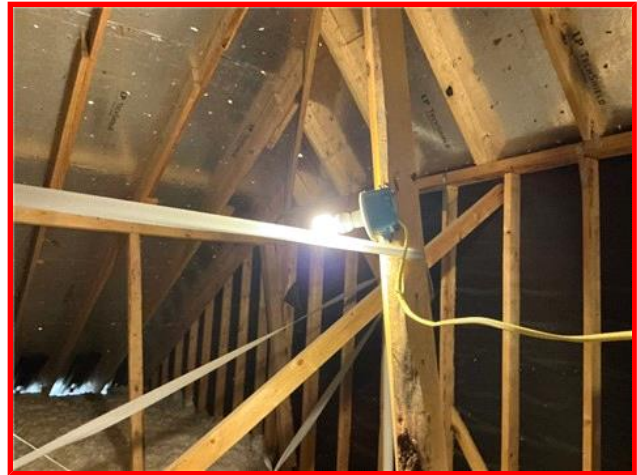
Attic Light Missing Cover
