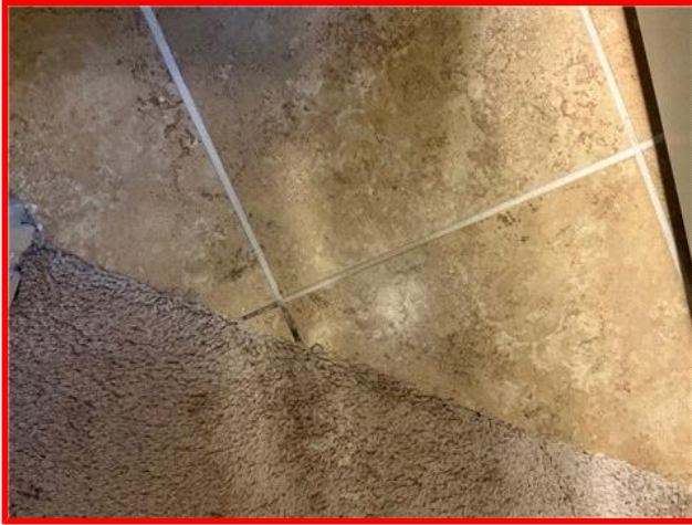
Missing Grout in Downstairs Bathroom Floor
