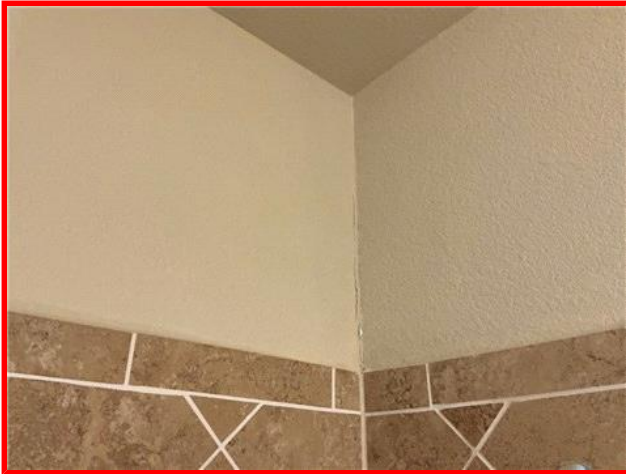
Wall Separation in Downstairs Bathroom
