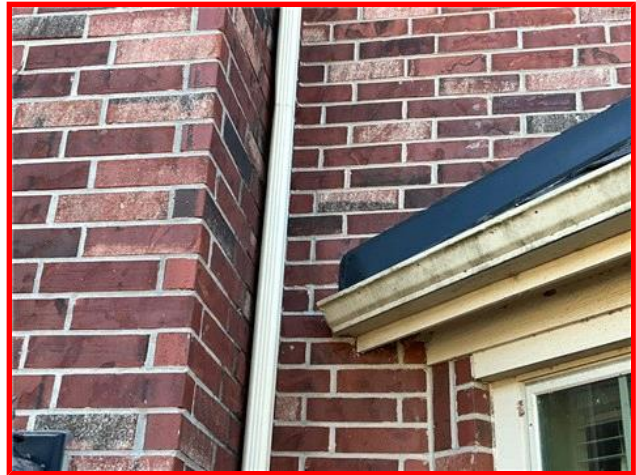
Missing Kickout Flashing at Front
