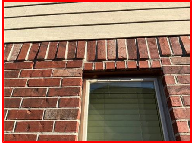
Crack in Brick at Right
