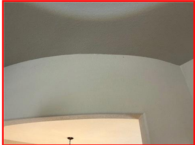
Crack in Upstairs Game Room
