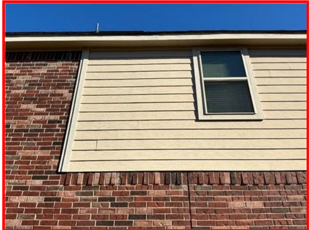
Siding Separation at Right
