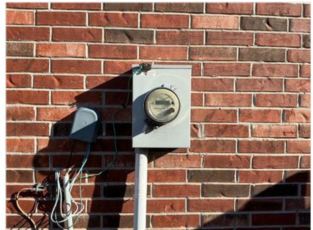
Incoming Electrical Service
