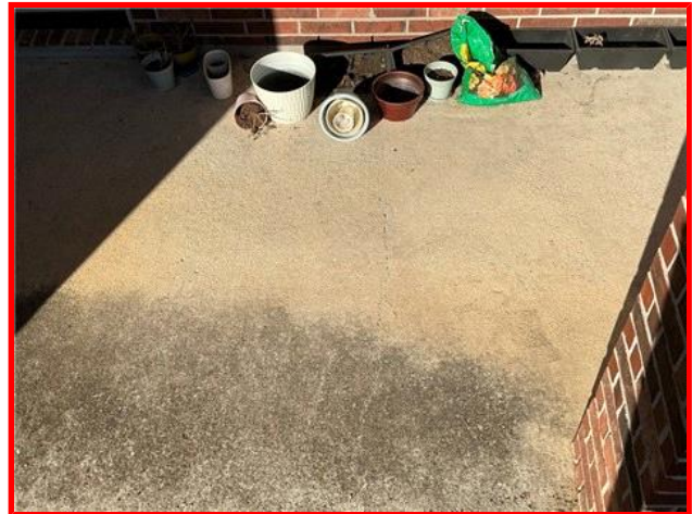
Crack in Patio
