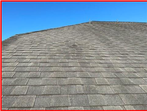
Granular Loss & Raised Vent Boot
