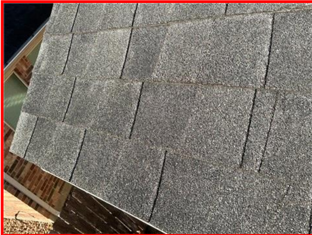
Roof - Granular Loss
