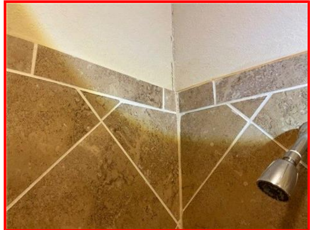
Separation / Corner Crack in Upstairs Bathroom
