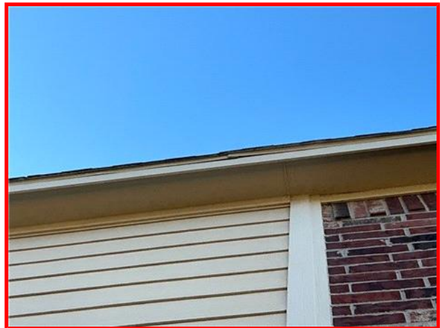
Fascia Board Separating at Left
