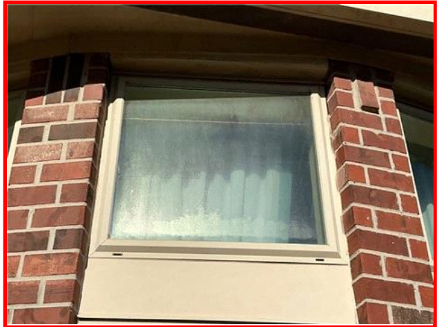
Failed Thermal Seal at Bedroom
