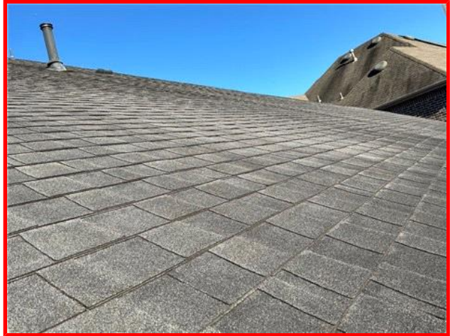
Roof - Granular Loss
