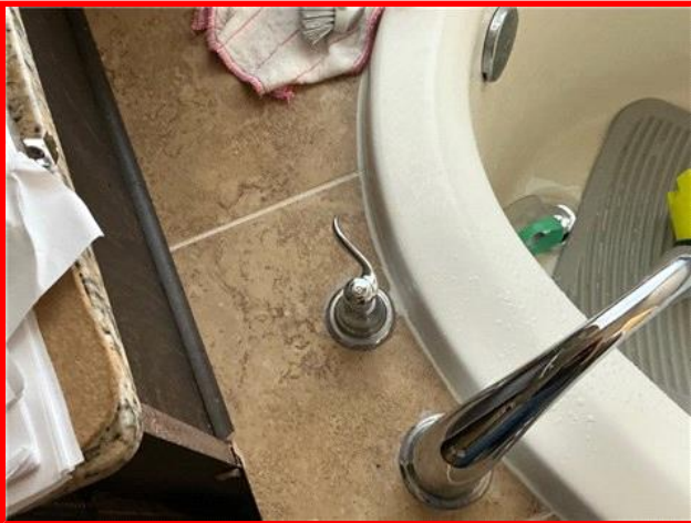
Loose Handle at Primary Bathroom Tub
