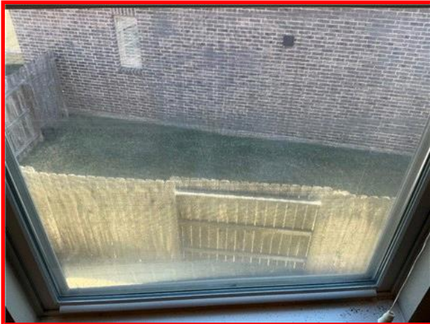
Failed Thermal Seal at Left Upstairs Bedroom
