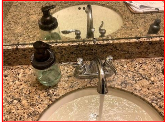
Loose Handle at Jack & Jill Bathroom Sink
