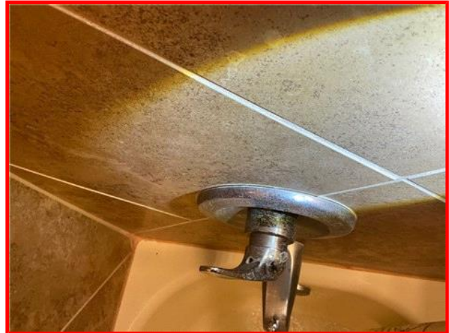
Missing Caulk at Tub Faucet
