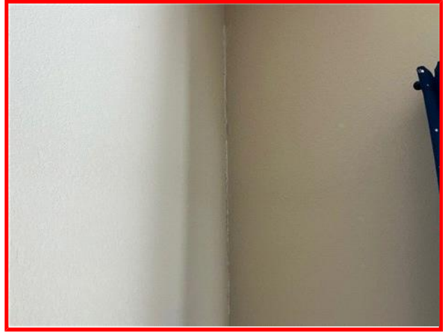
Separation in Downstairs Bedroom
