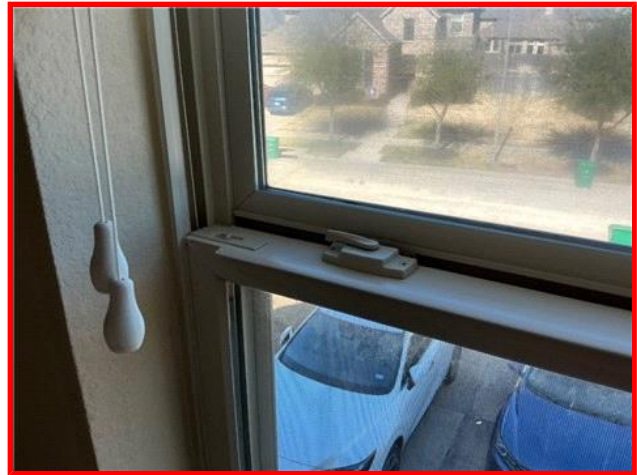
Failed Thermal Seal at Game Room - Window Difficult to Close
