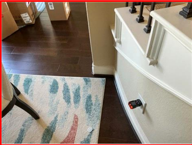
Loose Outlet in Dining Room
