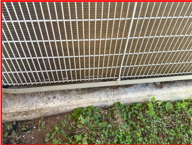
Damaged Coils at A/C Unit
