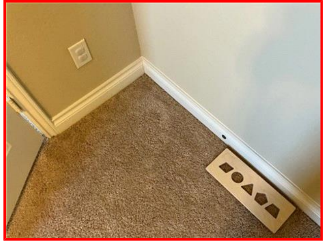
Missing Doorstop in Upstairs Front Room
