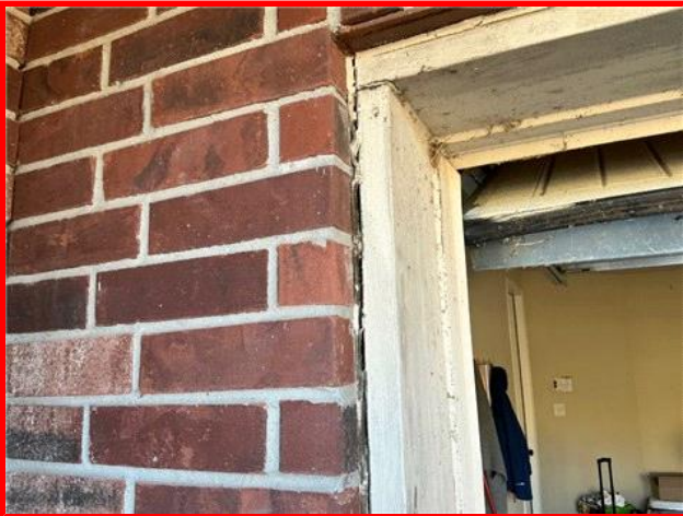
Garage Trim Separation
