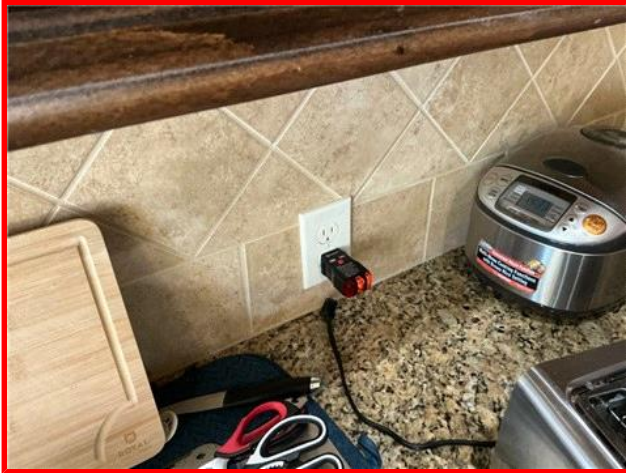
Loose Outlet in Kitchen
