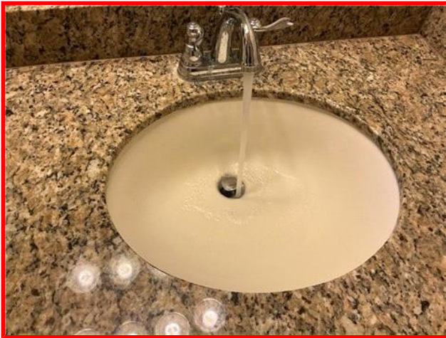
Stopper Does Not Engage in Jack and Jill Bathroom
