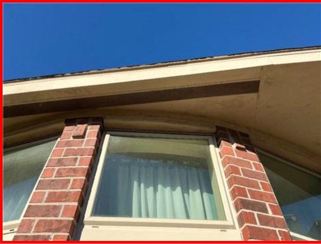
Failed Thermal Seal at Primary Bedroom
