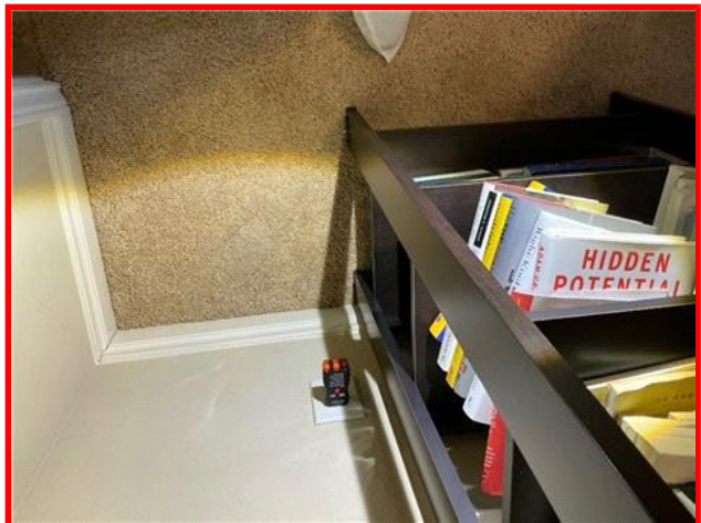
Loose Outlet at Upstairs Front Left
