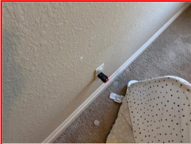
Loose Outlet in Upstairs Front Bedroom
