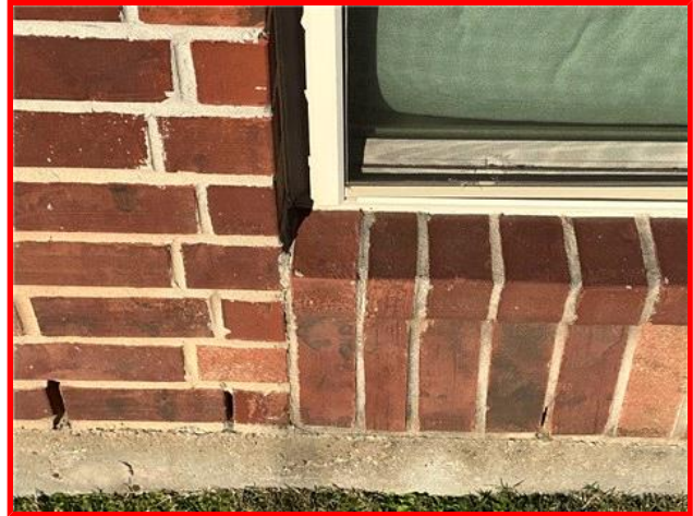
Crack in Mortar at Left
