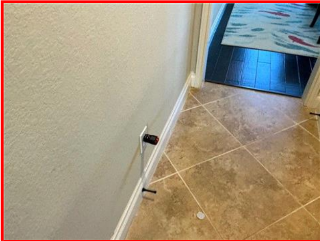
Loose Outlet in between Kitchen & Dining Room
