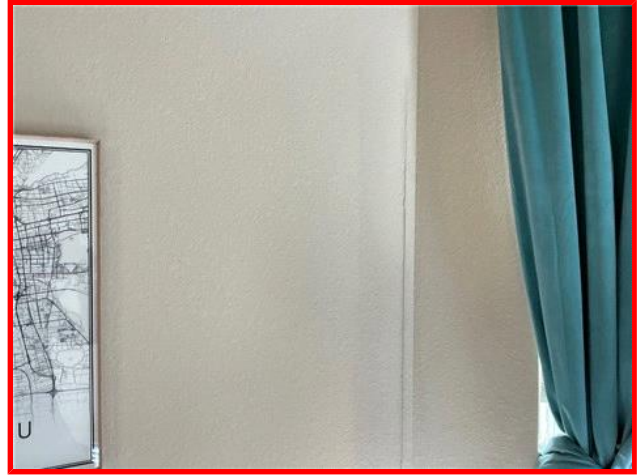
Seam Tape Failure in Primary
