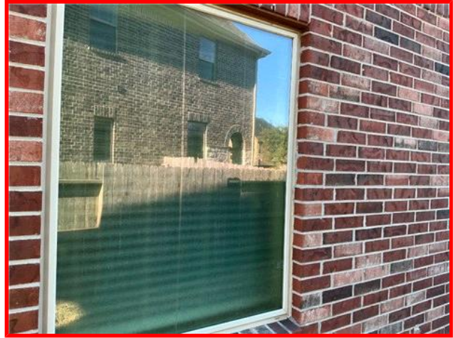
Failed Thermal Seal at Primary Bedroom
