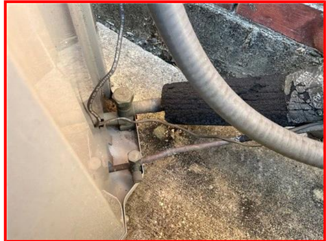
Deteriorated Refrigerant Line Insulation
