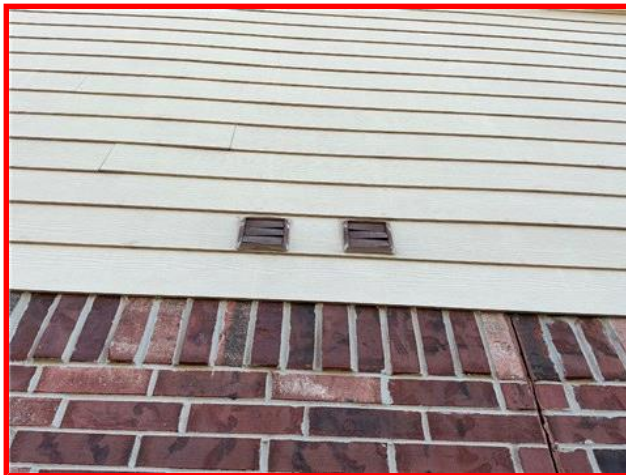
Damaged Vent Covers
