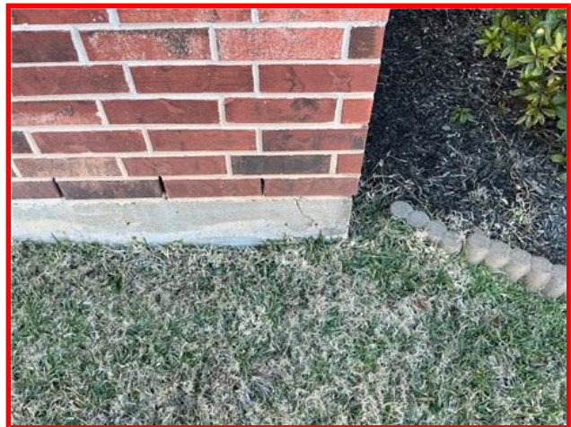
Crack at Front Left Corner
