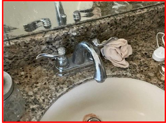
Loose Handle at Primary Bathroom Sink
