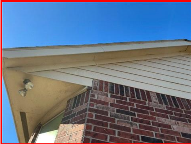
Fascia Separation at Left
