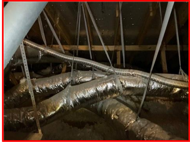
Exhaust Vent Pipes in Contact with Ducts
