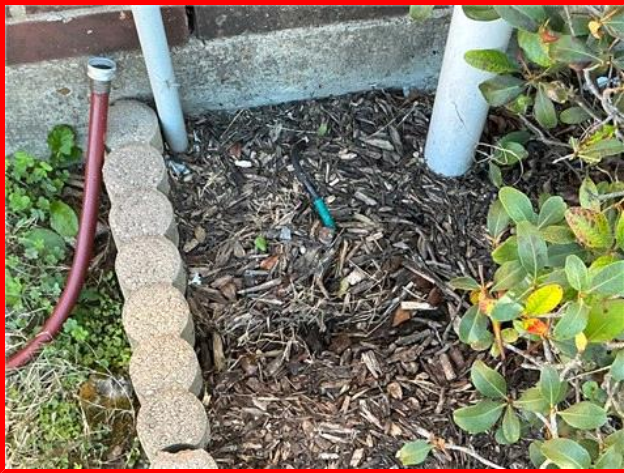
Grounding Rod Too Deep
