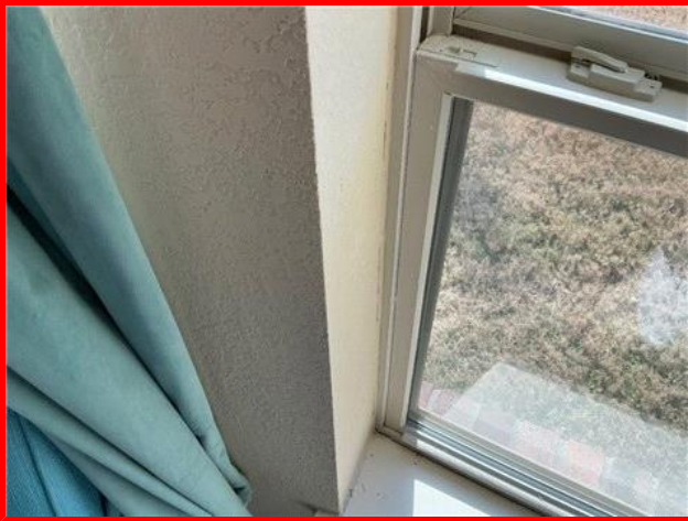
Separation / Cracks at Window Framing in Primary Bedroom
