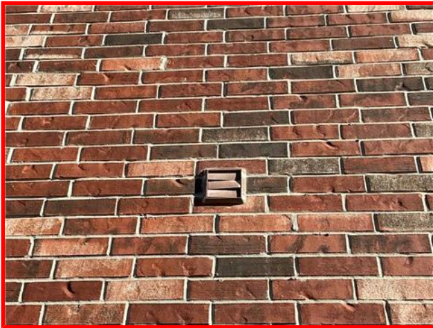
Damaged Vent Cover at Right
