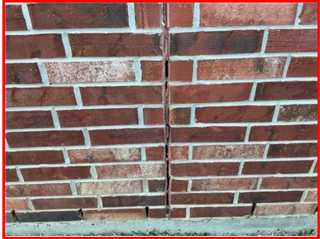
Missing Mortar at Left Expansion Joint
