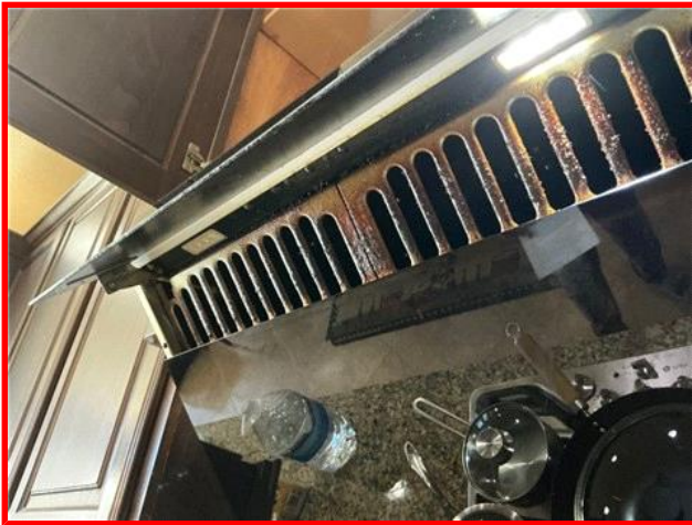
Dirty Range Vent
