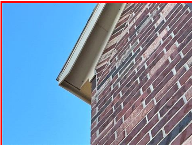
Soffit & Frieze Board Separation
