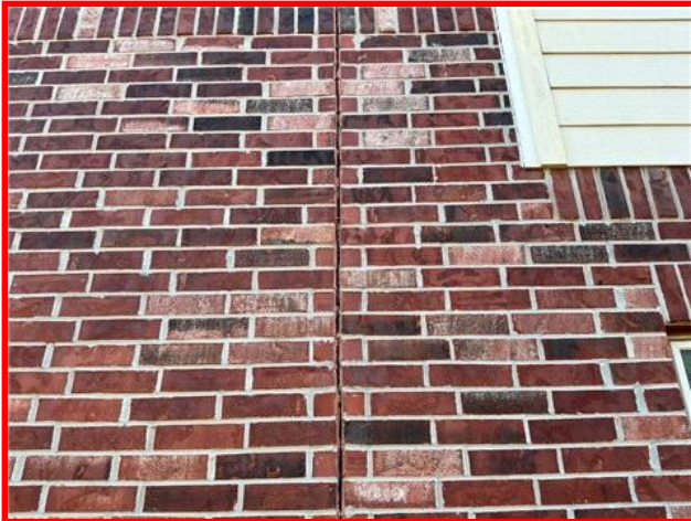
Missing Mortar at Right Expansion Joint
