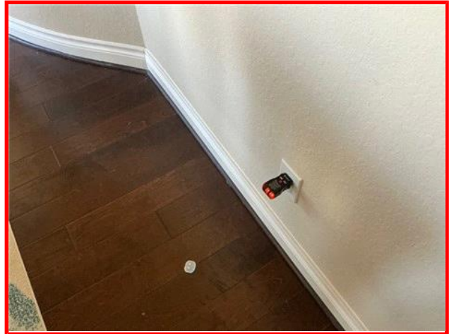
Loose Outlet in Dining Room
