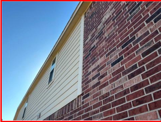
Trim Separation at Left
