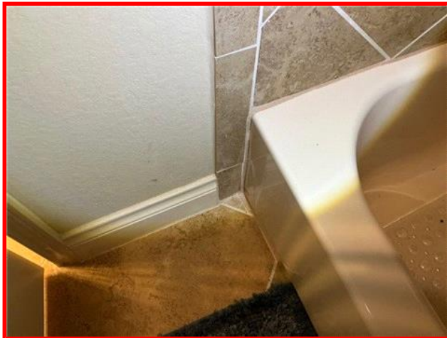
Deteriorated Caulk in Jack & Jill Bathroom
