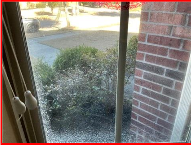
Failed Thermal Seal at Dining Room
