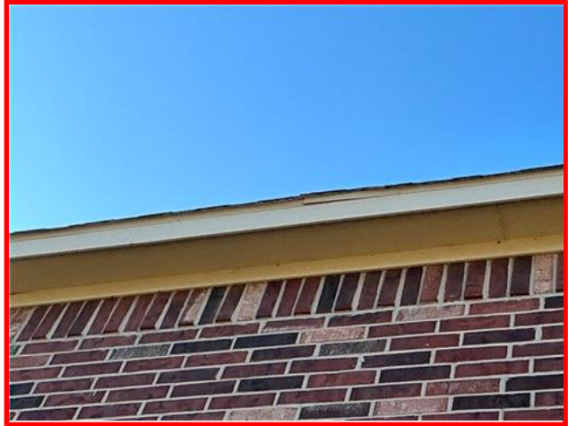
Damaged Drip Edge Flashing at Left
