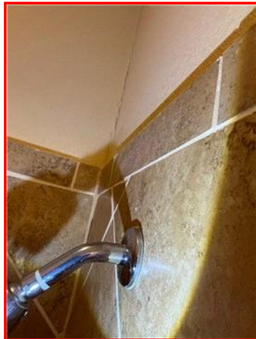
Caulk Missing around Shower Head in Upstairs Bathroom
