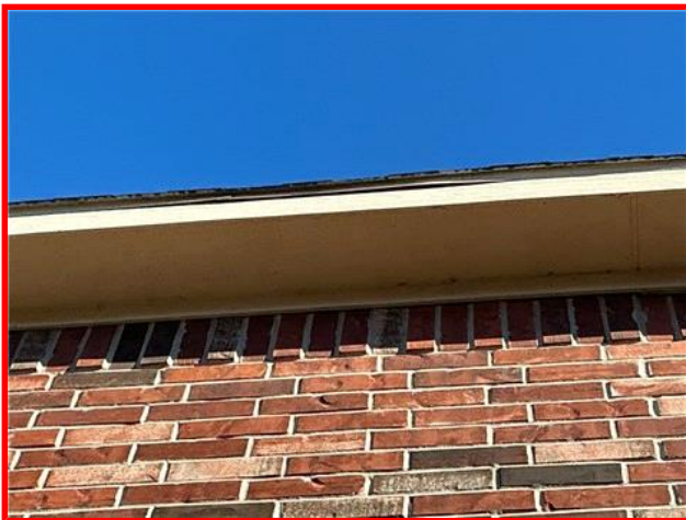
Damaged Flashing at Left
