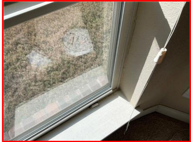
Separation around Window in Primary Bedroom
