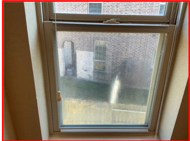
Failed Thermal Seal at Jack & Jill Bathroom
