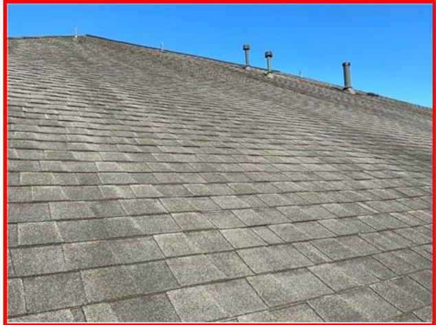
Roof - Granular Loss
