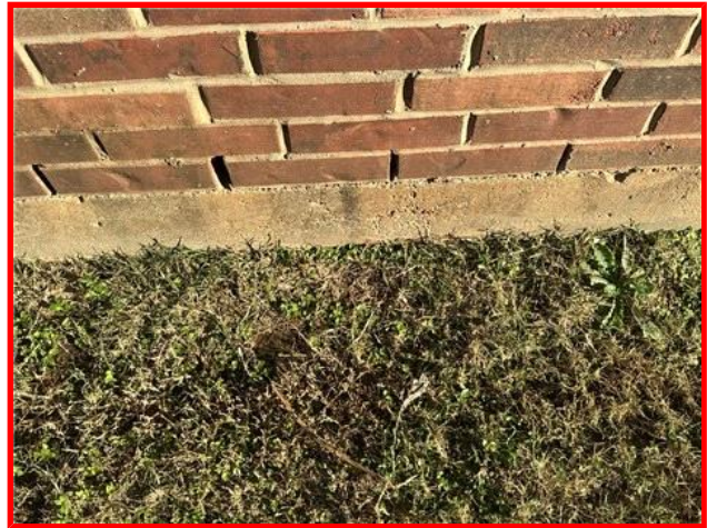
Spalling at Left
