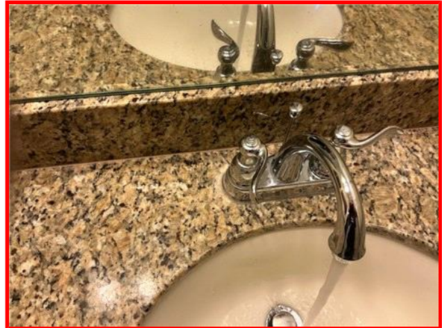
Loose Handle at Jack & Jill Bathroom Sink
