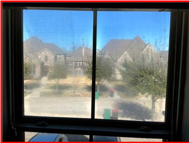
Failed Thermal Seal at Upstairs Front Bedroom
