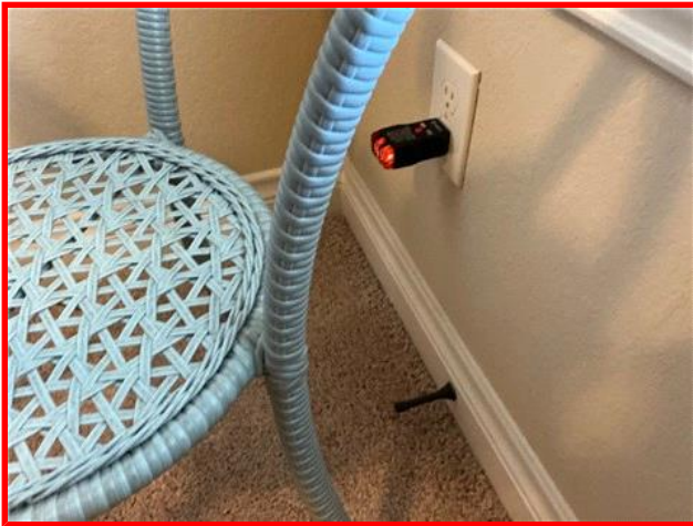
Loose Outlet in Upstairs Back Bedroom
