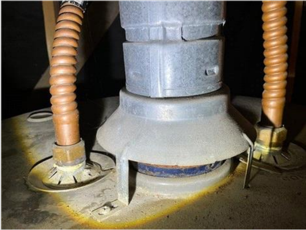
Rust beginning at Water Heater
