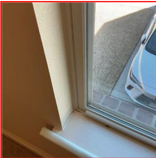
Crack in Window Framing at Upstairs Front
