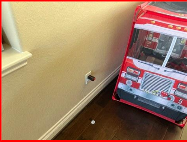
Loose Outlet in Foyer
