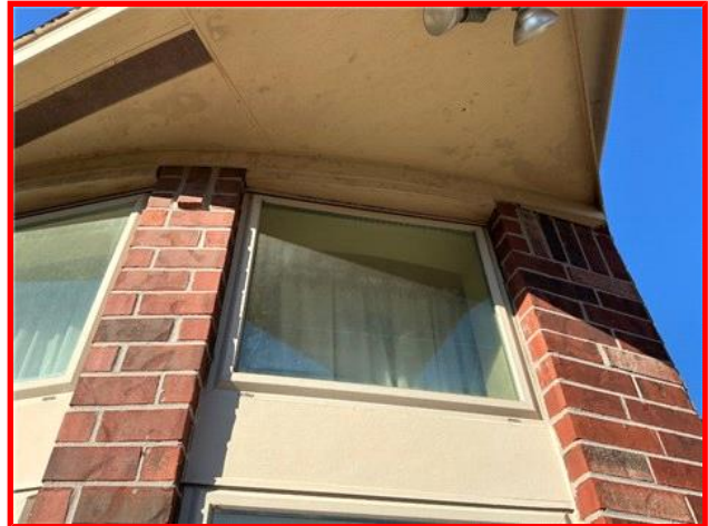
Failed Thermal Seal at Primary Bedroom
