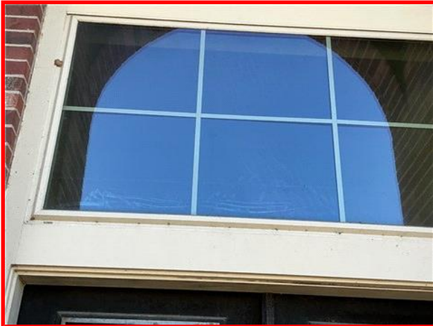
Failed Thermal Seal at Over Front Door
