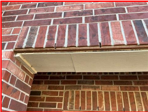
Rusted Lintel & Gap in Trim
