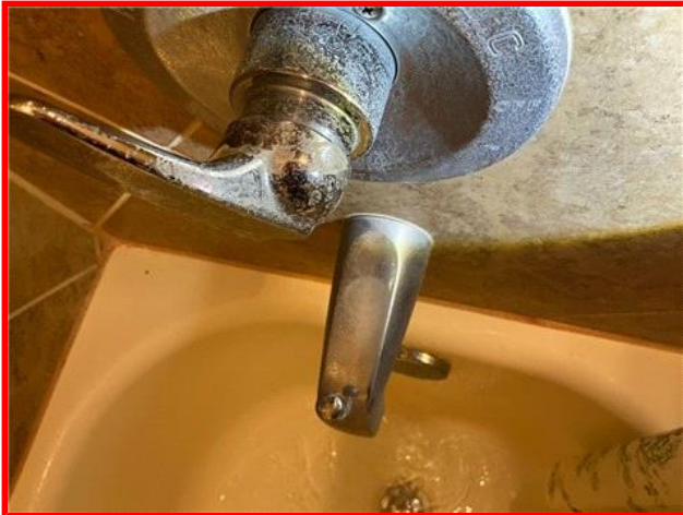
Missing Caulk at Tub Faucet
