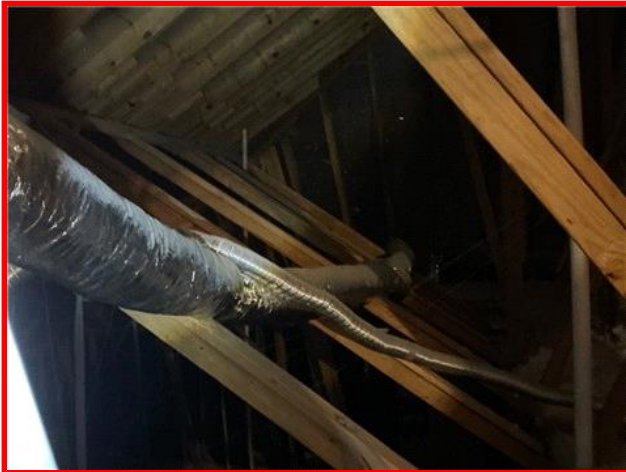
Exhaust Vent Pipes in Contact with Ducts
