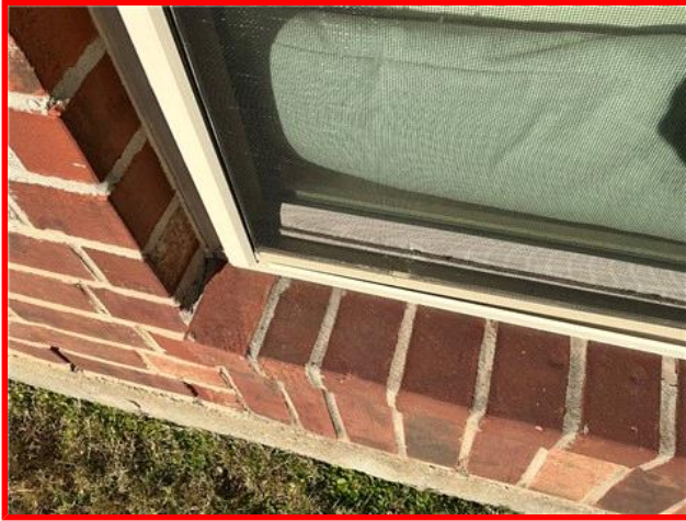
Crack in Mortar at Rear
