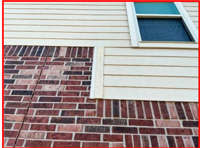
Trim Separation at Left
