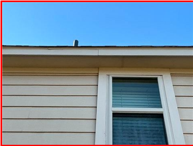
Separated Fascia at Left
