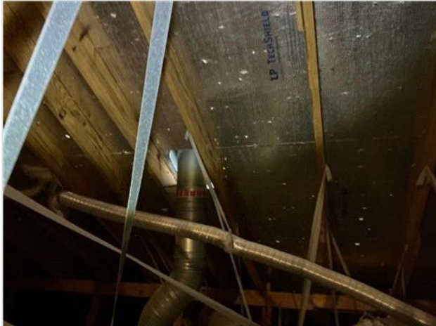
Chimney Not Sealed Properly
