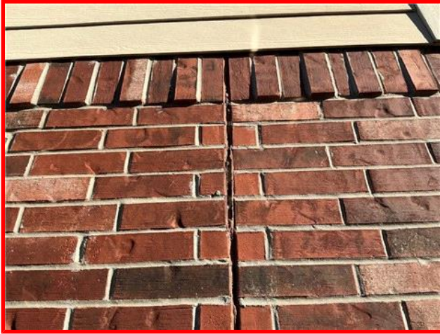
Missing Mortar at Right Expansion Joint
