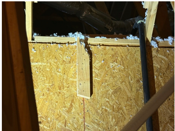
Non-structural broken piece of wood observed at walk-in attic
