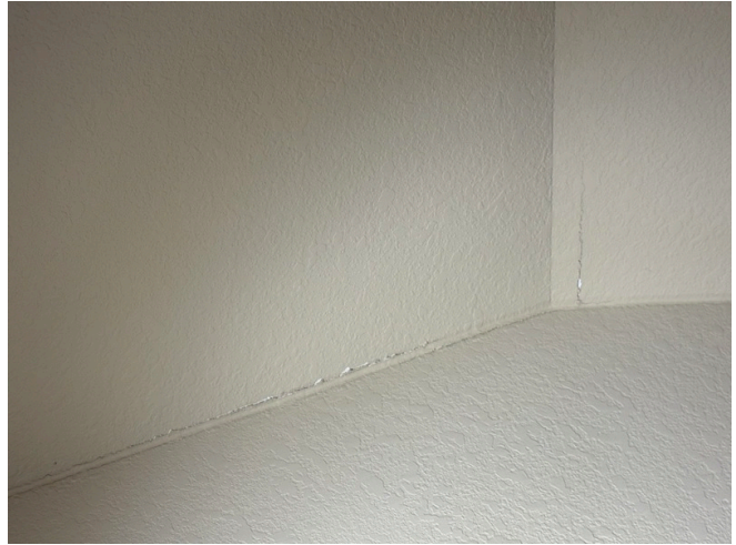
Ceiling drywall and tape seam separation in game room ceiling
