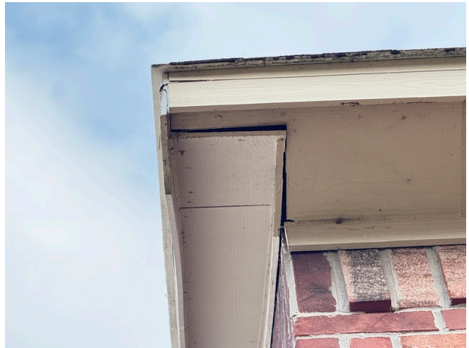
Soffit and trim separation at front right corner
