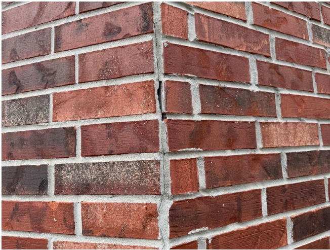
Mortar crack along corner at rear left corner
