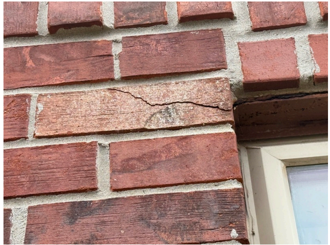
Brick crack at top left corner of bathroom window (right elevation)
