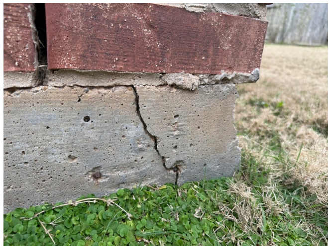
Spalled foundation grade beam resulting in wedge-crack (typical)
