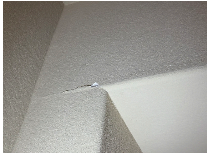
Drywall cracking visible at floor to column transition on the catwalk
