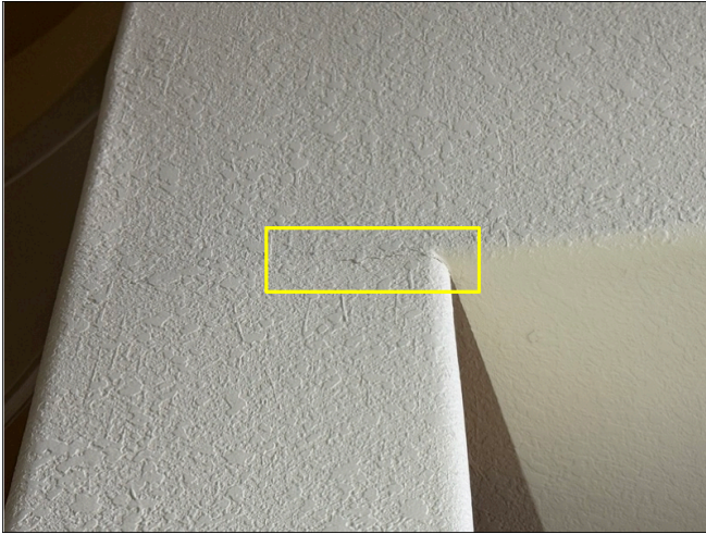
Drywall crack at the floor to column transition at the corner of the staircase in the foyer
