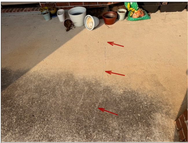
Surface crack in the patio floor (typical)
