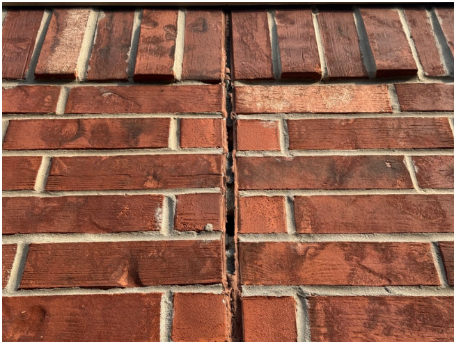
Expansion joint sealant deterioration at right elevation with openings to the wall cavity (typical)
