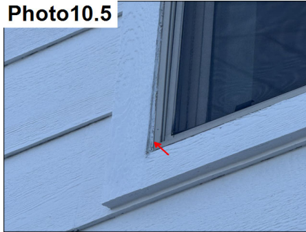
Sealant separation noted at windows in stucco and siding. Reseal all windows.
