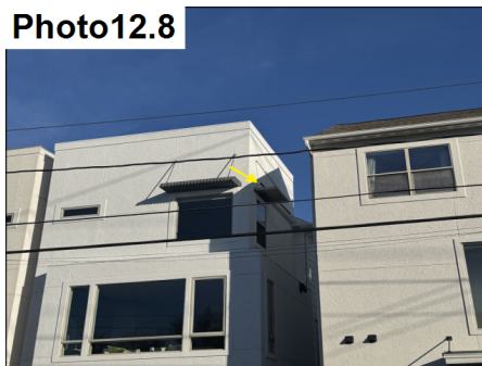
Large roof scupper flashings noted. Assess and reseat all flashing terminations.
