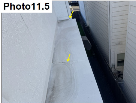
Proper metal caps are present at flat areas. Assess and reseal all metal cap terminations and transitions.
