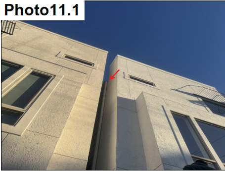
Separation noted at roof termination. Assess and thoroughly seal all roof terminations.
