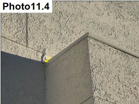
Proper metal caps are present at flat areas. Assess and reseal all metal cap terminations and transitions.
