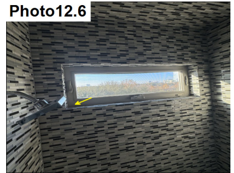
Interior shower window noted. Assess and reseat the interior of the window to minimize moisture intrusion.
