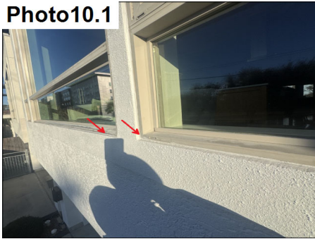
Sealant separation noted at windows in stucco and siding. Reseal all windows.
