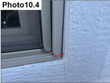
Sealant separation noted at windows in stucco and siding. Reseal all windows.
