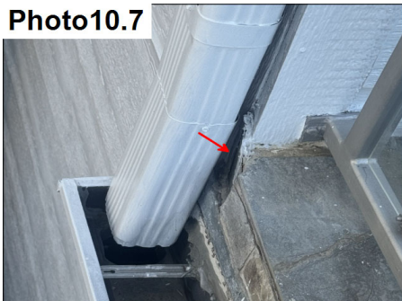
Sealant separation noted at balcony terminations. Reseal all balcony terminations.
