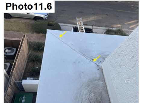
Proper metal caps are present at flat areas. Assess and reseal all metal cap terminations and transitions.
