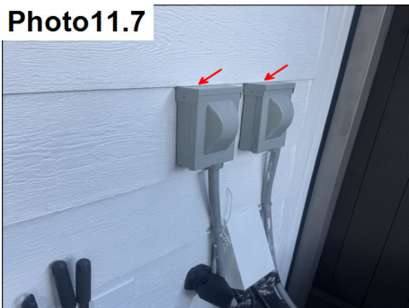
Some penetrations lack sealants. Seal all penetrations.
