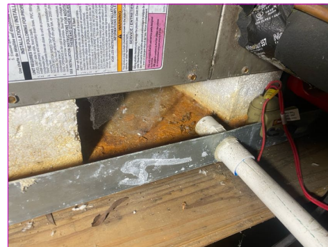
The attic-installed cooling system evaporator coil had a rusty condensate drain pan. This condition could result in moisture damage to attic or home interior materials.
