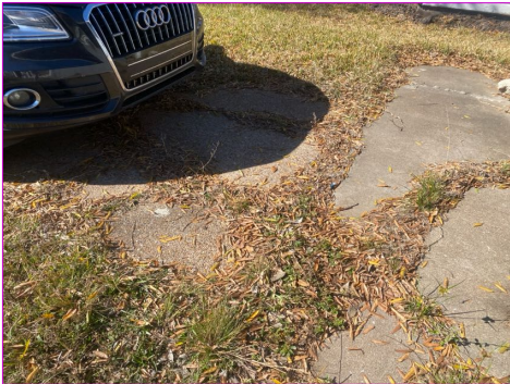
Significant cracks in the driveway should be filled with an appropriate material to avoid continued damage to the driveway.
