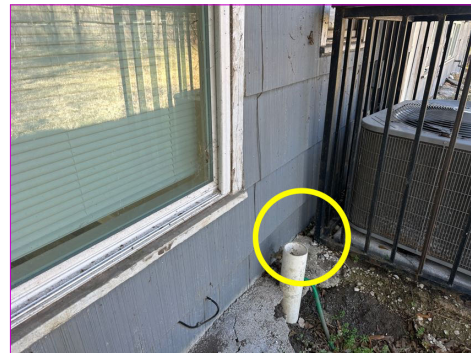
A clean out cover missing. The Inspector recommends repair by a qualified contractor.
