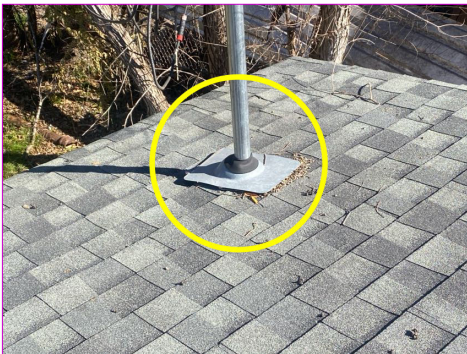
The electrical mast is loose on the roof. The inspector recommends that a qualified contractor evaluate and repair the condition.
