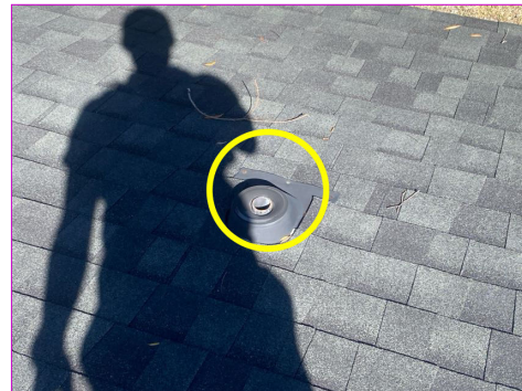
The plumbing vent was damaged. The inspector recommends that a qualified contractor evaluate and repair the condition.
