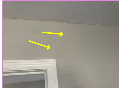
The walls exhibited settlement cracks. These cracks are commonly associated with normal foundation movement; however, the extent and cause could not be fully determined at the time of inspection. The inspector recommends a qualified contractor further evaluate and repair as needed.
