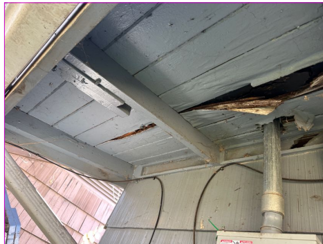
Soffits were old, severely deteriorated and sagging in some areas around the home. The Inspector recommends repair/replacement by a qualified contractor to prevent pests from entering the soffit space.
