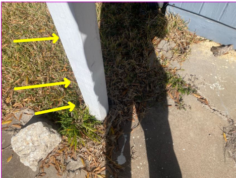
The exterior posts supporting the driveway overhang are not properly connected and/or are damaged. This condition may compromise the structural stability of the overhang. The inspector recommends that a qualified contractor evaluate and repair this condition as necessary.
