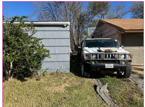
The inspector had limited access to inspect the right side of the house due to a vehicle parked extremely close to the exterior wall. As a result, portions of this area could not be fully evaluated at the time of inspection.
