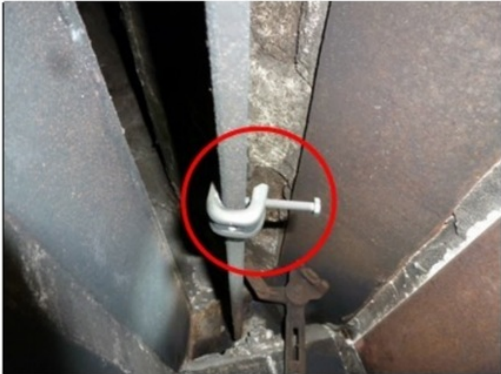
HEI file photo showing c-clamp in masonry fireplace
