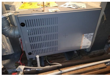
Heating Equipment - Functional:
