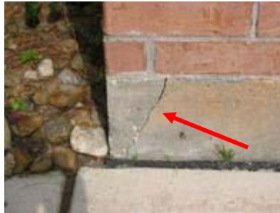
corner or wedge crack
