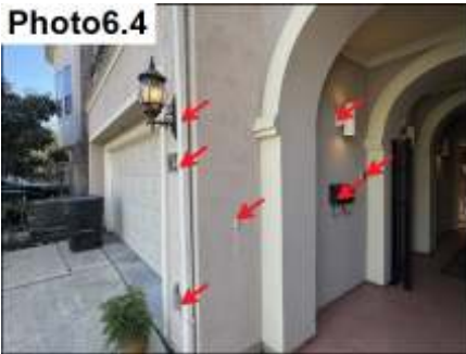
Penetration Sealants / Seal
