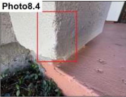
Impact Damage / Repair
