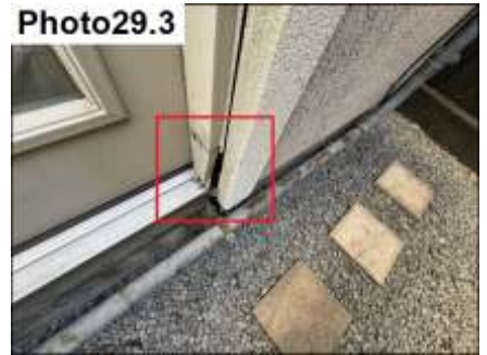
Wood Rot on Door Trim / Repair
