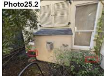
Wood Rot at Bottom Wall/ Repair
