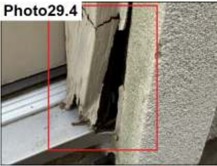
Wood Rot on Door Trim / Repair
