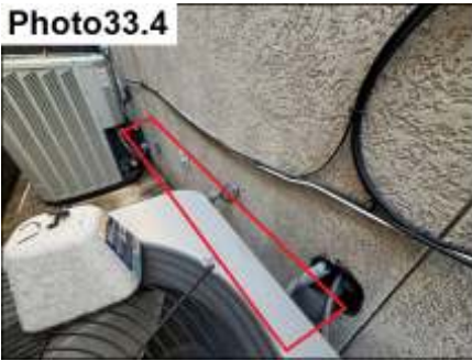
Substrate Damage / Assess & Repair
