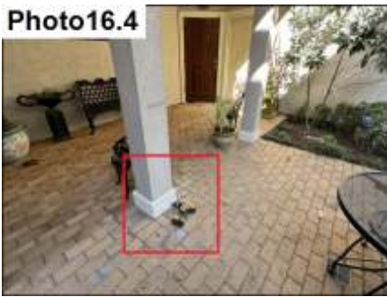
Substrate Damage / Assess & Repair
