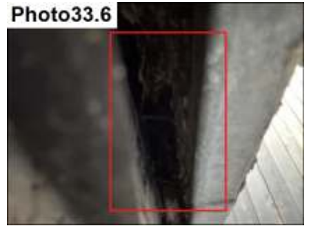
Substrate Damage / Assess & Repair
