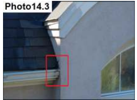
Kickout Flashing Failing/ Modify
