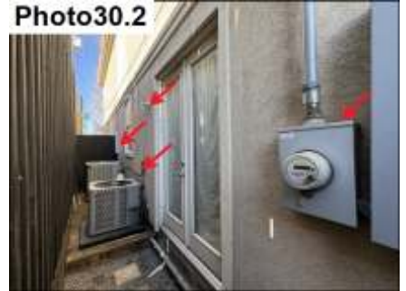
Penetration Sealants / Seal
