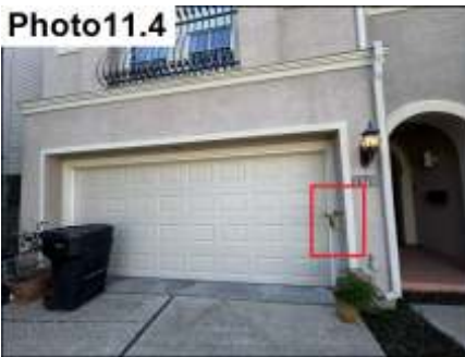
Substrate Damage / Assess, Repair and Install Proper Relief
