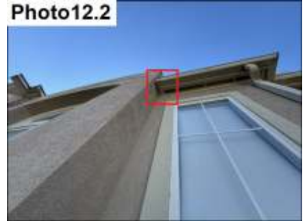
Wood Rot on Fascia / Repair
