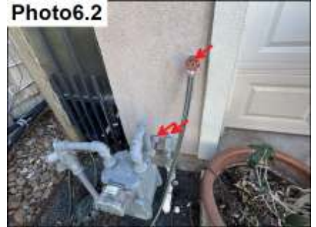
Penetration Sealants / Seal
