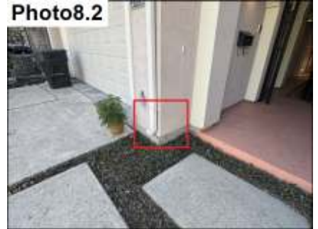
Impact Damage / Repair
