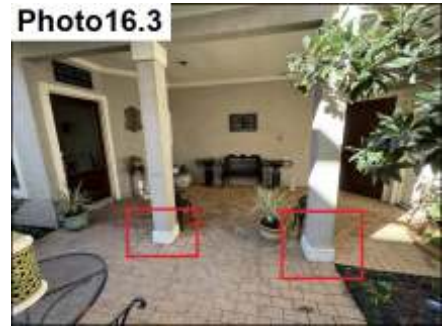
Substrate Damage / Assess & Repair
