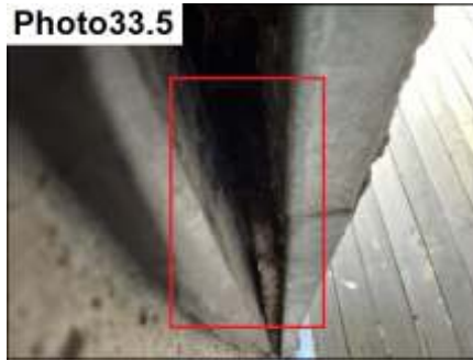
Substrate Damage / Assess & Repair
