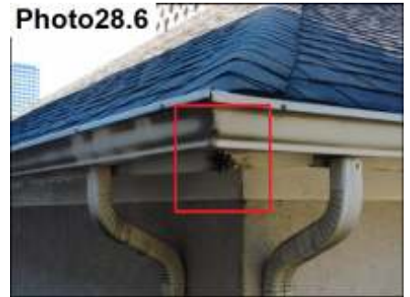
Wood Rot on Fascia / Repair
