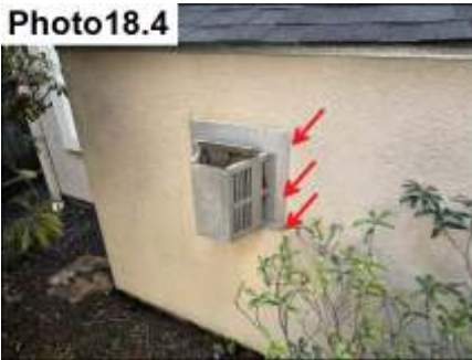
Penetration Sealants / Seal
