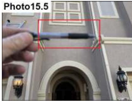
Cracks / Paint (Aesthetic)
