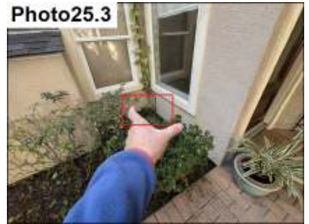
Wood Rot at Bottom Wall/ Repair
