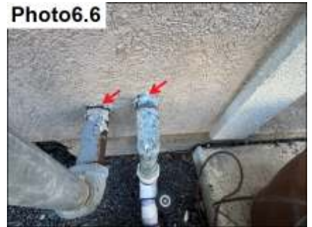
Penetration Sealants / Seal
