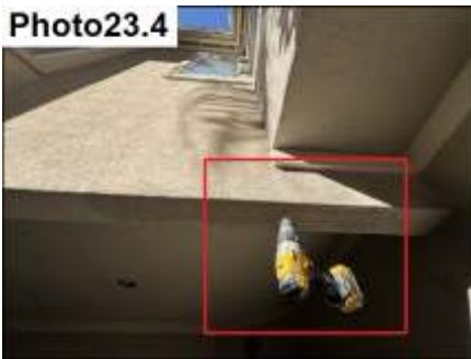
Photo23.4 Substrate Damage / Assess, Repair and Install Proper Relief
