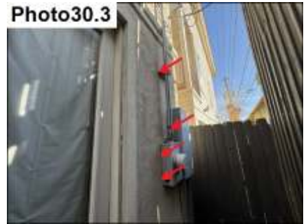
Penetration Sealants / Seal
