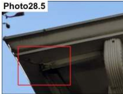
Wood Rot on Fascia / Repair
