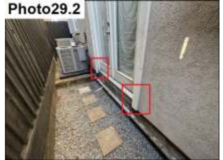
Wood Rot on Door Trim / Repair
