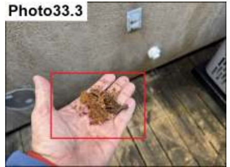
Substrate Damage / Assess & Repair
