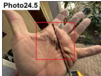
Photo24.5 Substrate Damage / Assess, Repair and Install Proper Relief
