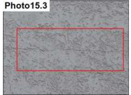
Cracks / Paint (Aesthetic)
