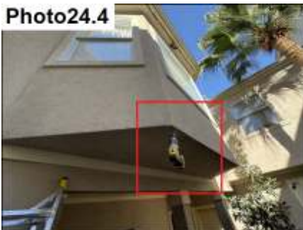
Photo24.4 Substrate Damage / Assess, Repair and Install Proper Relief
