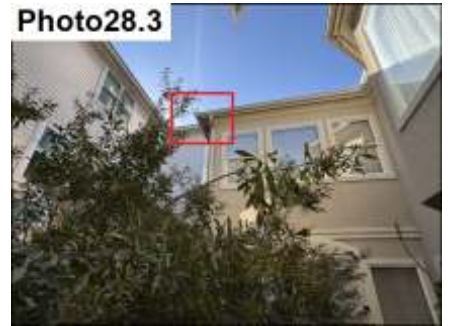
Wood Rot on Fascia / Repair
