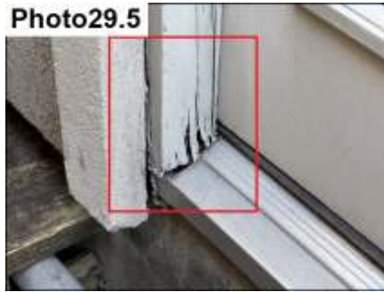
Wood Rot on Door Trim / Repair
