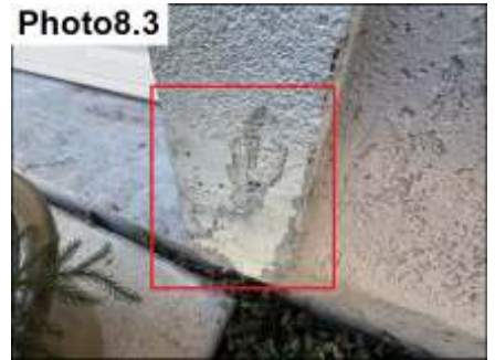
Impact Damage / Repair
