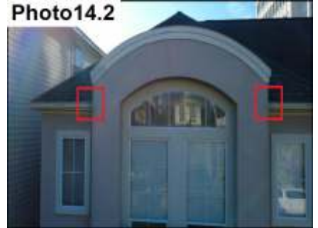
Kickout Flashing Failing/ Modify
