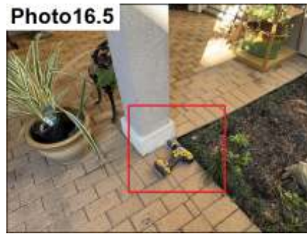
Substrate Damage / Assess & Repair
