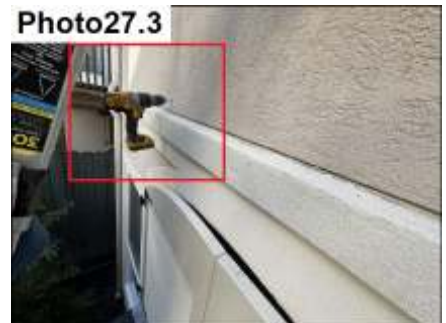
Substrate Damage / Assess & Repair
