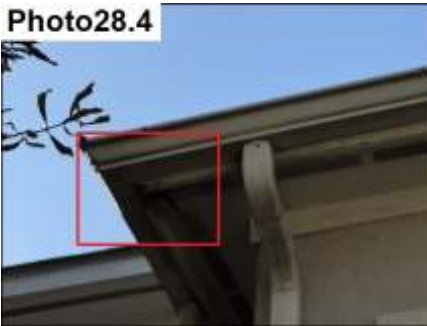
Wood Rot on Fascia / Repair
