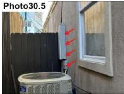
Penetration Sealants / Seal
