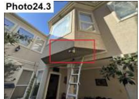
Photo24.3 Substrate Damage / Assess, Repair and Install Proper Relief
