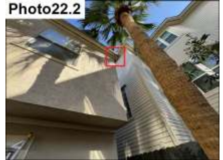
Wood Rot on Fascia / Repair
