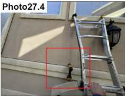
Substrate Damage / Assess & Repair
