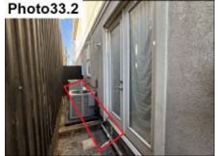
Substrate Damage / Assess & Repair
