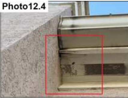
Wood Rot on Fascia / Repair
