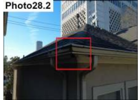
Wood Rot on Fascia / Repair
