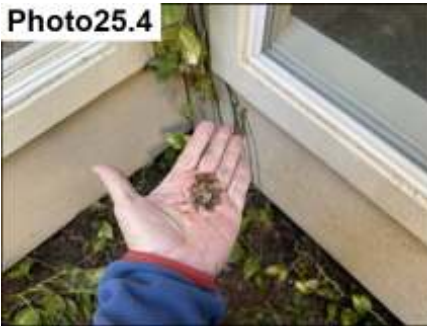
Wood Rot at Bottom Wall/ Repair
