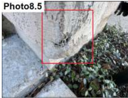
Impact Damage / Repair
